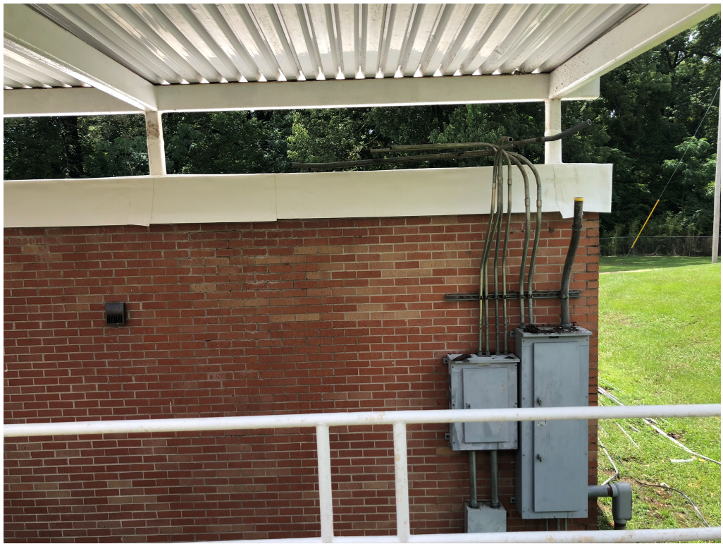
Figure 5 – Cut Power Conduit @ Building B
