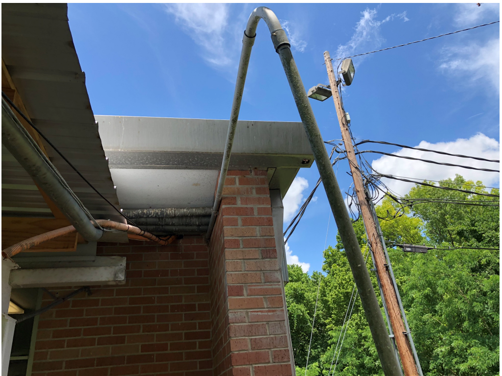
Figure 8 – Conduit inside of footprint of new ADA Ramp; should re route be overhead?
