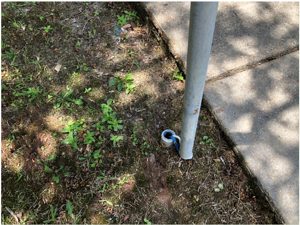
Figure 7 – Conduit inside of footprint of new ADA Ramp; should re route be overhead?
