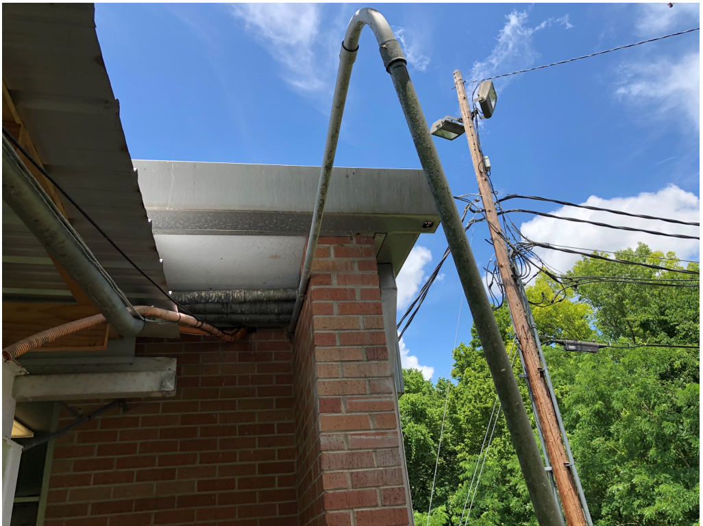
Figure 8 – Conduit inside of footprint of new ADA Ramp; should re route be overhead?
