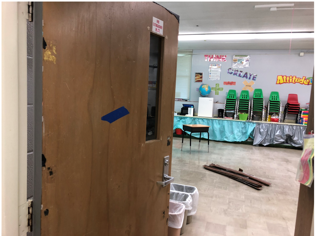
Figure 6 – Blue Tape on door to indicate No Paint in Room (typical in 300 wing)
