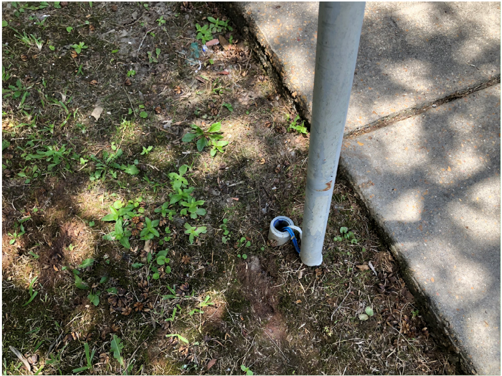
Figure 7 – Conduit inside of footprint of new ADA Ramp; should re route be overhead?
