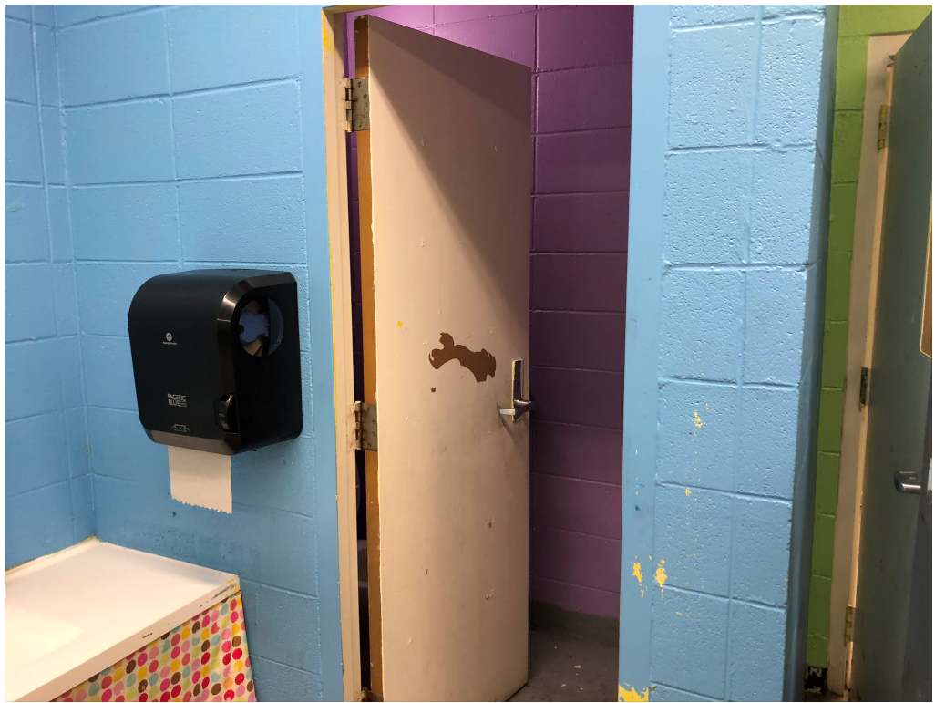
Figure 5 – Doors in Rooms Requested to Forego Painting Show Much Damage
