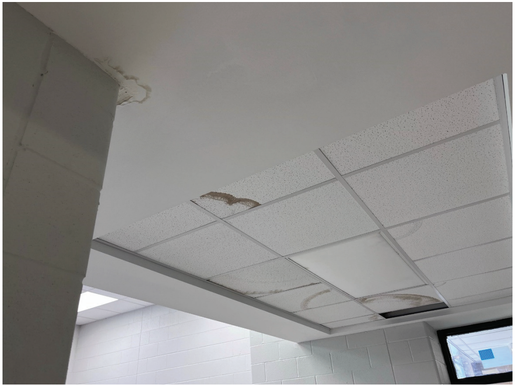
Figure 3 – Leak at E end of Addition
