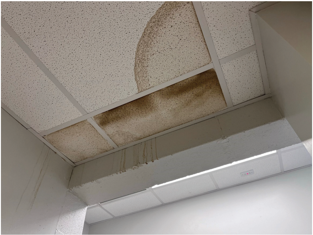
Figure 1 – Leak at W end of Addition
