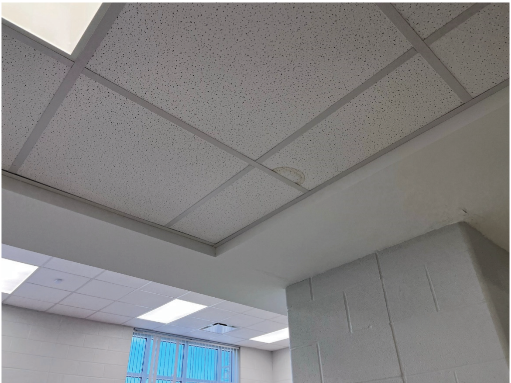
Figure 2 – Leak at E end of Addition
