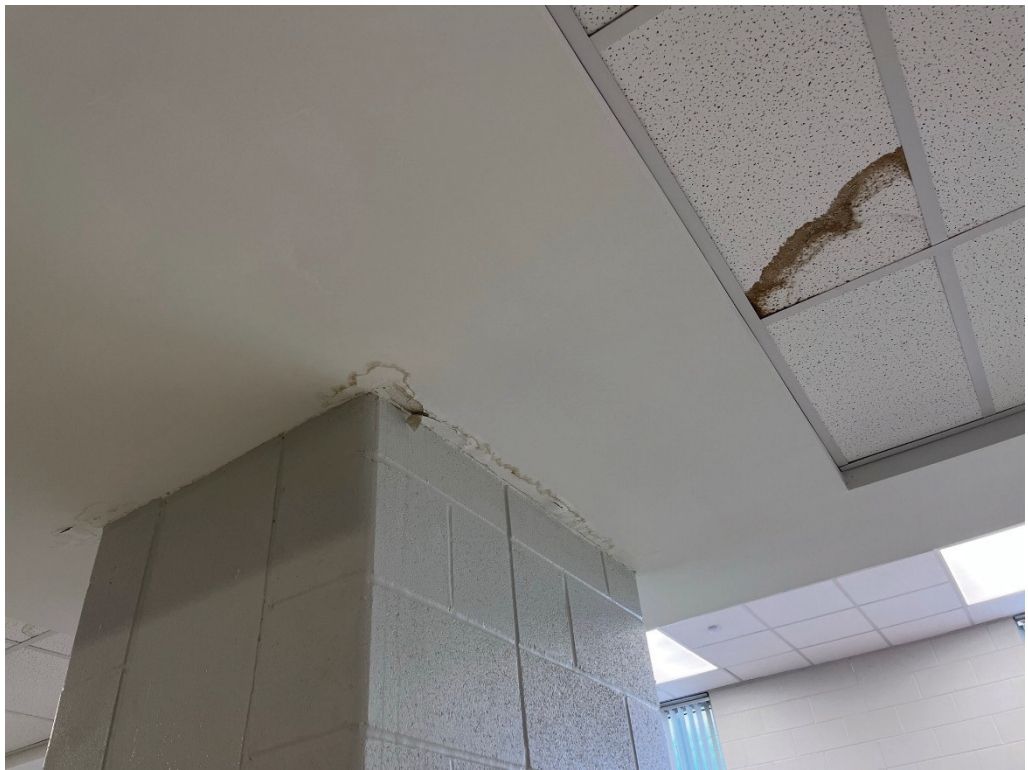
Figure 4 – Leak at E end of Addition
