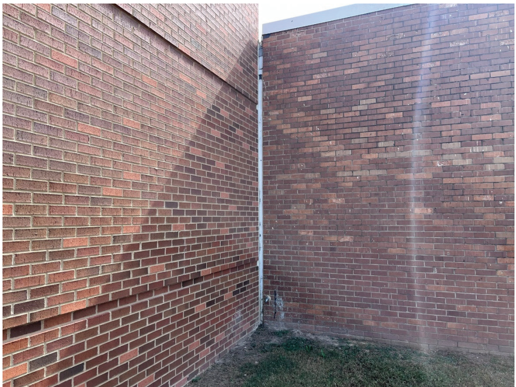
Figure 12 – Missing Expansion Cover
