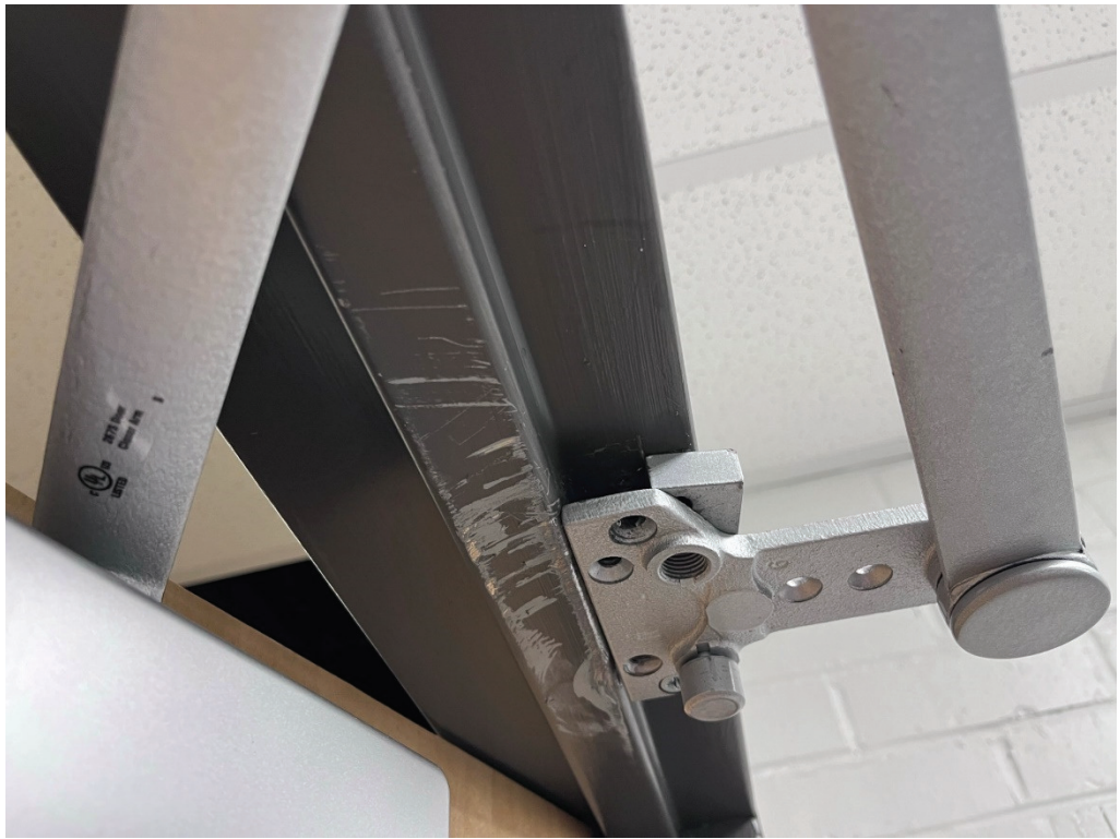
Figure 7 – No Predrilled hole is apparent
