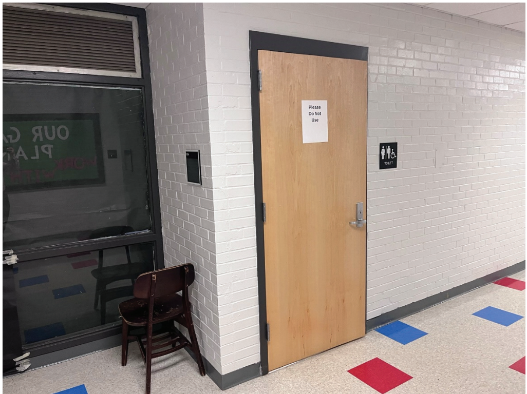
Figure 6 – Door with door closer not installed completely
