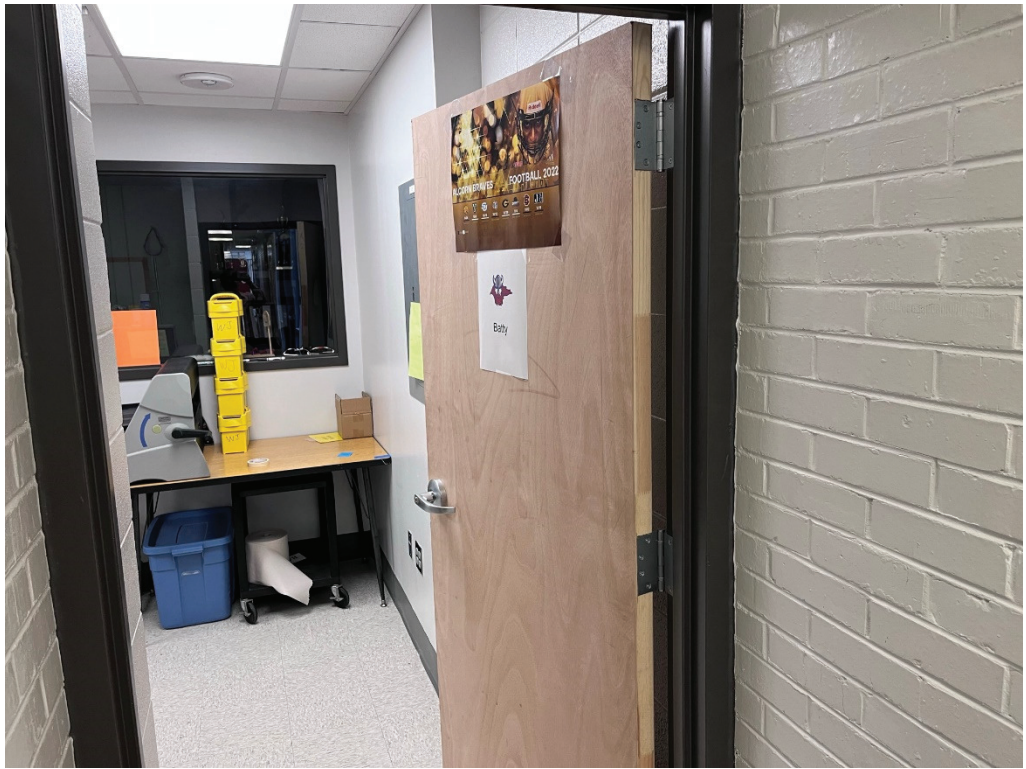
Figure 5 – Door Installed with Bare Wood
