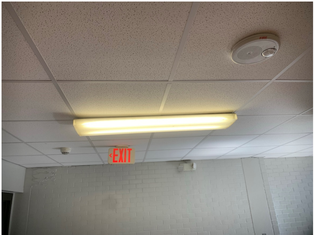
Figure 14 – Light crooked at end of E-226
