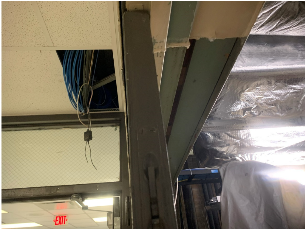
Figure 17 – Hardware has been painted, making it inoperable; return to working order
