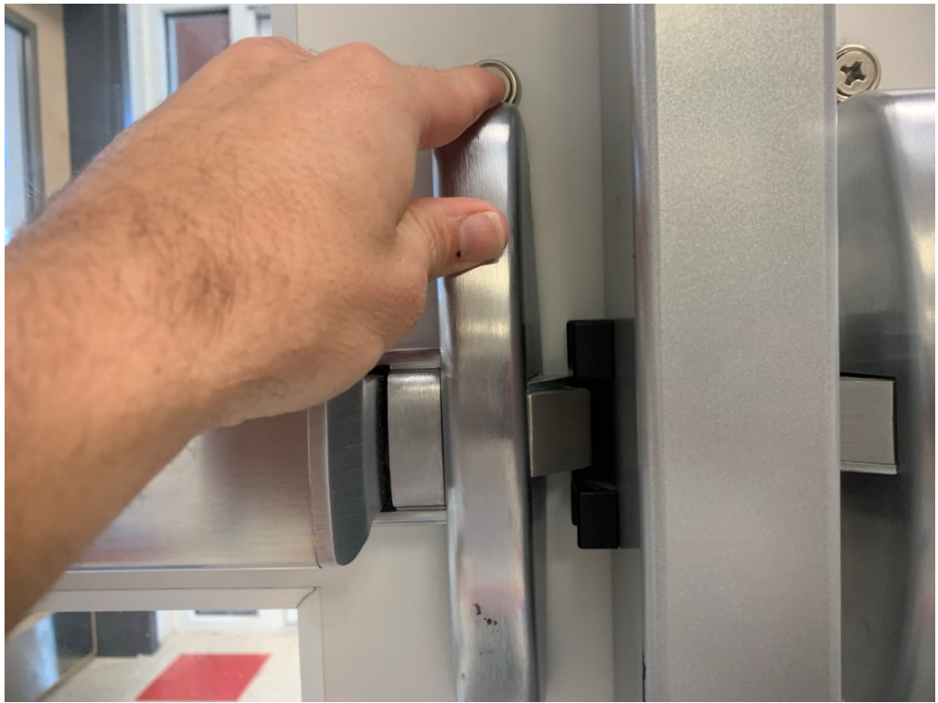
Figure 23 – Secondary latch not engaged @ catch; adjust catch to receive both parts of latch
