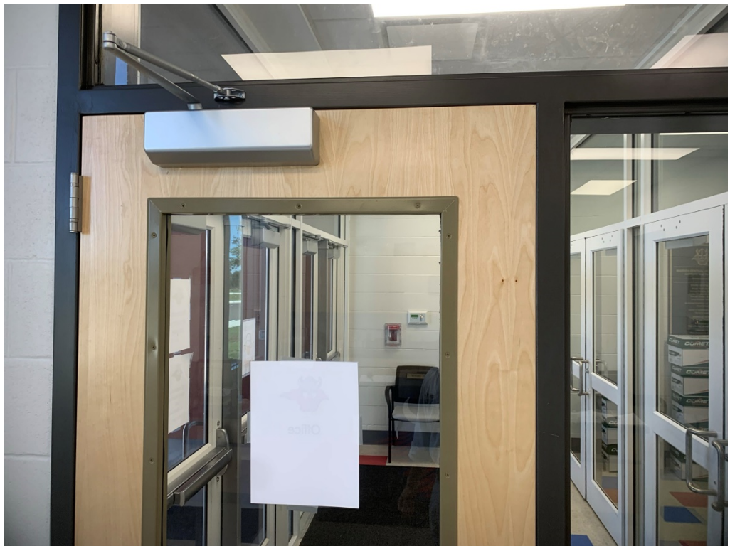
Figure 2 – Door needs adjustment; it's crooked in frame and drags at the top
