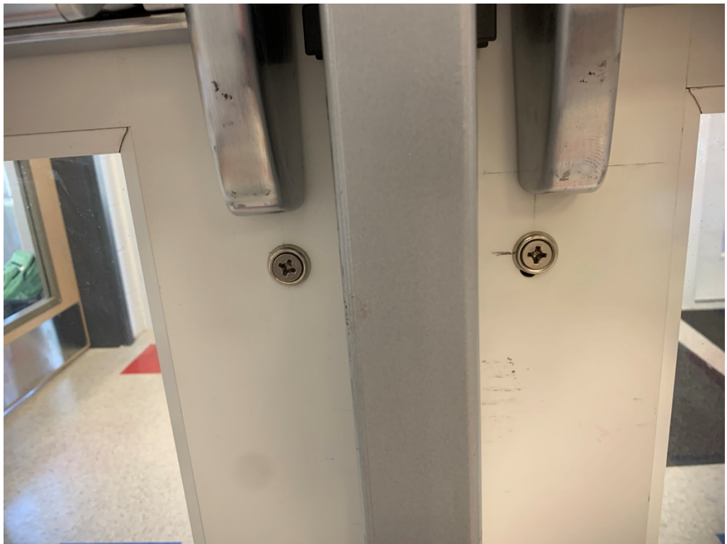
Figure 22 – Construction marks still present at storefront; remove
