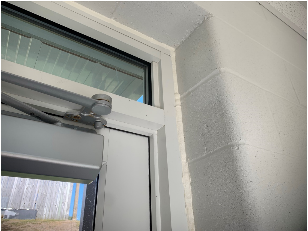
Figure 16 – Caulking still lumpy at new; smooth
