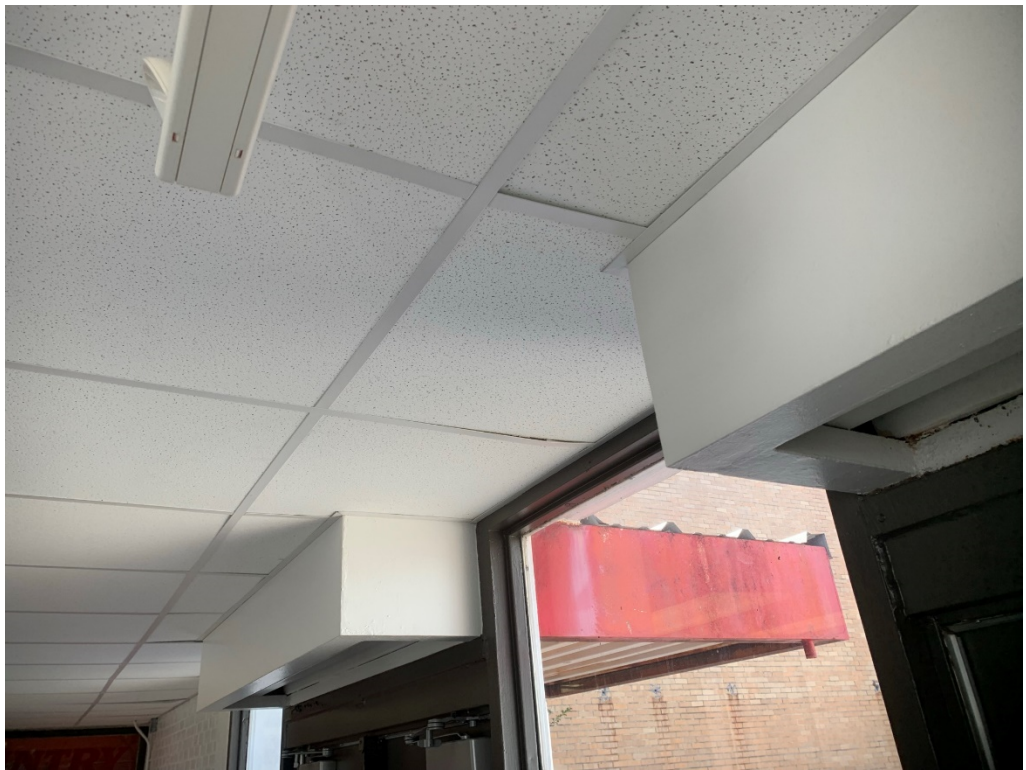
Figure 10 – Ceiling is still sagging at south end of E-220
