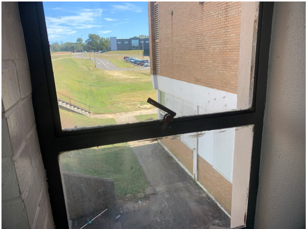
Figure 8 – Paint at window glazing to be removed
