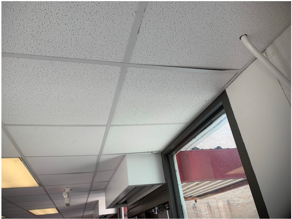
Figure 11 – Ceiling is still sagging at south end of E-220
