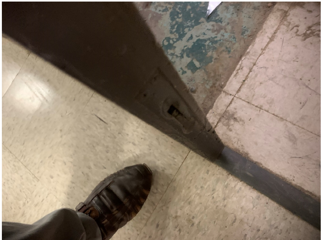
Figure 18 – Hardware has been painted, making it inoperable; return to working order
