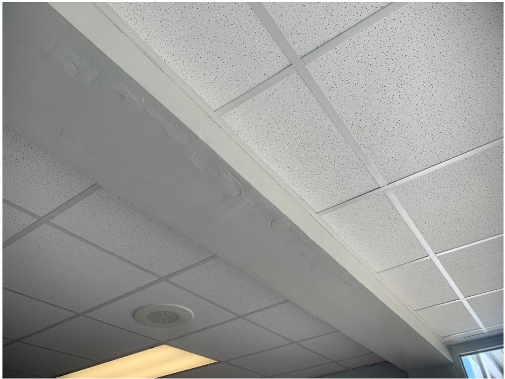
Figure 7 – Mottled finish at south end of E-320 to be smoothed and repainted
