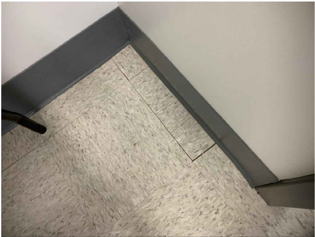
Figure 6 – Tile to be resecured in place at A-305
