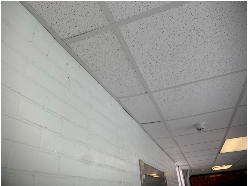
Figure 9 – Ceiling is still sagging at south end of E-220
