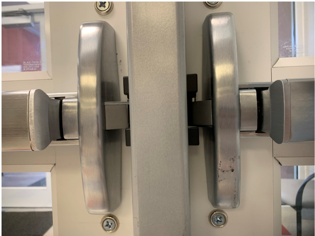
Figure 24 – Secondary latch not engaged @ catch; adjust catch to receive both parts of latch
