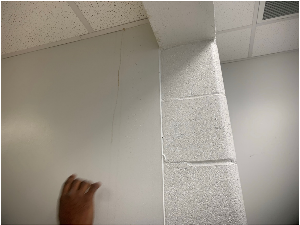
Figure 5 – Roof leak still present at A-305
