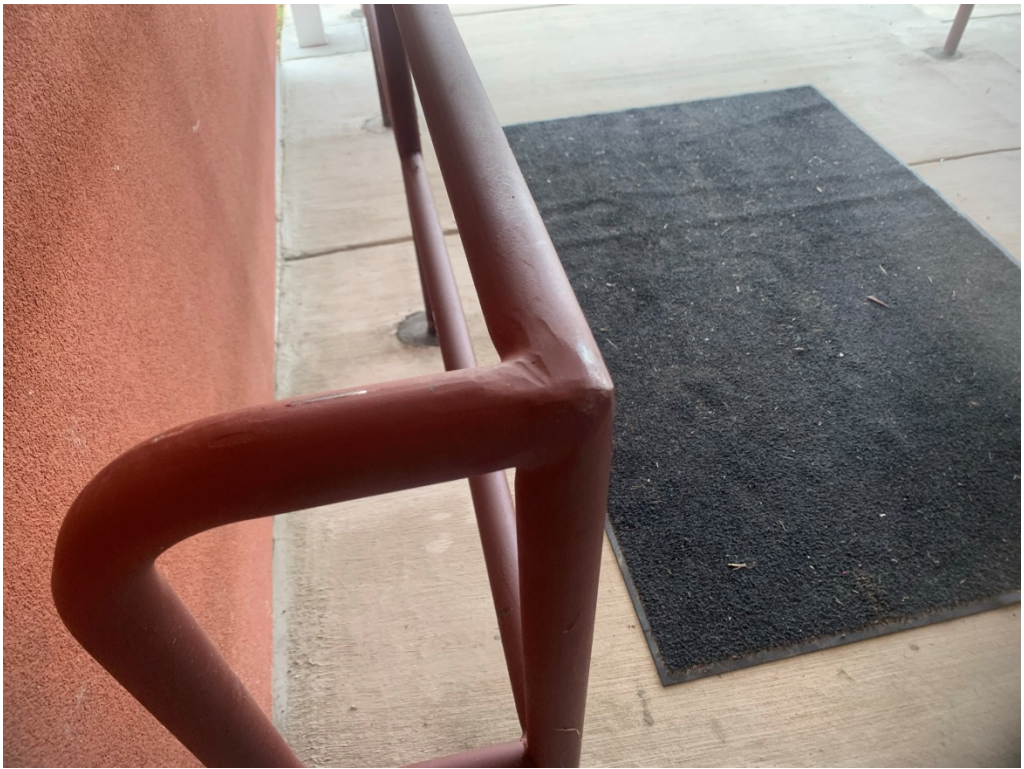
Figure 3 – Field repairs needed at handrails
