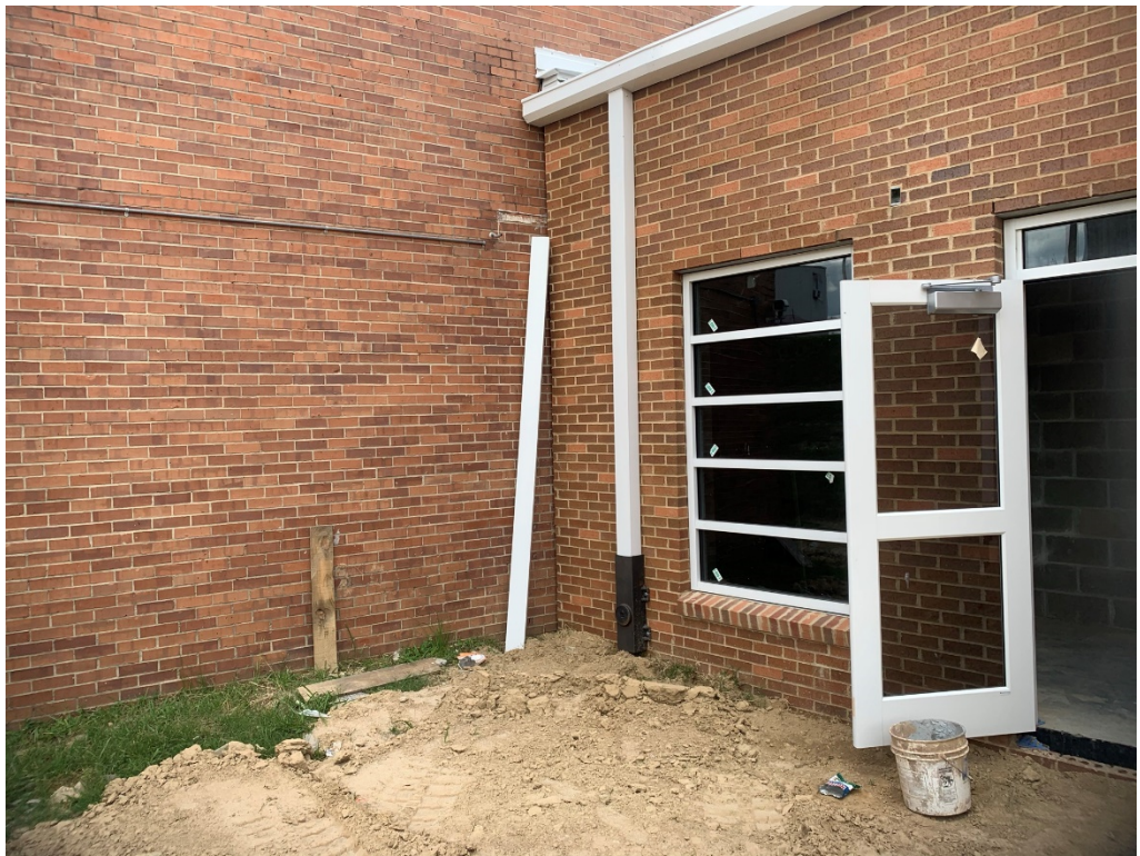
Figure 8 – Gutters Tied into Drainage at North Façade of Corridor at 2 nd Floor
