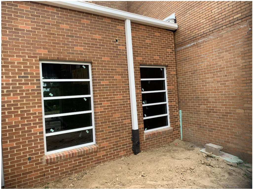
Figure 7 – Gutters Tied into Drainage at North Façade of Corridor at 2 nd Floor
