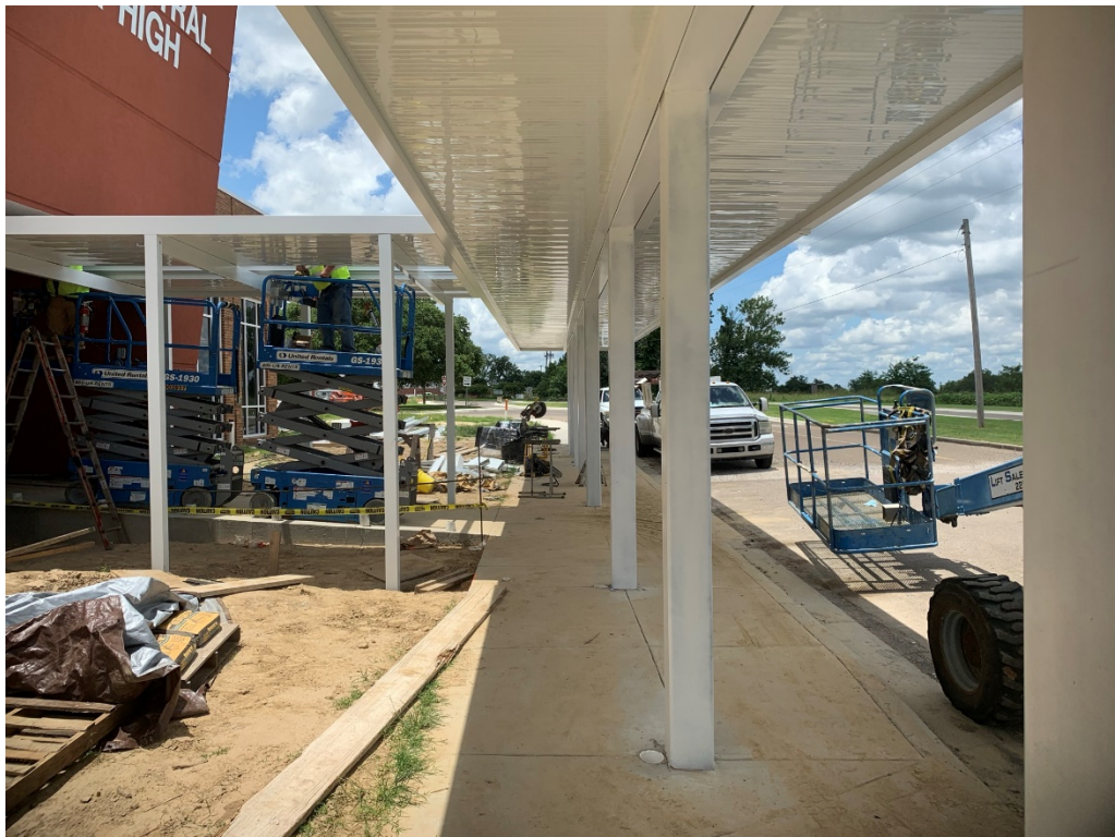
Figure 2 – Awning Installation; paint at steel work is ongoing and requires more coverage
