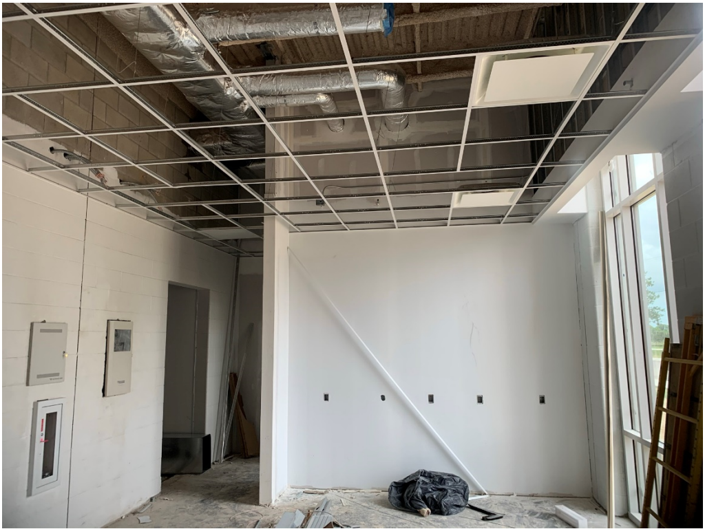
Figure 3 – Admin Area with Grid Installed
