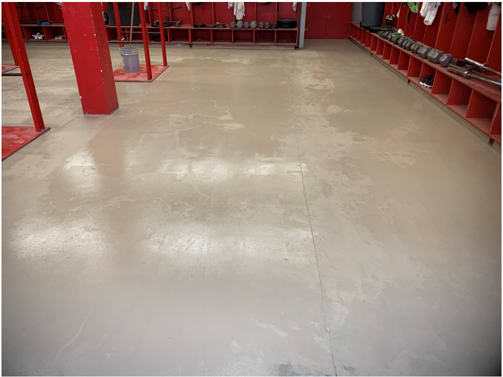
Figure 7 – Floor Paint at Field House
