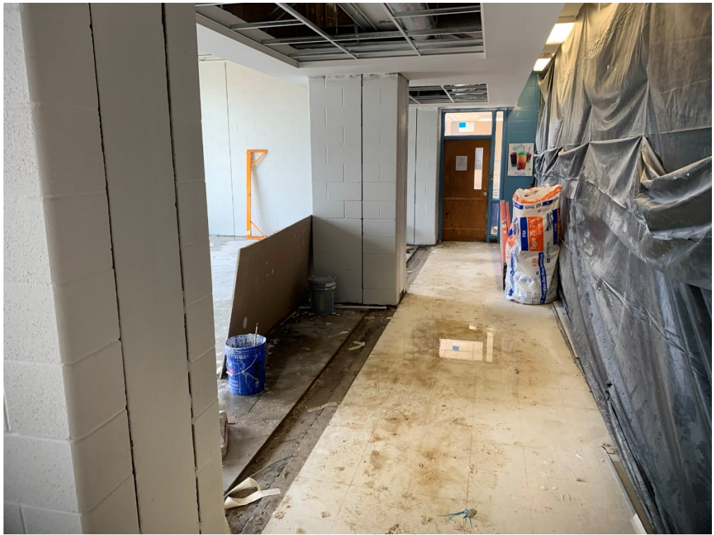
Figure 5 – Water Noted in cafeteria extension due to roof unfinished roof flashing
