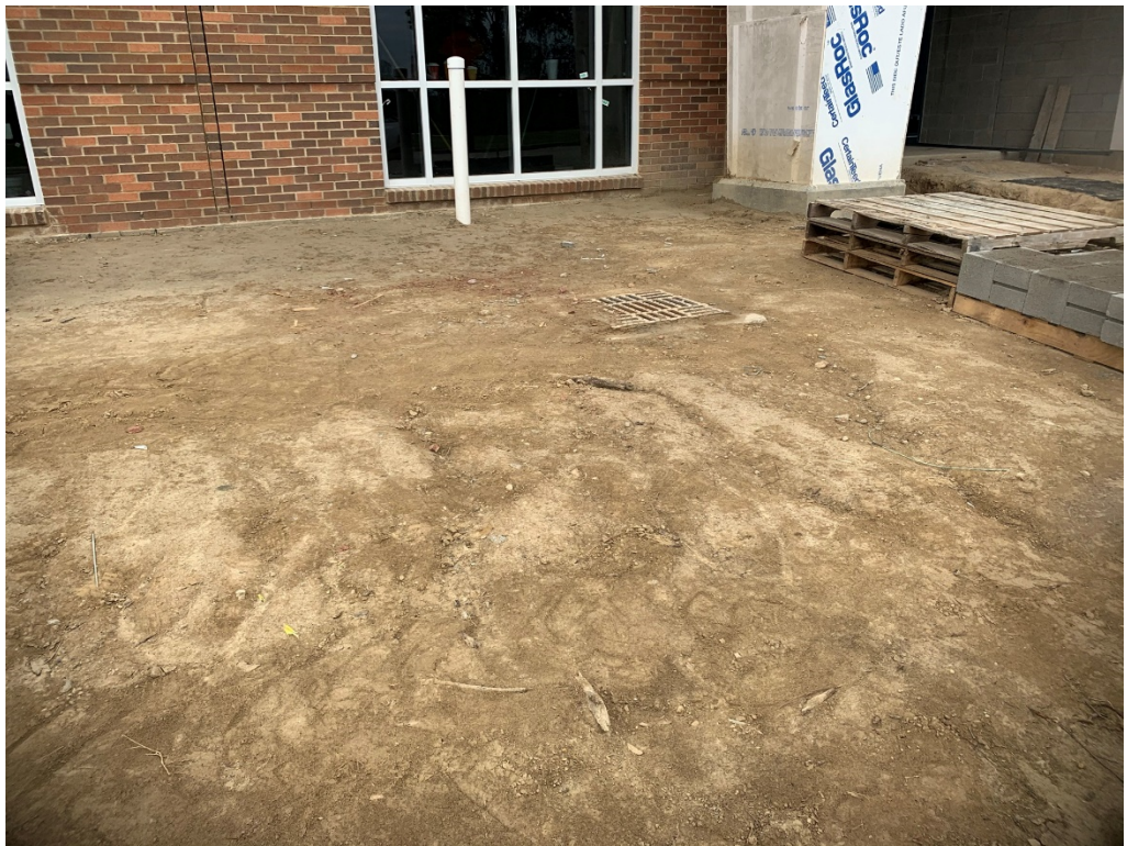
Figure 8 – Is this inlet too high? it does not appear to have a collection area
