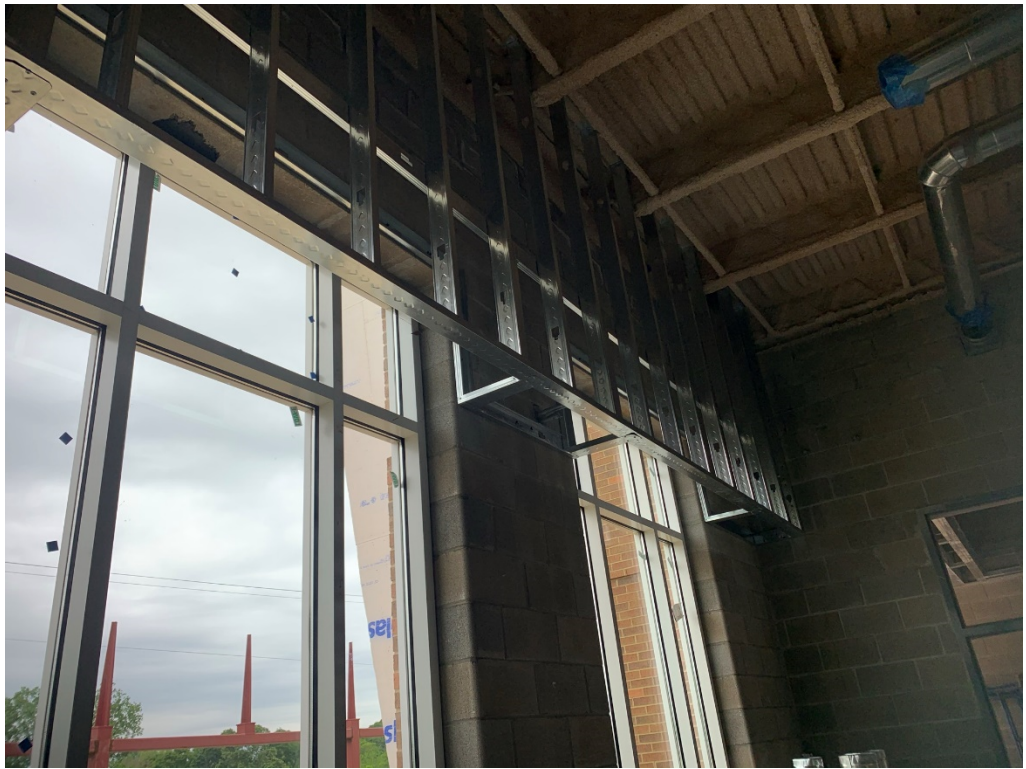
Figure 5 – Admin Area; furr down
