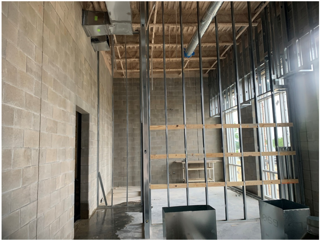
Figure 3 – Admin Area Framing (water from recently cut opening for ducting; to be sealed)
