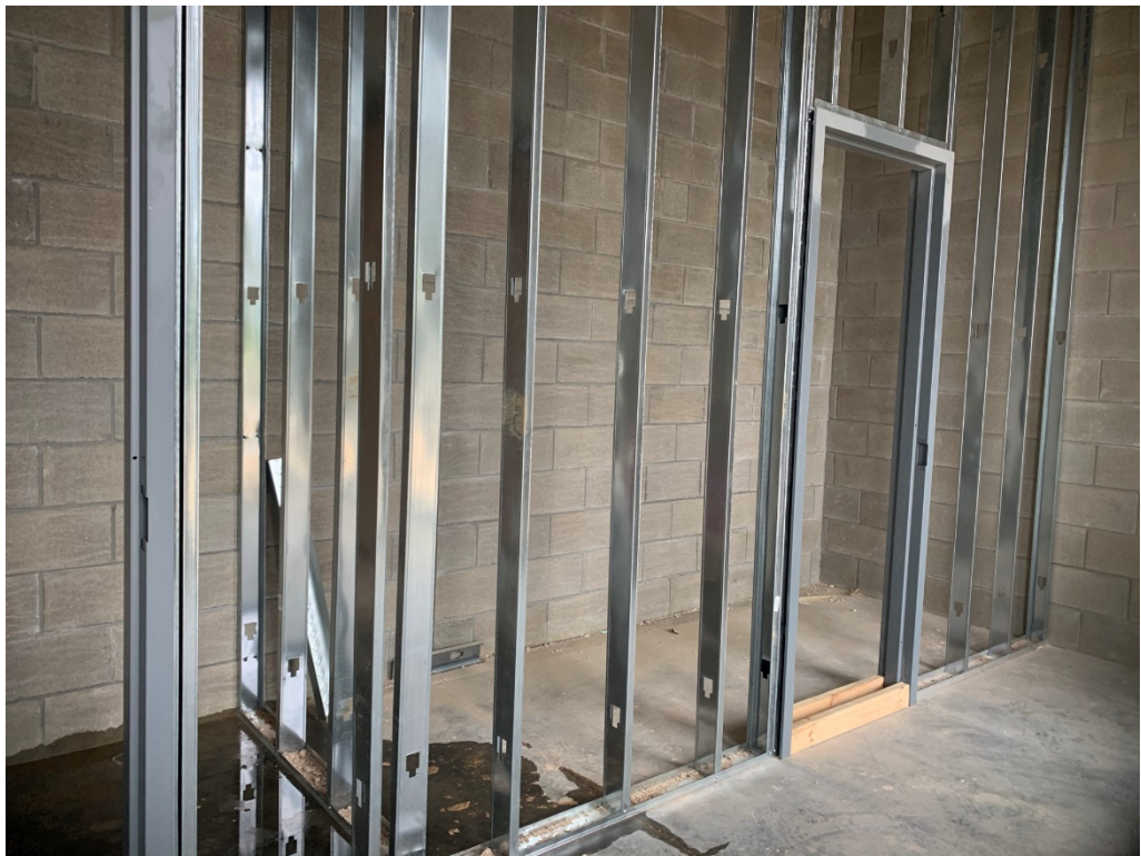
Figure 4 – Admin Area Framing (water from recently cut opening for ducting; to be sealed)
