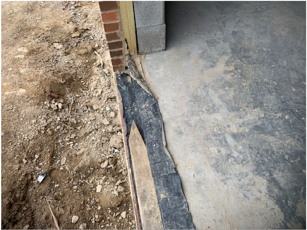
Figure 3 – Asphalt Flashing will require repair/replacement
