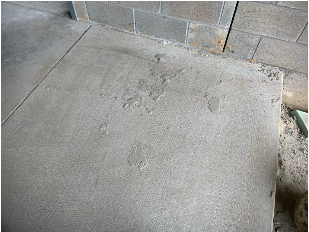
Figure 7 – Mortar Spills on New Concrete
