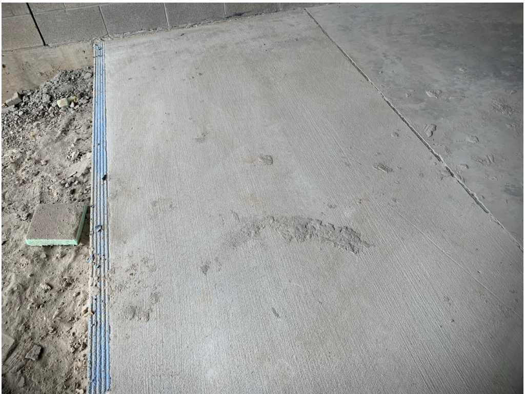
Figure 8 – Mortar Spills on New Concrete
