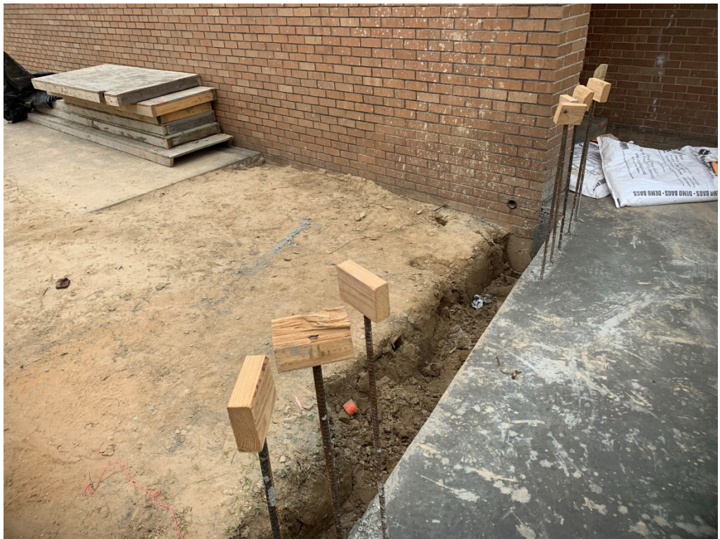
Figure 14 – Difference Between New Slab & Sidewalk appears to require at least 36' of ramp to maintain 1:12 slope min but preferably should be 1:20 (60')
