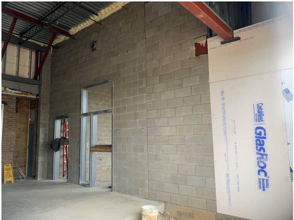
Figure 6 – New CMU Interior Wall with Frames; there should be no foam at this rated wall
