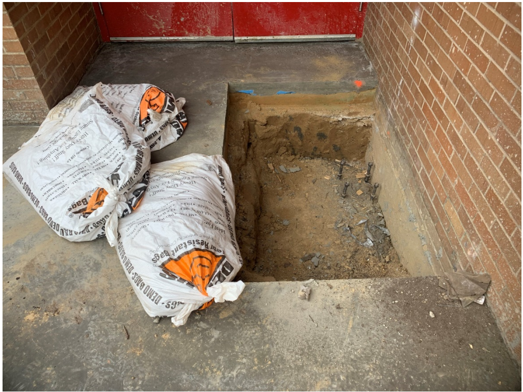
Figure 13 – Inadequate Protection at Excavation
