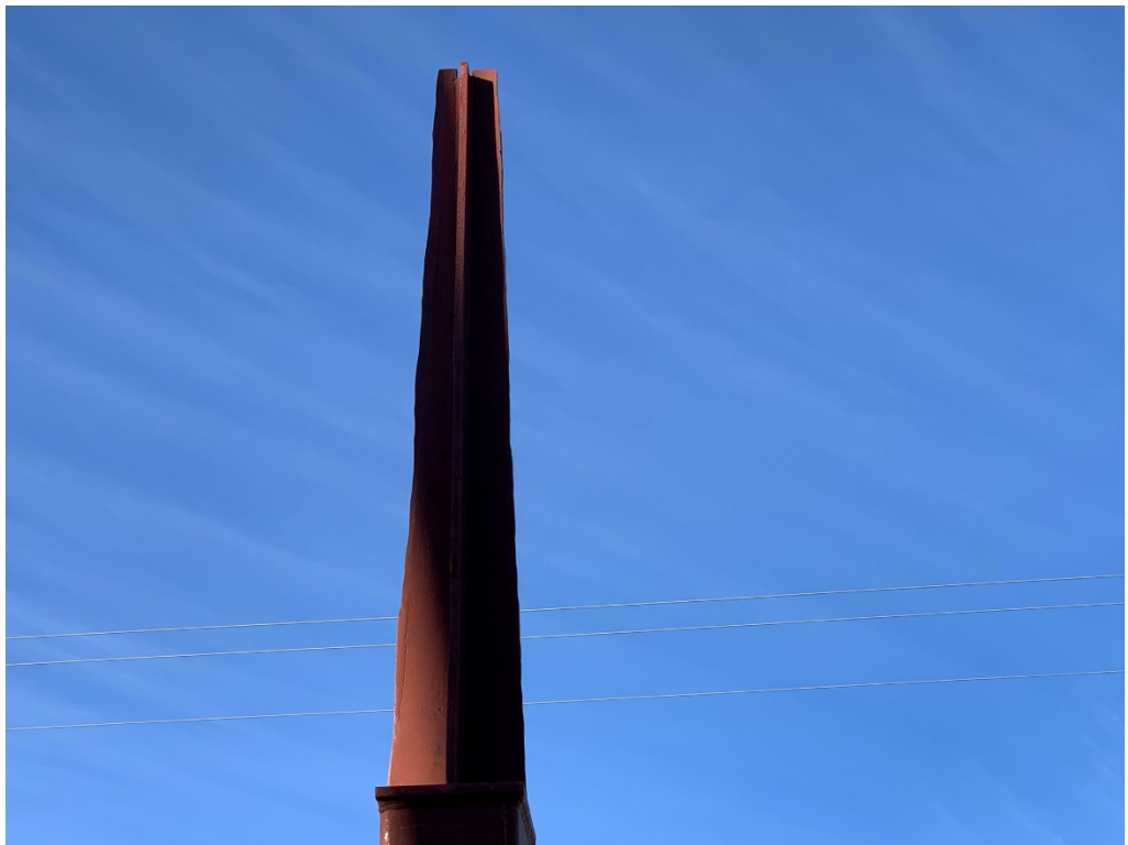
Figure 2 – Steel Spires need to Be Replaced with New spires that are cut Straight
