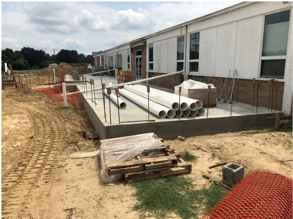
Figure 4 – PVC Stored on Site
