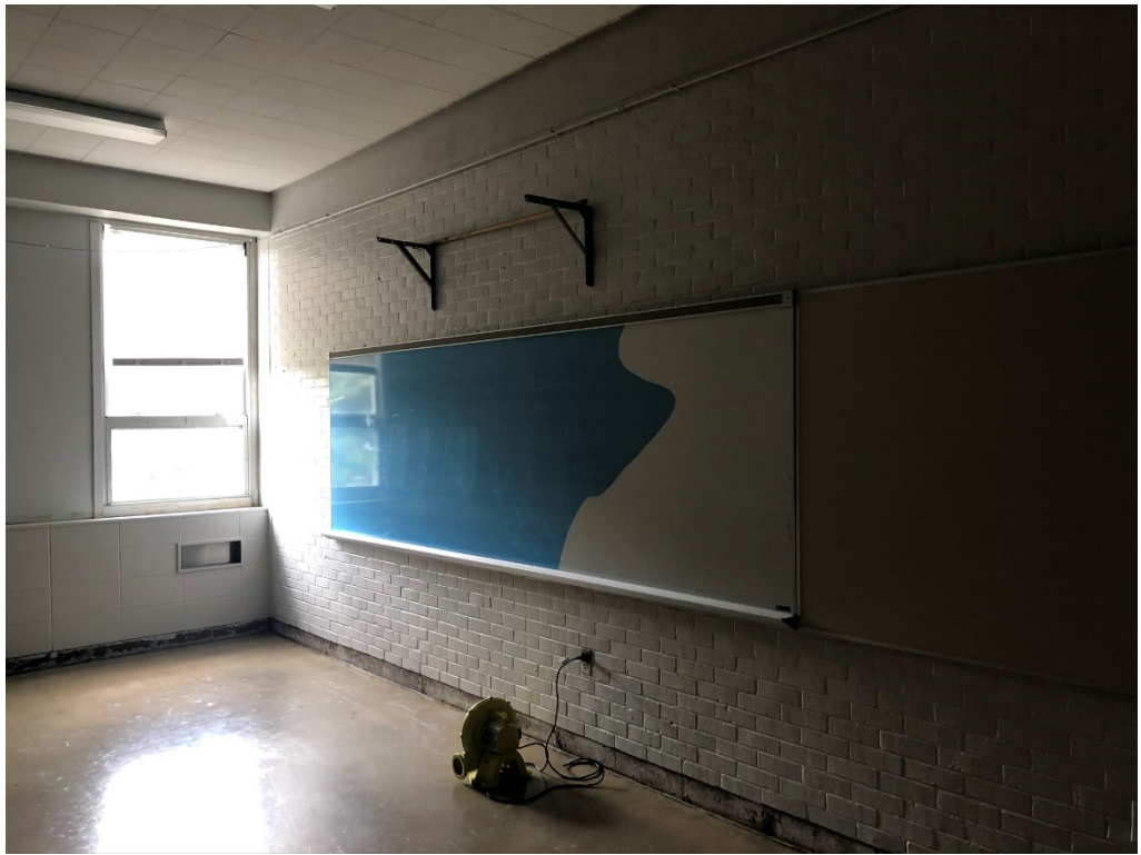
Figure 1 – Display Board Installed
