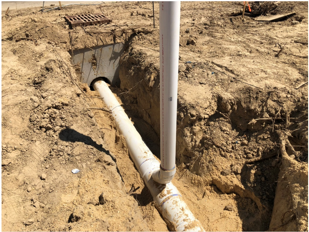
Figure 3 – Sewer discharge to Street
