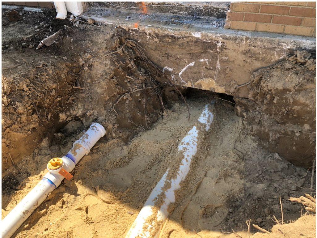
Figure 2 – Sewer leaving main building
