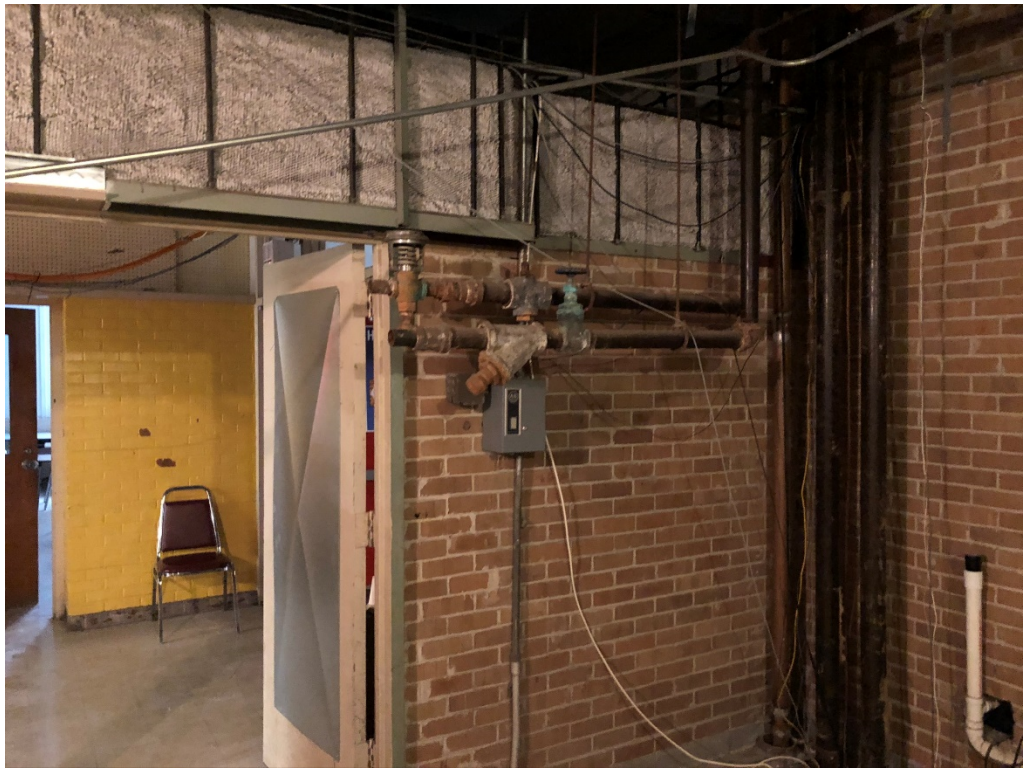
Figure 5 – Similar Condition on 2 nd Floor Mechanical Room Exists as in E-322
