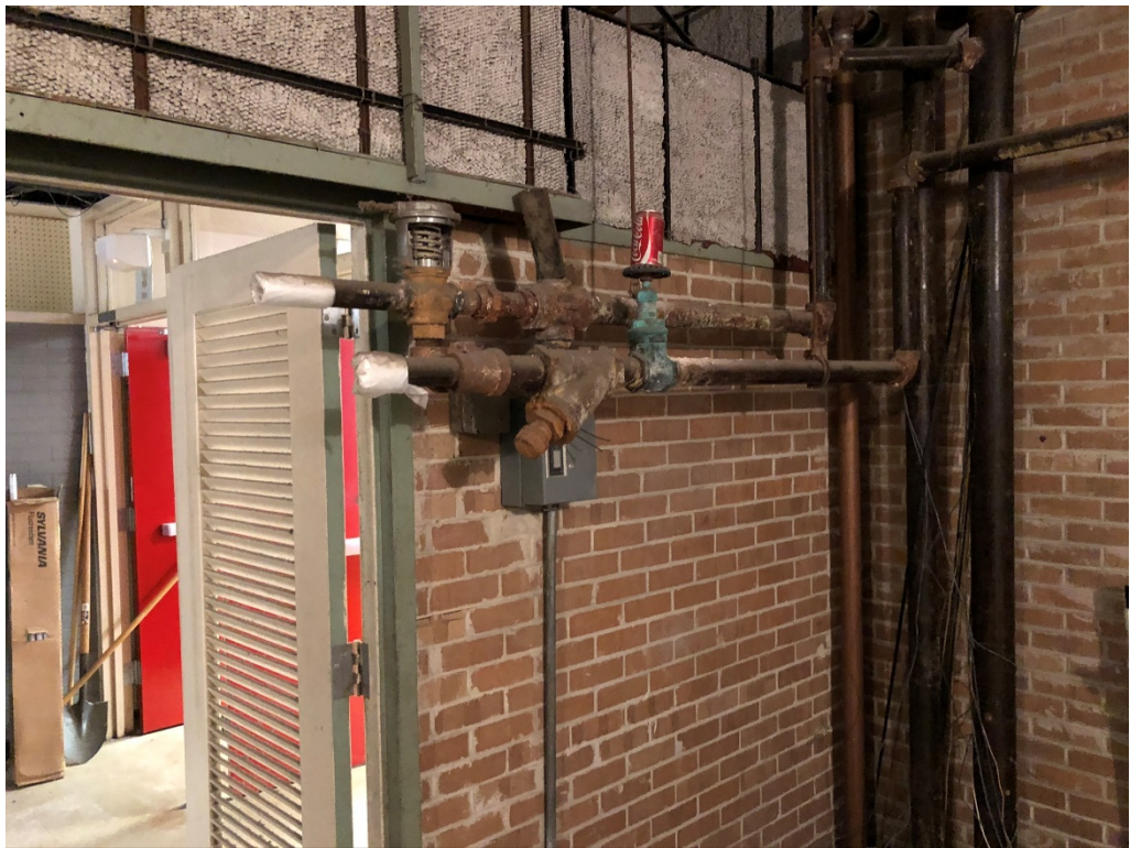
Figure 4 – E-322; existing hazard at door to be used for entry to Janitor's closet
