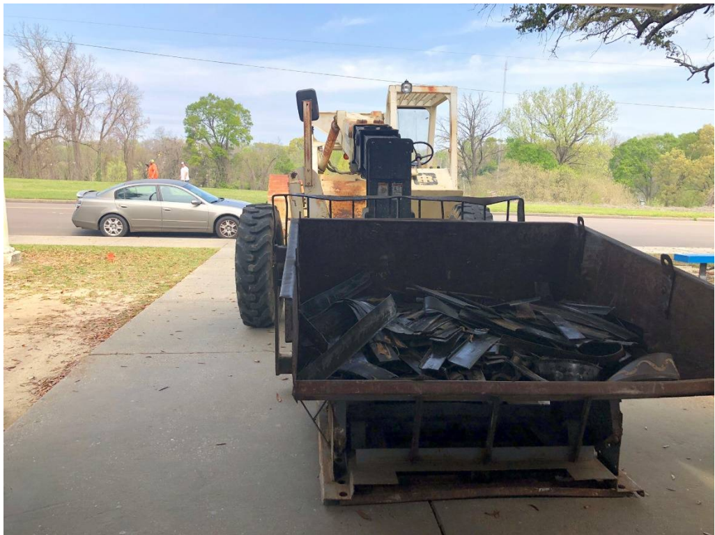
Figure 4 – Methods for Removing Debris from Front Door
