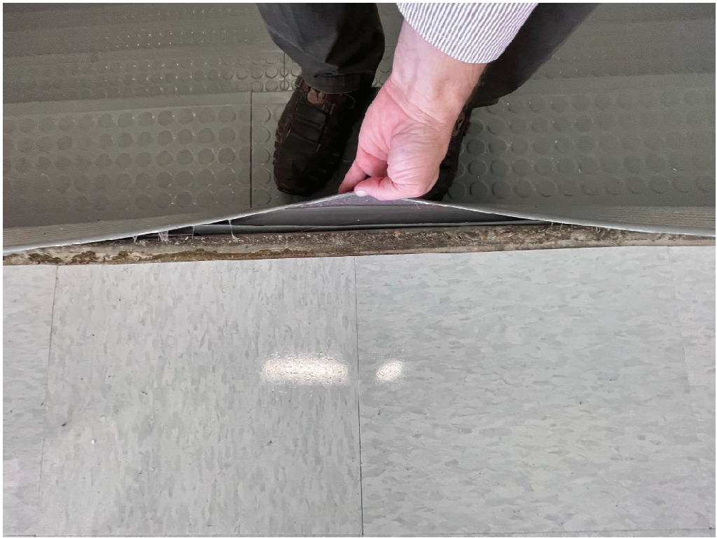
Figure 3 – Rubber Nosing poorly adhered
