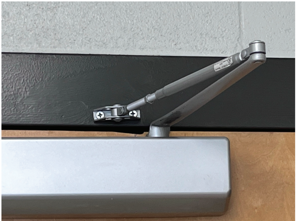
Figure 2 – Closer Rubs Top of Door
