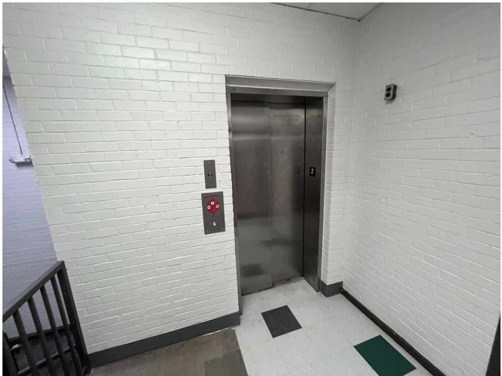
Figure 8 – Elevator has Not worked for Months
