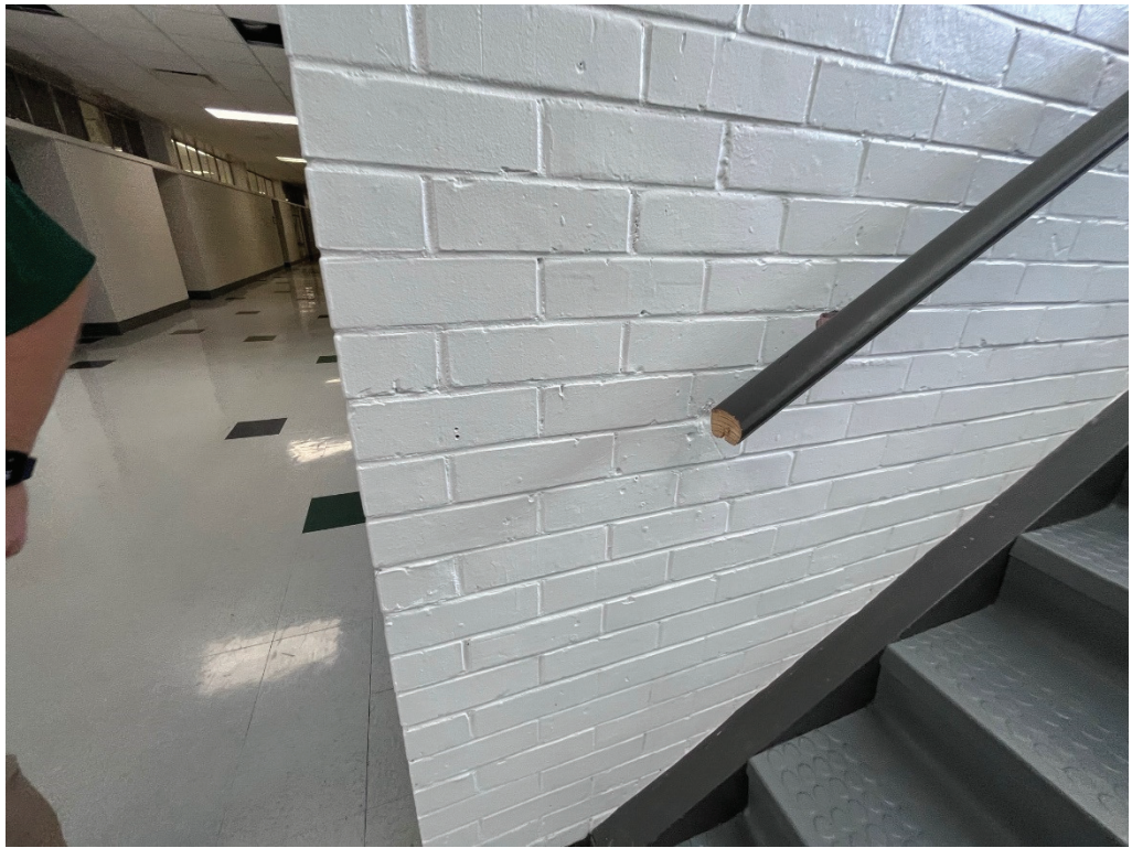
Figure 5 – Handrail Extension not Substantial; needs to be replaced
