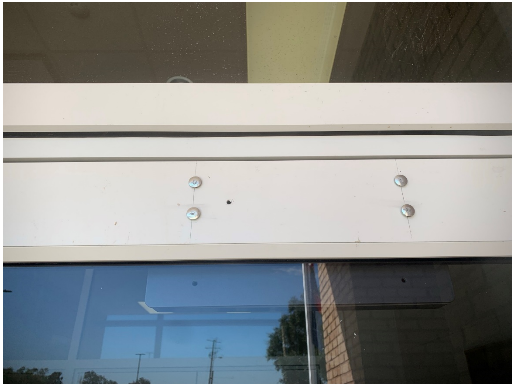
Figure 7 – Construction marks still present at New Doors; fill mis-drilled hole
