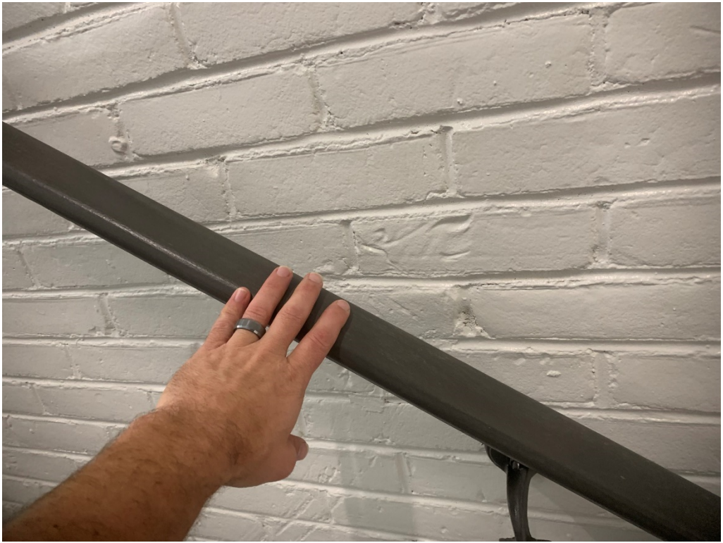
Figure 23 – Handrail is rough in some areas and needs to be sanded and repainted
