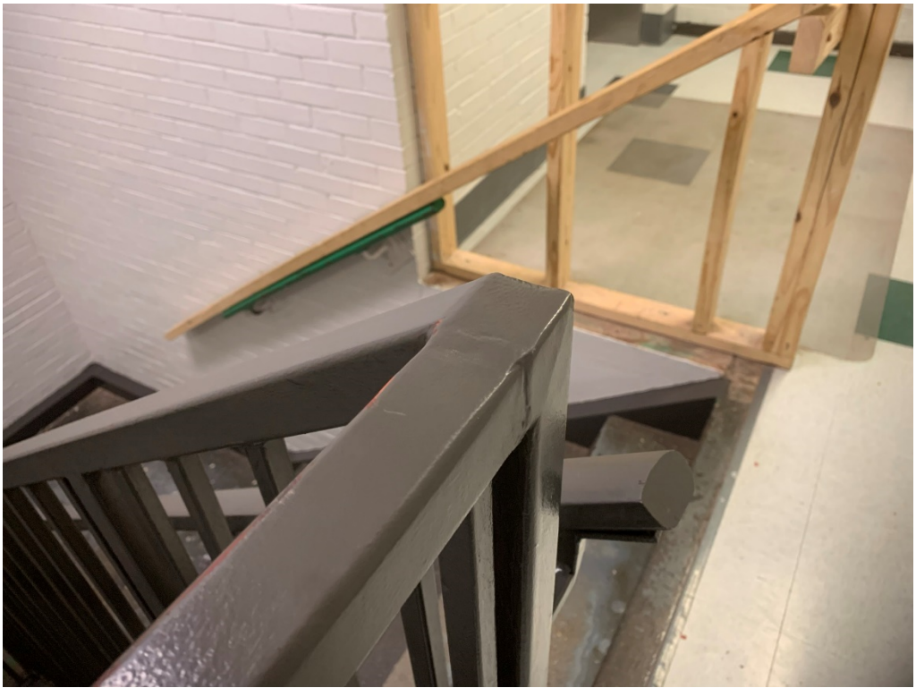
Figure 37 – Guardrails need repair for smooth appearance
