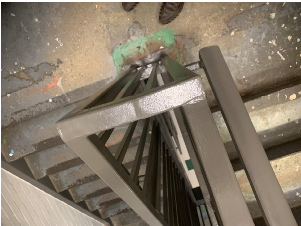
Figure 38 – Guardrails need repair for smooth appearance
