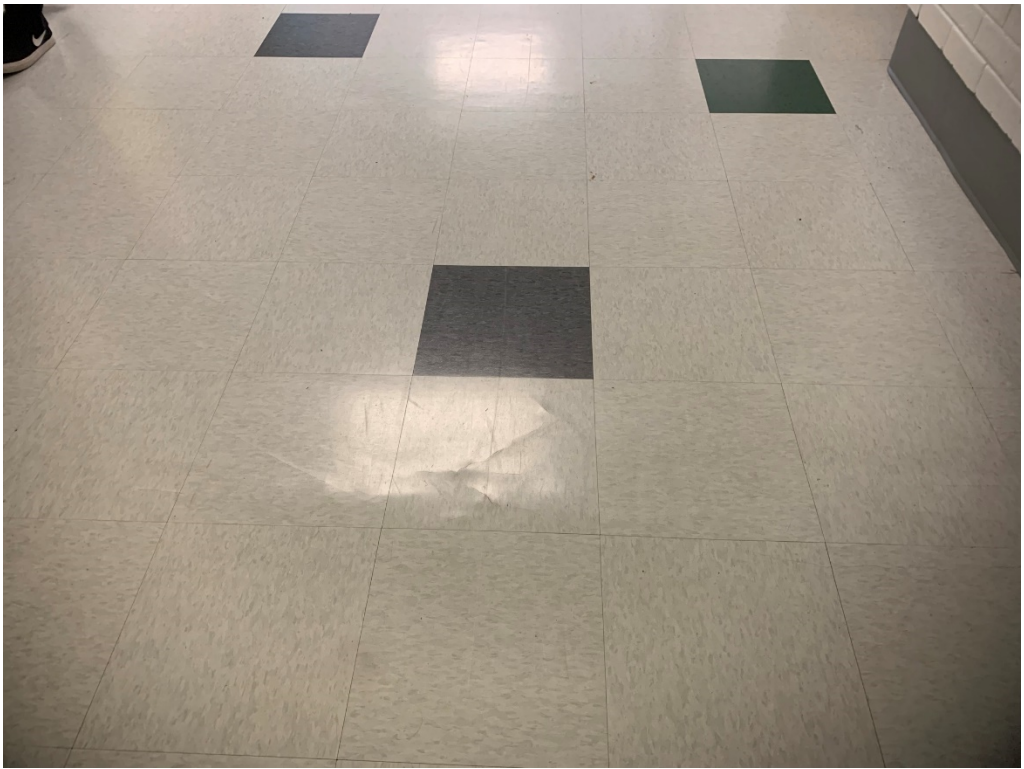
Figure 43 – Floor tile at E-216 near E-212 transmitting through poorly prepped subfloor; replace and prep correctly
