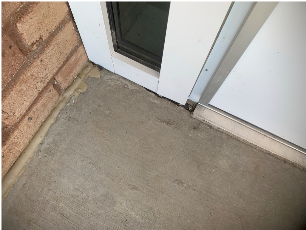
Figure 10 – Fill in gaps between concrete porch and slab at storefront install at entrance
