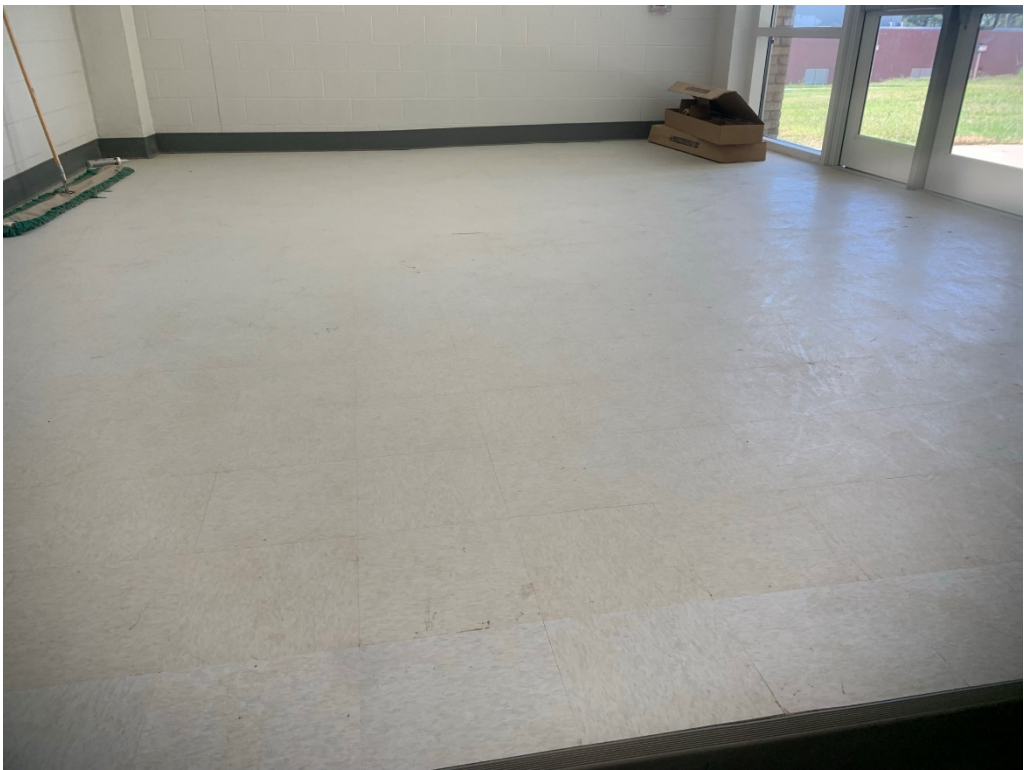
Figure 20 – Floors need cleaning
