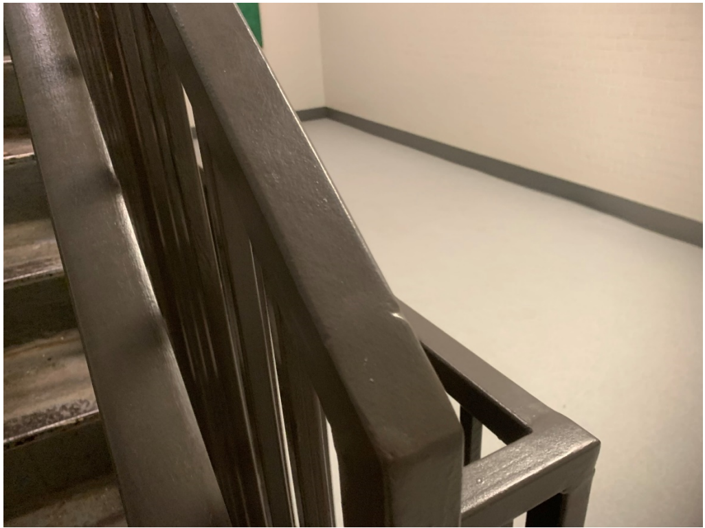
Figure 29 – Guardrails need repair for smooth appearance
