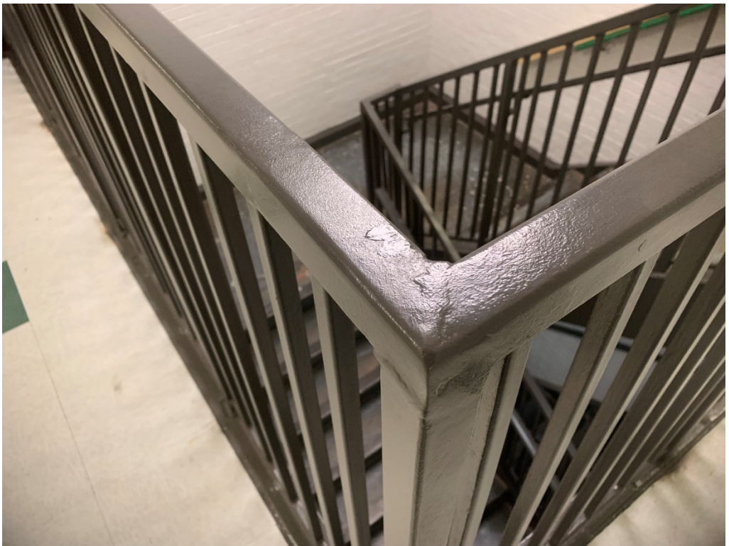
Figure 36 – Guardrails need repair for smooth appearance
