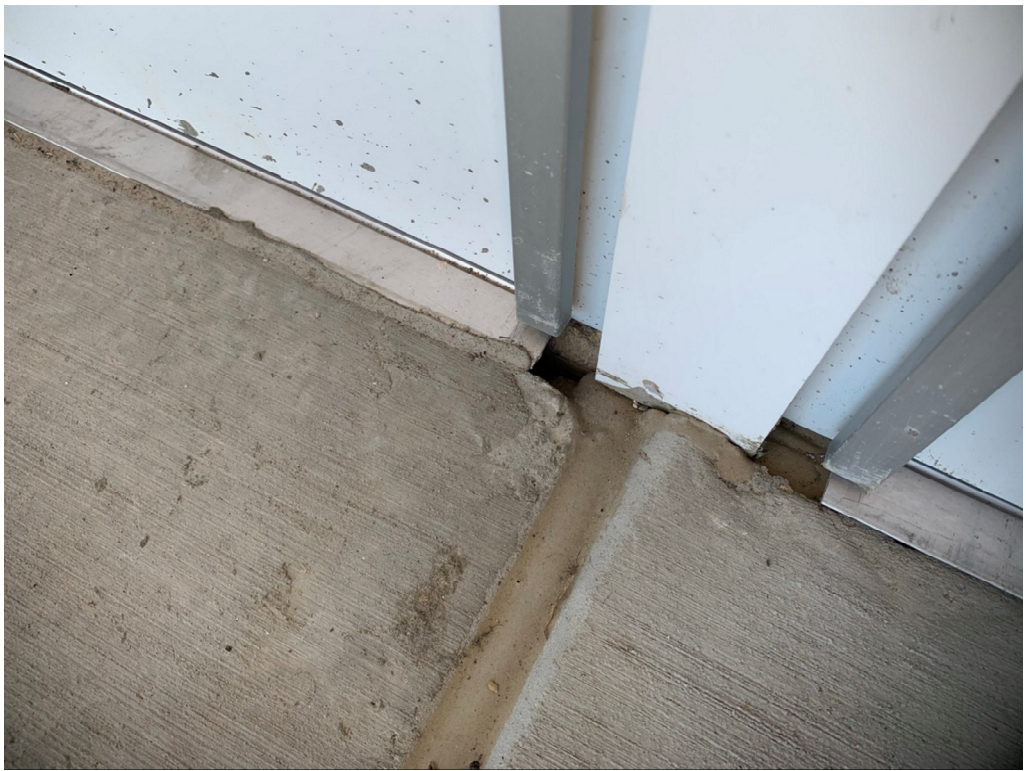
Figure 6 – Fill in gaps between concrete porch and slab at storefront install at entrance
