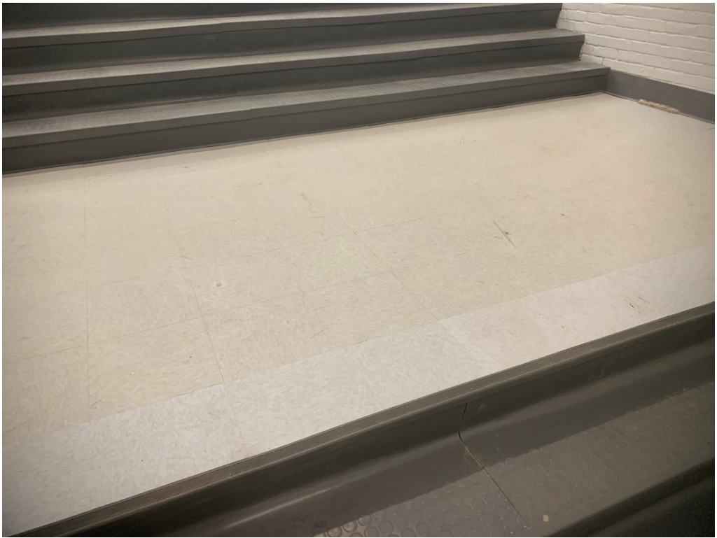
Figure 19 – Floors need cleaning
