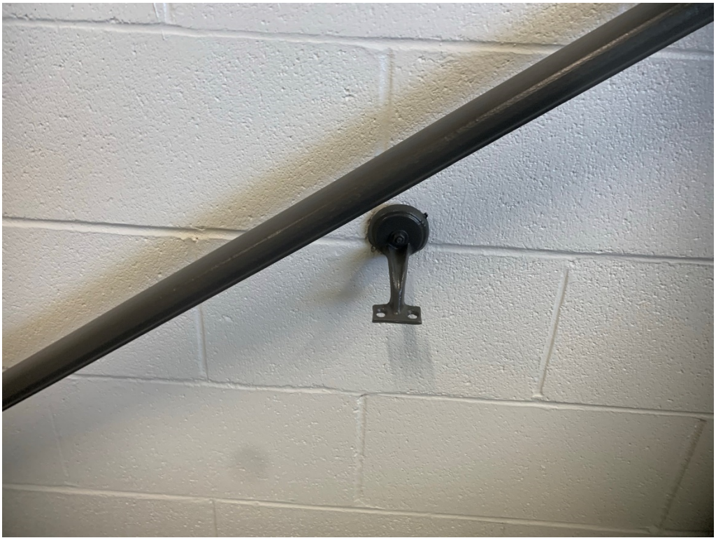
Figure 21 – Handrails missing supports
