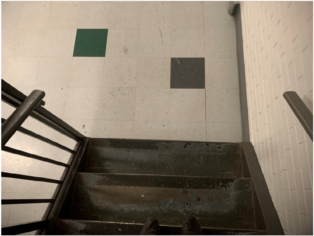
Figure 41 – Handrail does not extend 12" past last step
