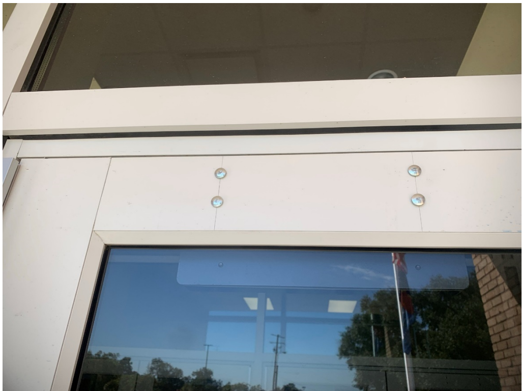
Figure 8 – Construction marks still present at New Doors
