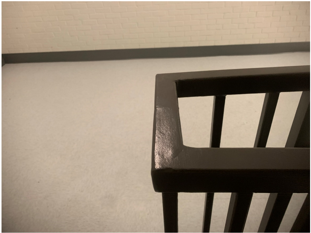
Figure 31 – Guardrails need repair for smooth appearance
