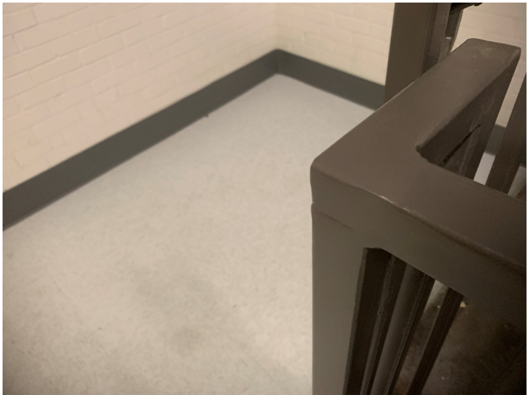
Figure 30 – Guardrails need repair for smooth appearance
