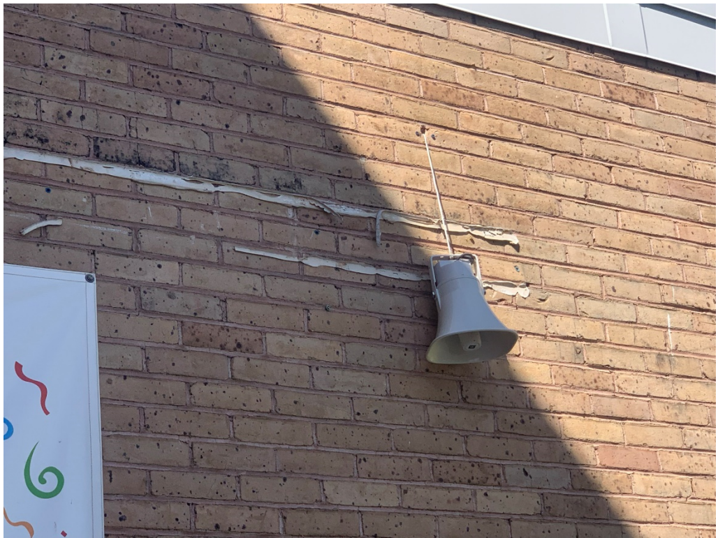
Figure 3 – Caulk still present at demoed awning; anchor mega phone
