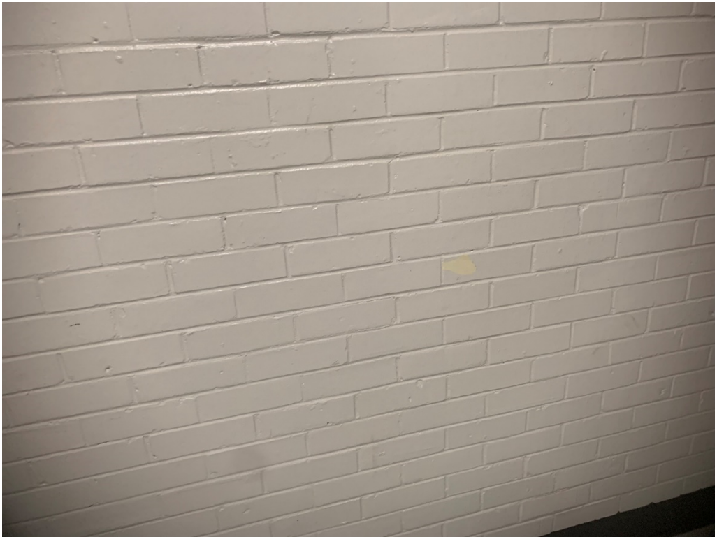
Figure 35 – Paint peeling at walls in cooridor
