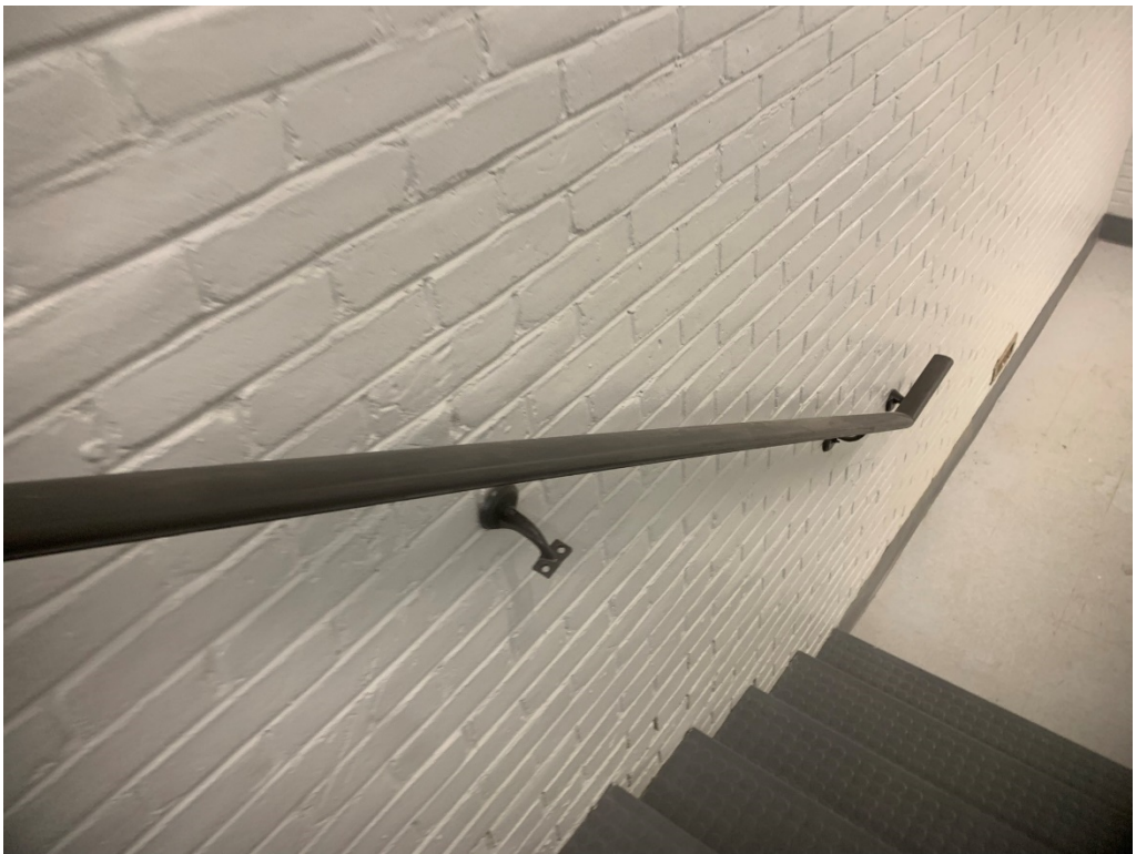
Figure 22 – Handrails missing supports
