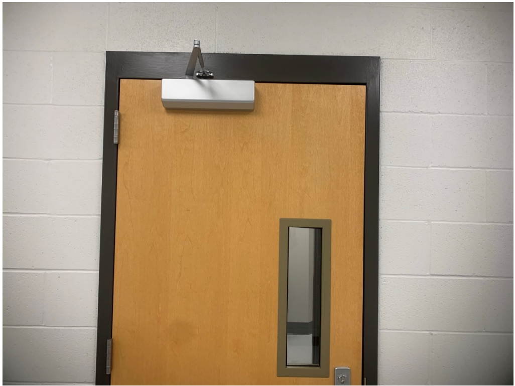
Figure 17 – Door 215 needs to be adjusted (crooked in frame)
