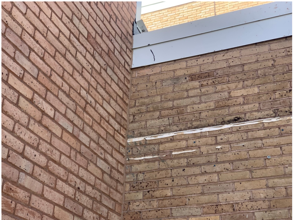
Figure 2 – Roof tar still present from new construction
