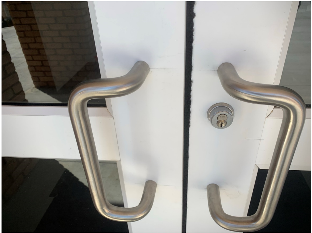
Figure 9 – Construction marks still present at New Doors
