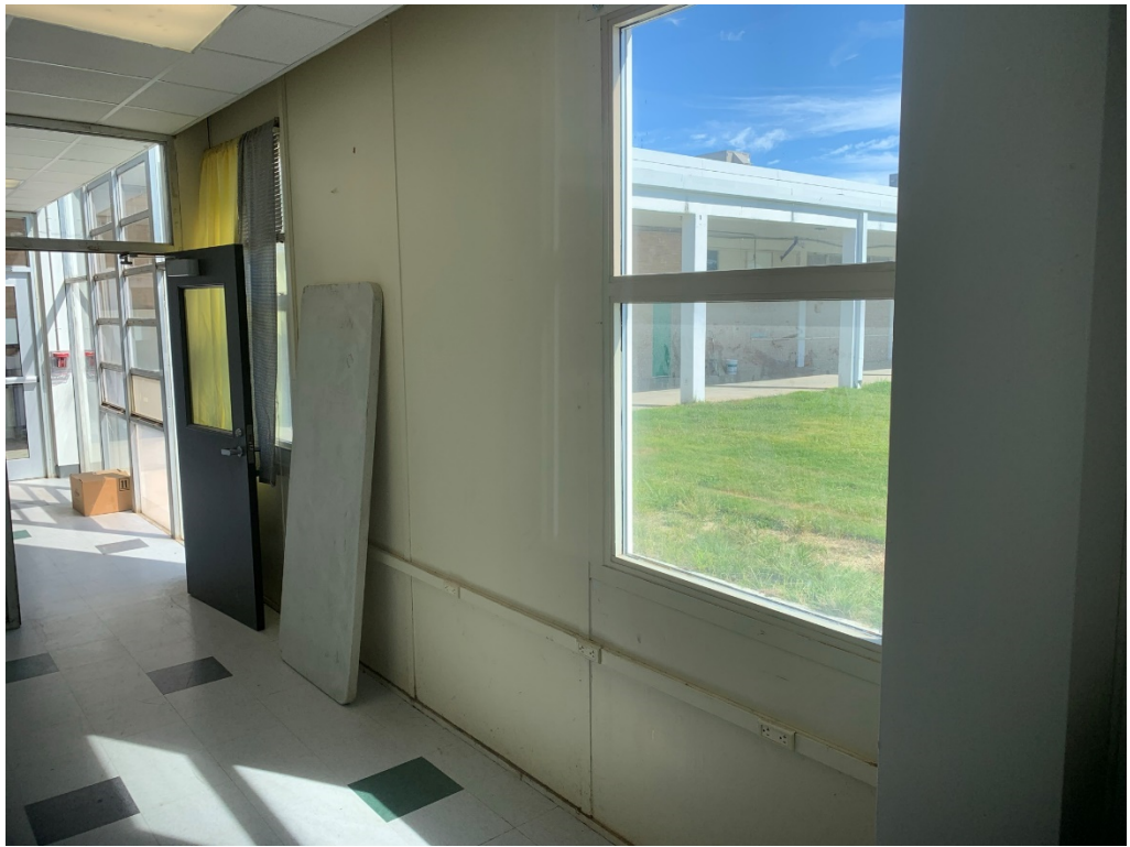
Figure 47 – Wall Missing Paint
