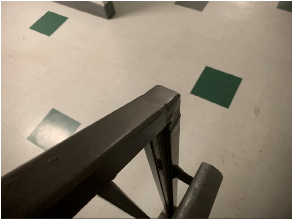
Figure 39 – Guardrails need repair for smooth appearance
