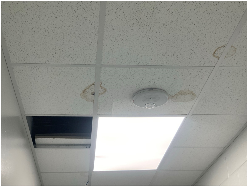
Figure 11 – Leaks still present at A-212
