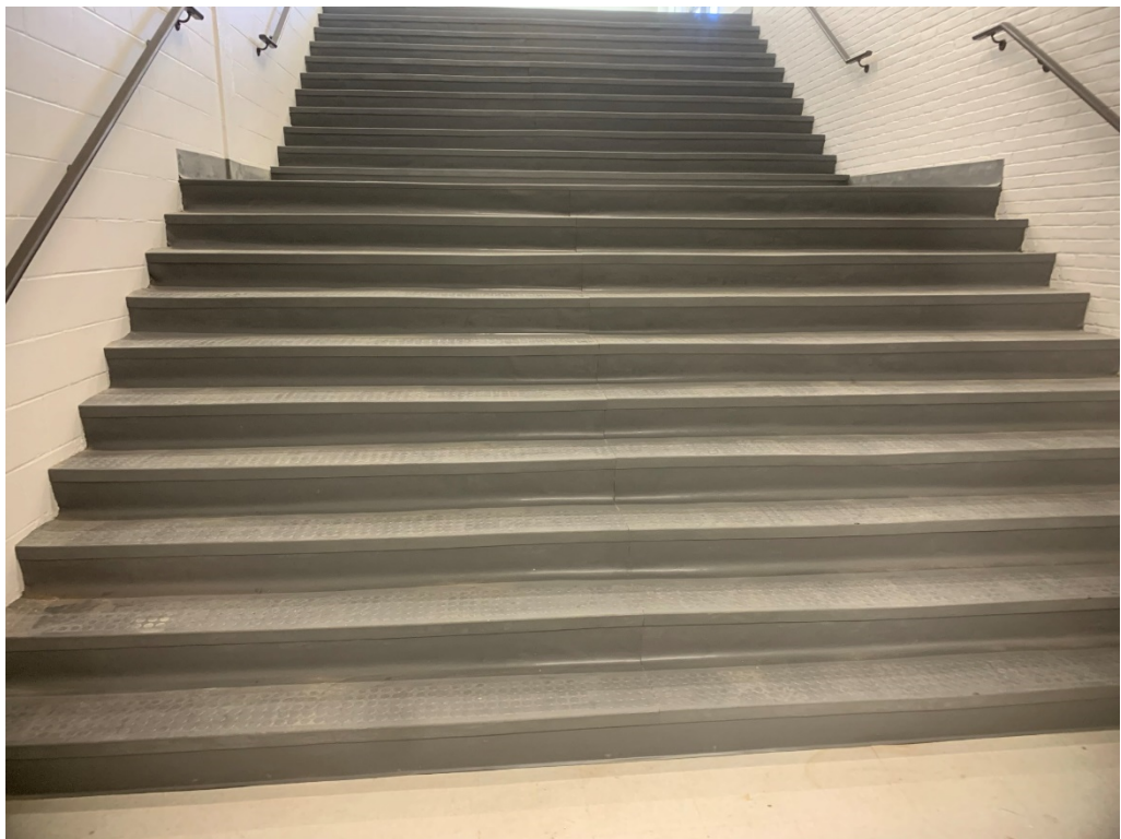
Figure 18 – Floors need cleaning
