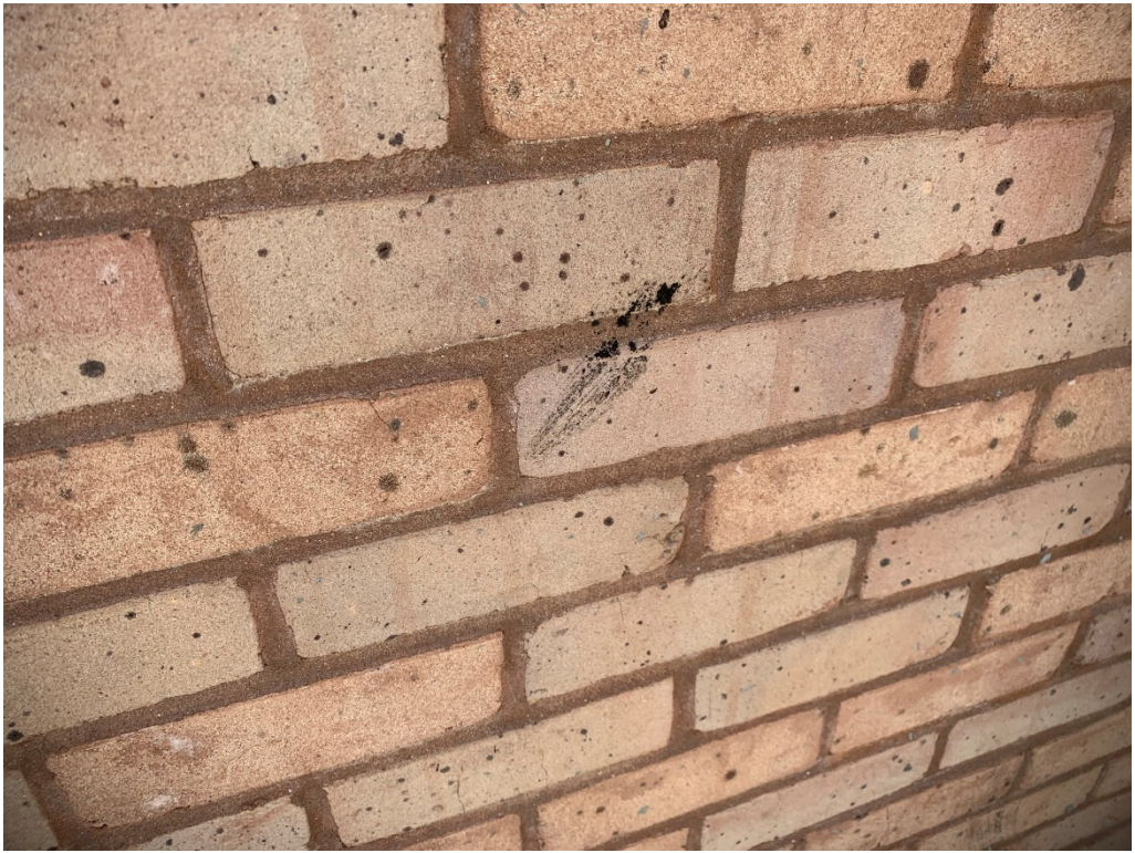
Figure 3 – Asphalt from Roof Work on Brick
