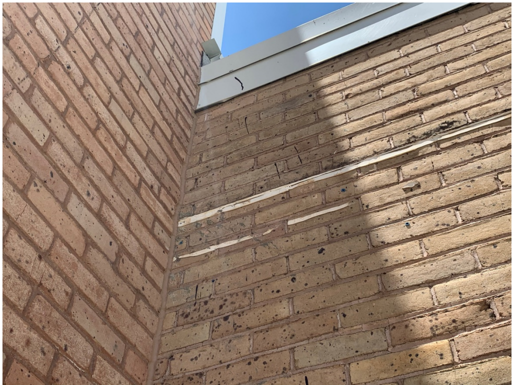
Figure 2 – Asphalt from Roof Work on Brick & Flashing
