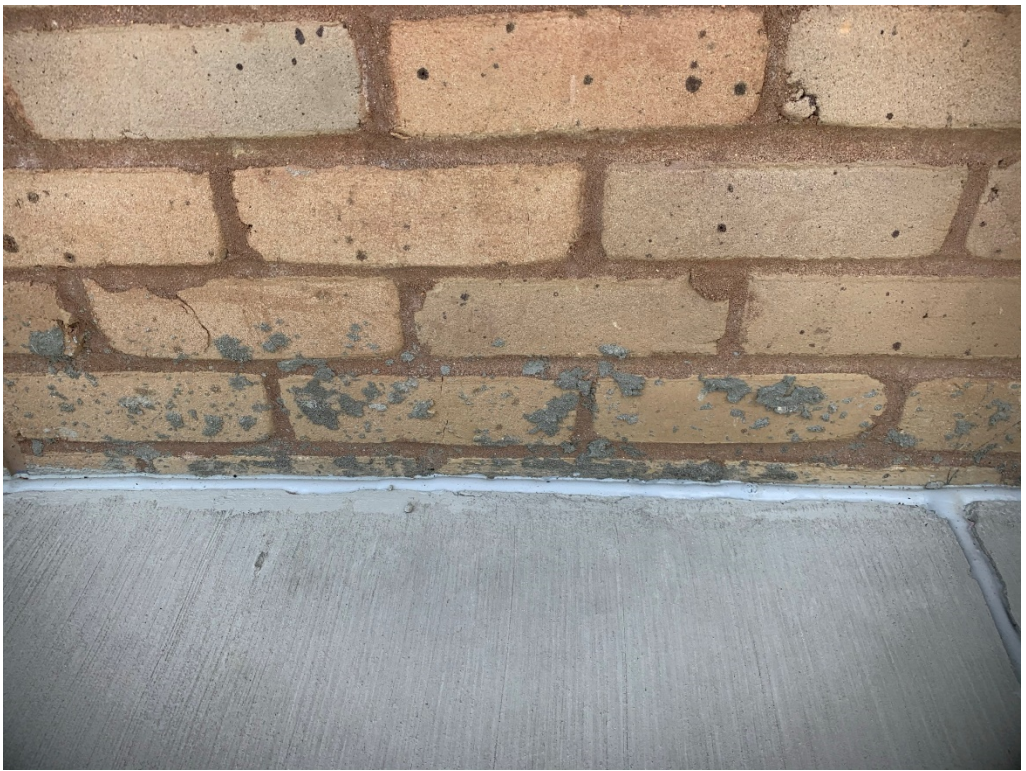
Figure 4 – Concrete Splatter to be Removed
