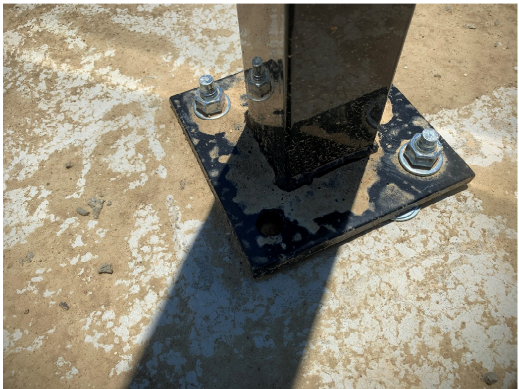
Figure 8 – Missing Concrete Anchors in Some Installed Members
