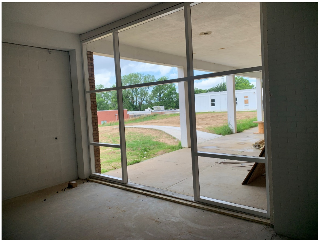
Figure 10 – Storefront; will interior of porch area be raised for final floor level to match threshold?
