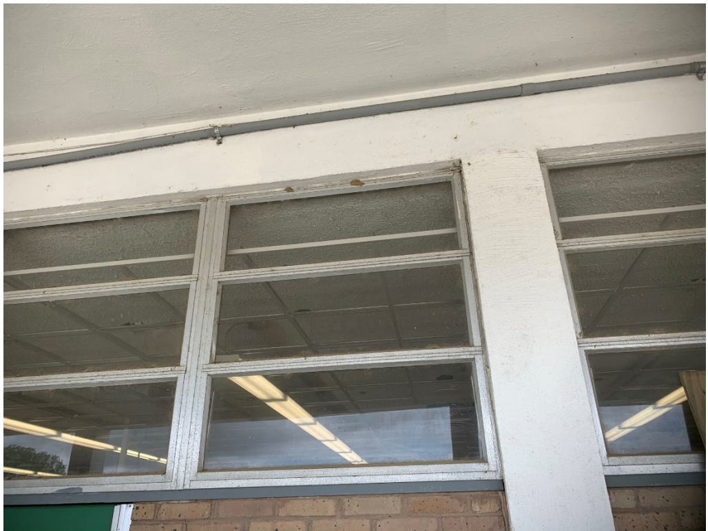
Figure 11 – Library ceiling needs finishing at end where window shows above new ceiling
