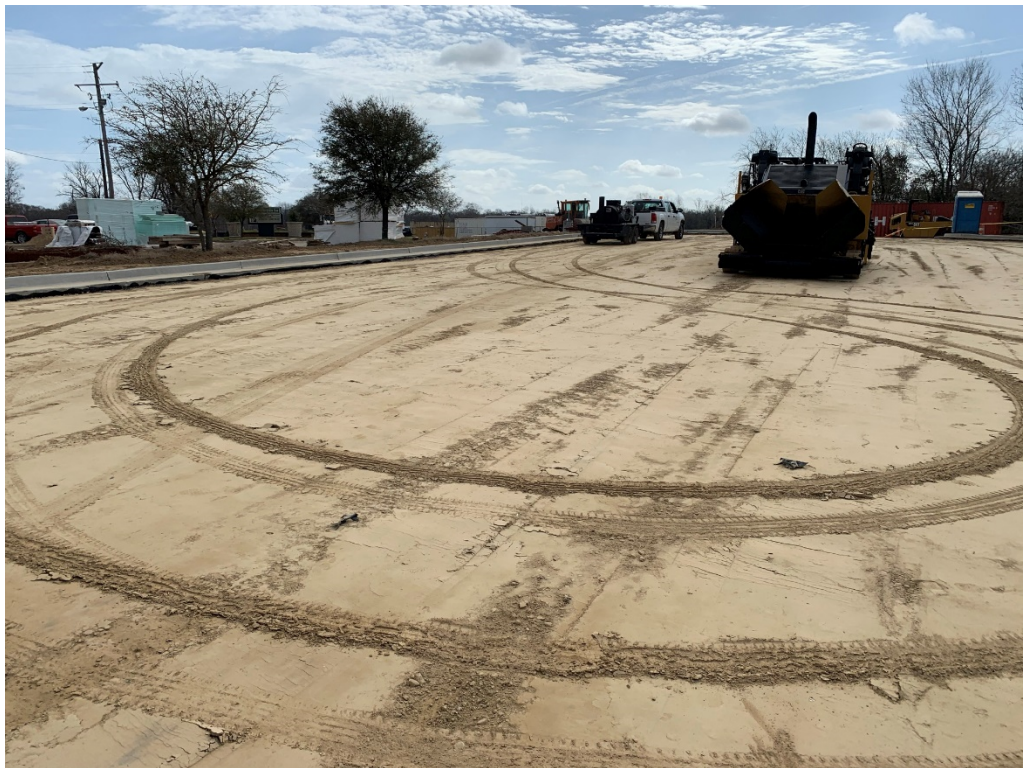
Figure 2 – Parking Lot Compacted (per OAC meeting requires additional verification of compaction after Weather Event)
