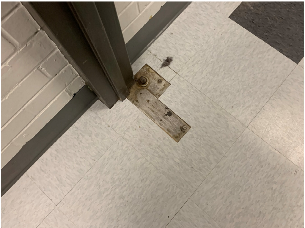
Figure 10 – VCT Should Overlay this Inset Piece of Hardware (at multiple locations)
