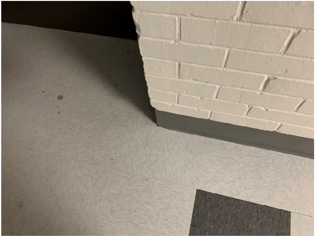
Figure 9 – Pre-Formed Corners are Required per Contract Documents at all Outside Corners
