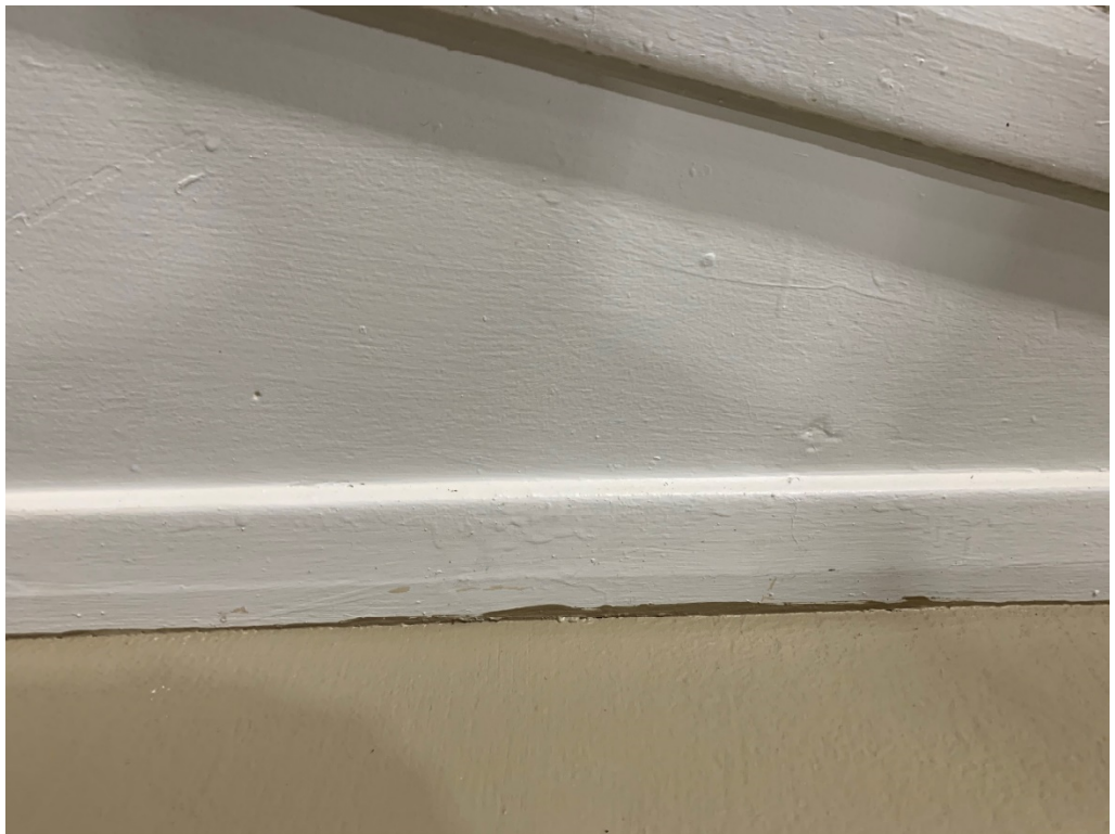
Figure 12 – Paint Touchups required at Base Throughout
