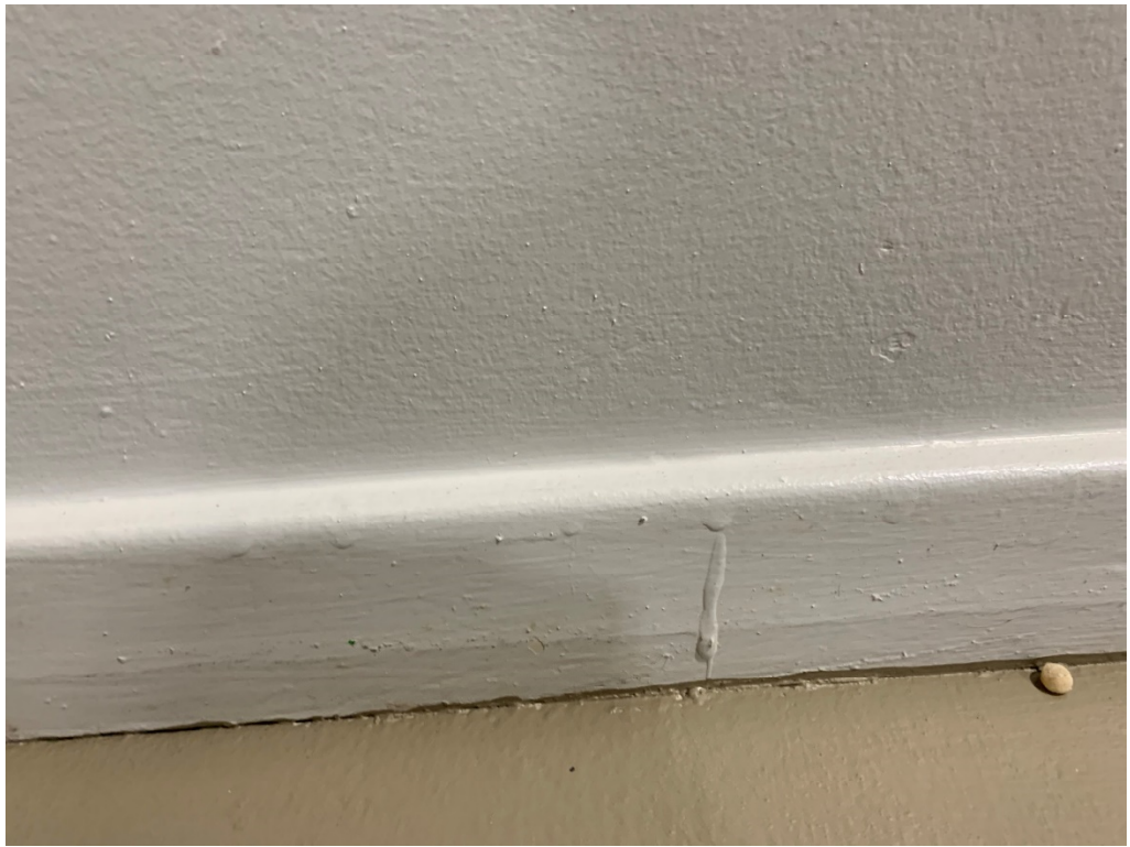
Figure 13 – Existing Drips Should be scraped/removed before new paint is applied
