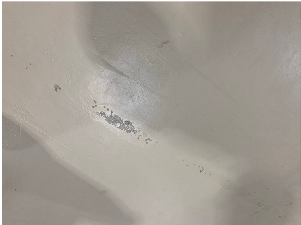
Figure 14 – Damage at Flooring in Auditorium
