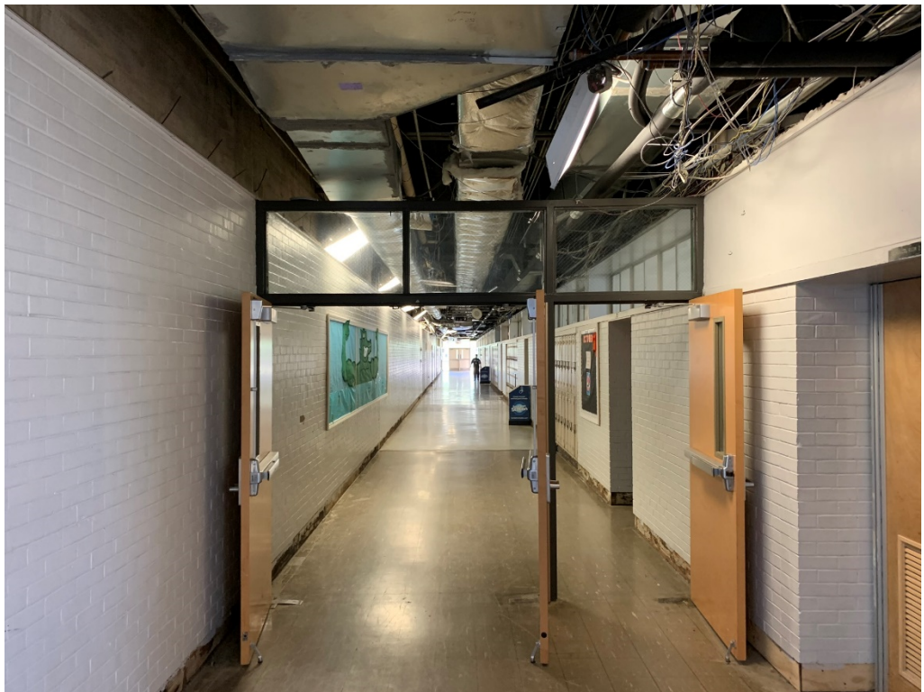
Figure 20 – Corridor E-215 New Ducting will Still be an Issue for the Second half of this Hallway
