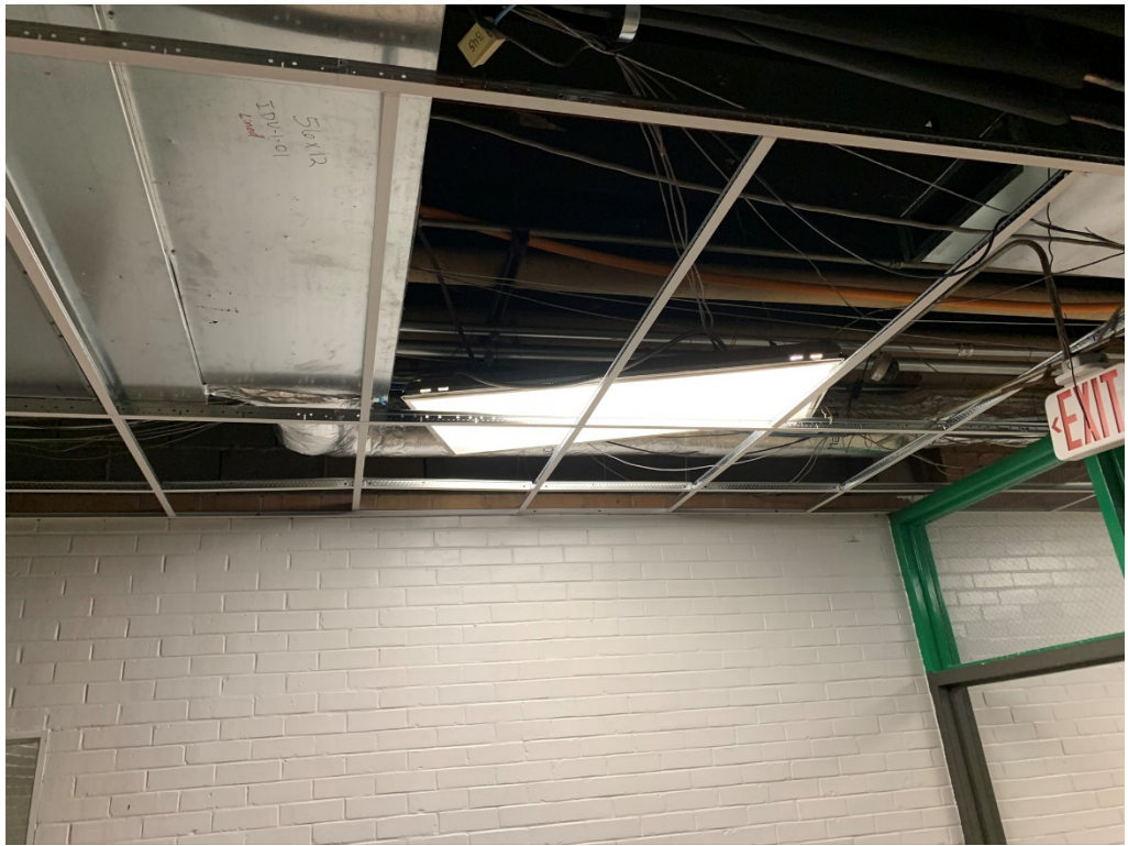
Figure 17 – New Ducting has not been Coordinated with Lighting Layout (limited to 2 place so far)
