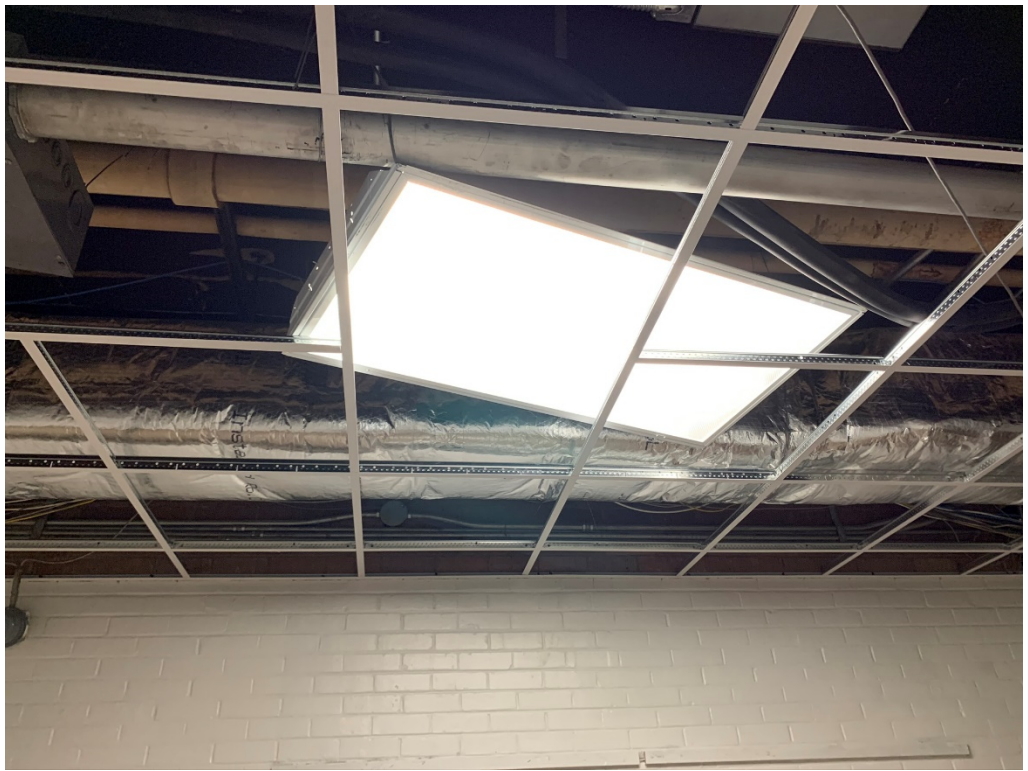
Figure 16 – New Ducting has not been Coordinated with Lighting Layout (limited to 2 place so far)
