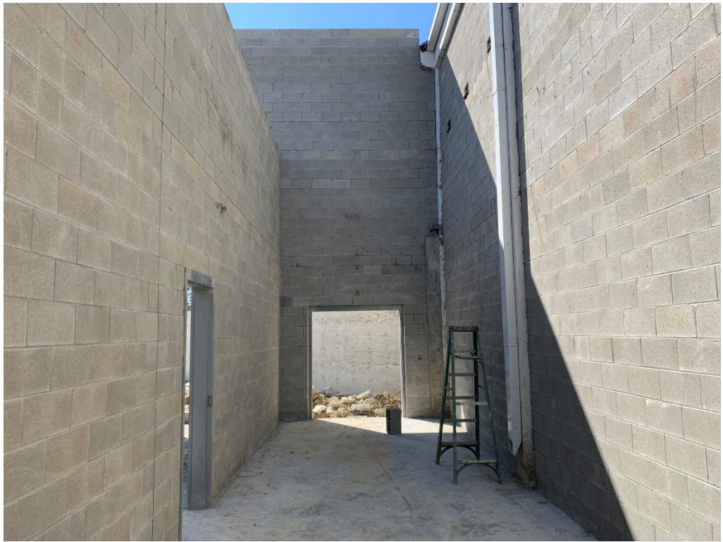
Figure 5 – Corridor A-202 Blocked In
