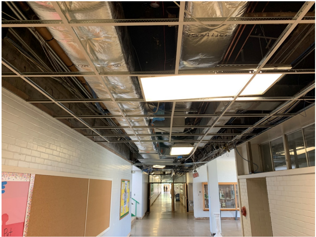
Figure 19 – Corridor E-215 New Ducting is Not Coordinated with Lighting Layout
