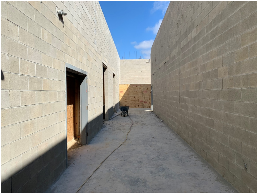
Figure 4 – Corridor A-202 Blocked In
