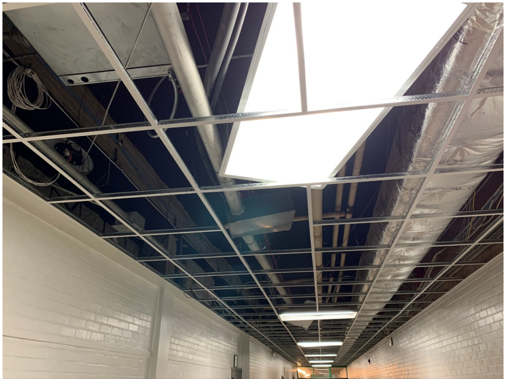
Figure 14 – Existing Conduit in Way of Light Install (Can this conduit be raised?)
