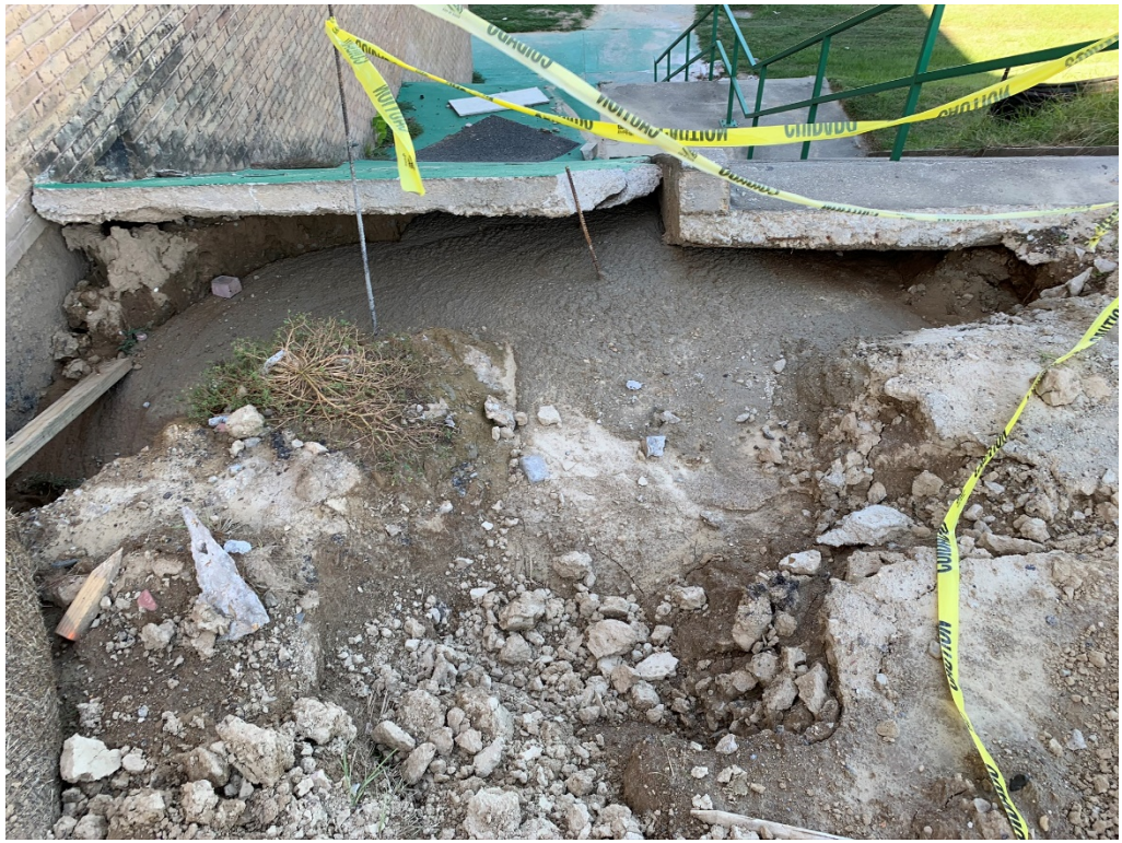
Figure 5 – Eroded Dirt Filled
