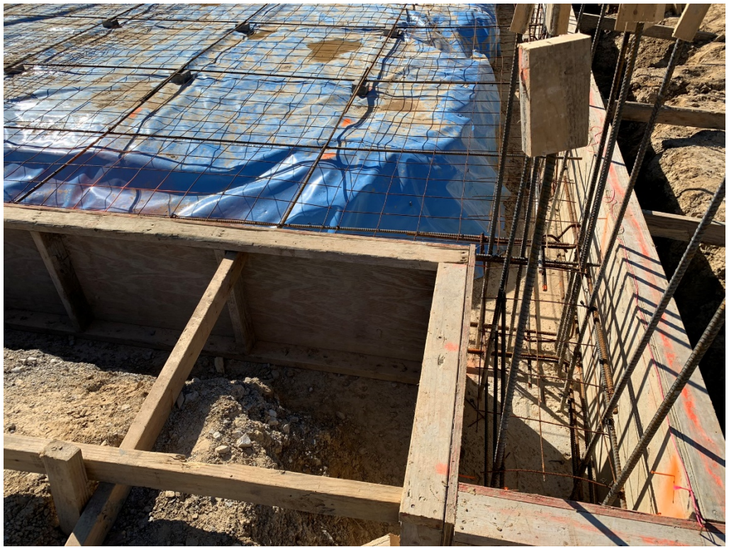
Figure 4 – Northeast Edge of Slab
