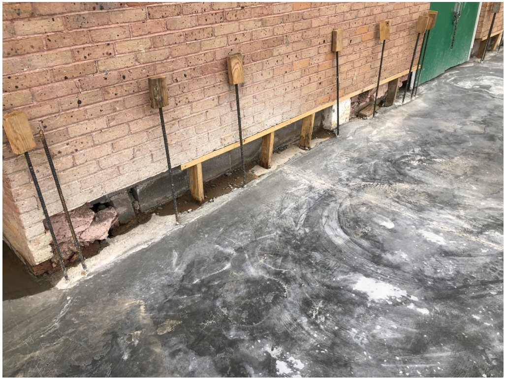
Figure 5 – Brick Temporarily Supported
