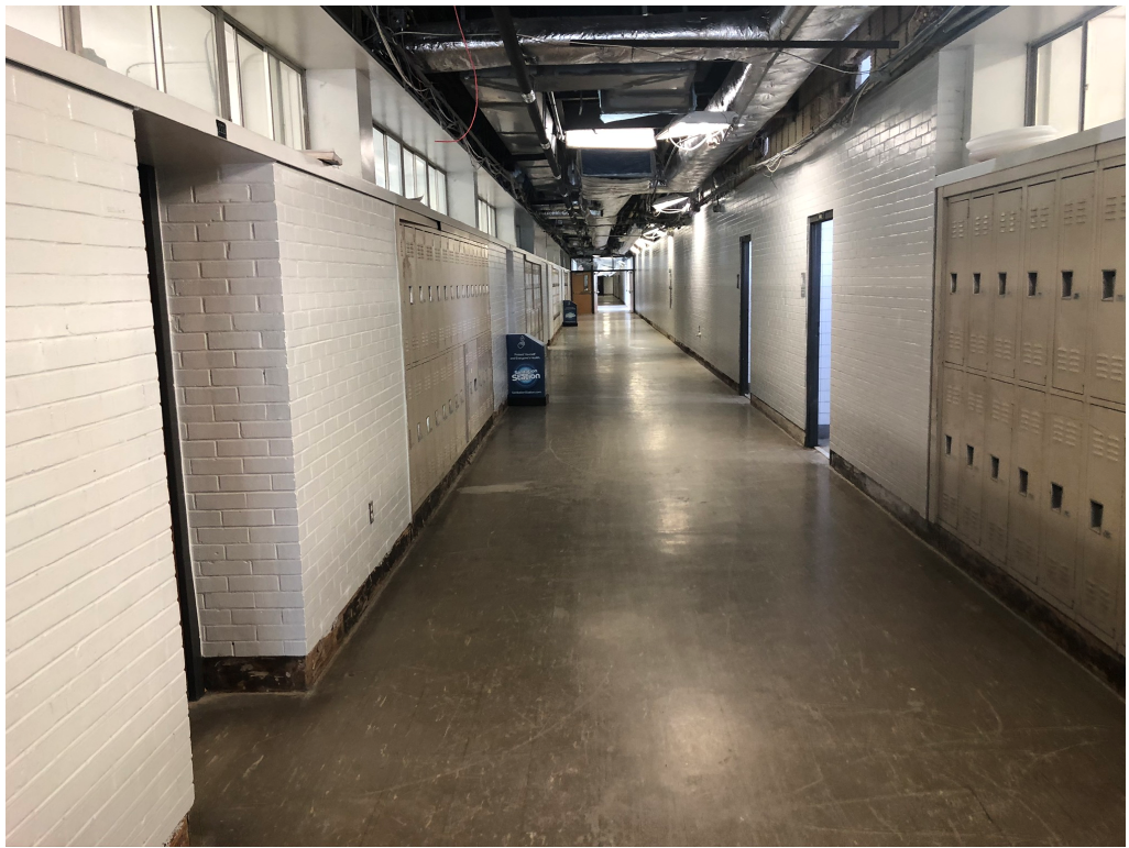
Figure 13 – Paint at Interior Corridor
