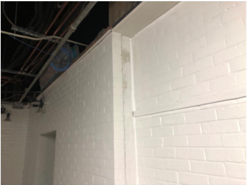
Figure 10 – Paint touch Ups Still Required
