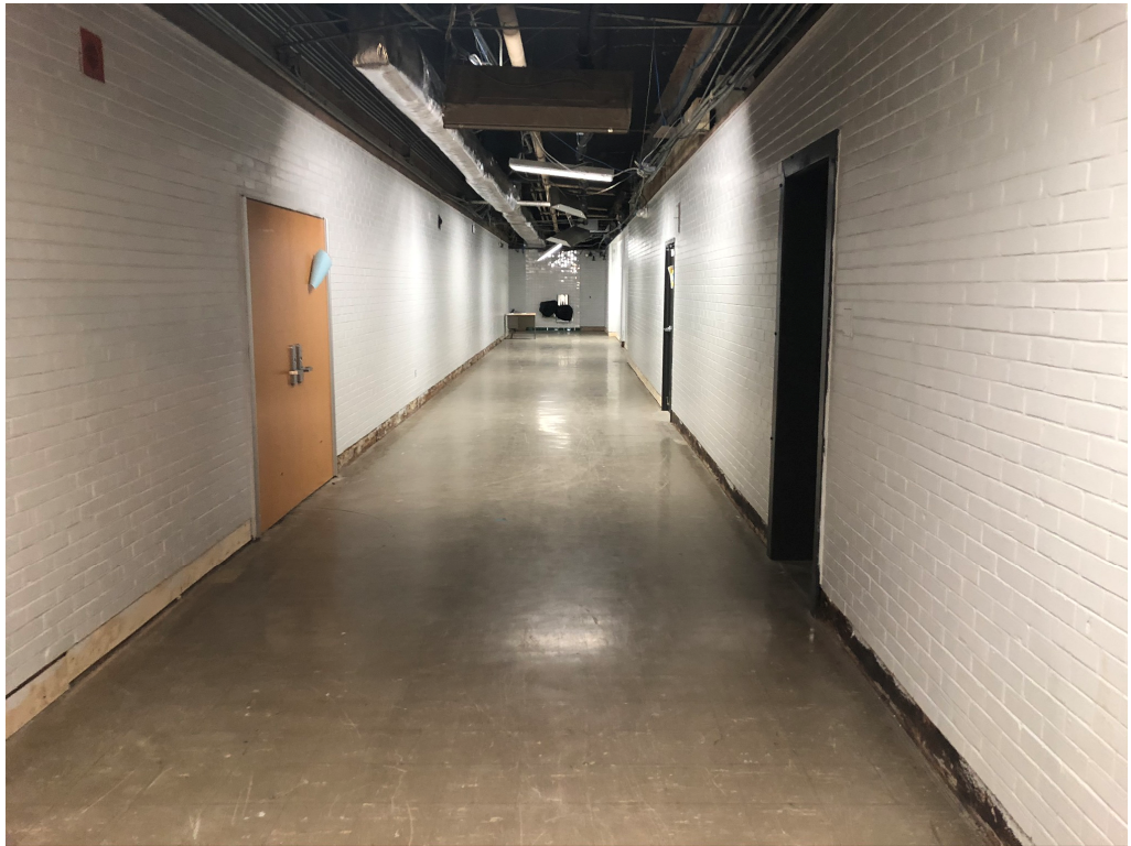
Figure 6 – Paint at Interior Corridor
