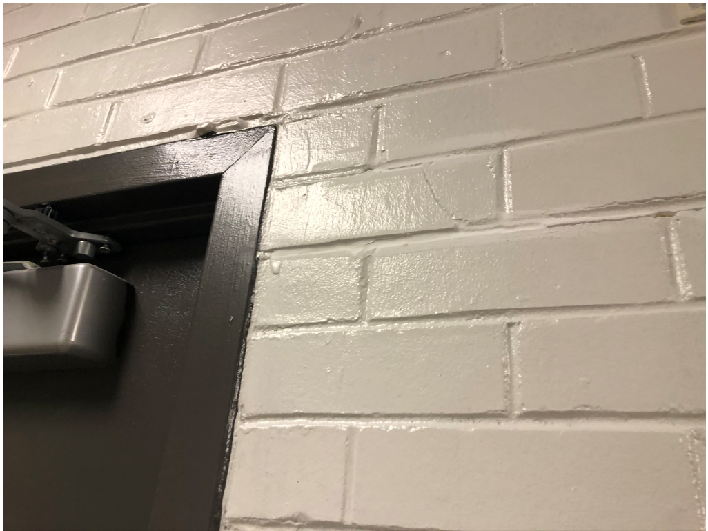
Figure 8 – Paint touch Ups Still Required
