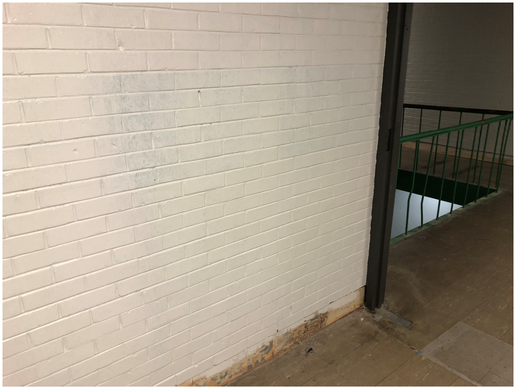
Figure 11 – Some Area only Appear to have a Single Coat
