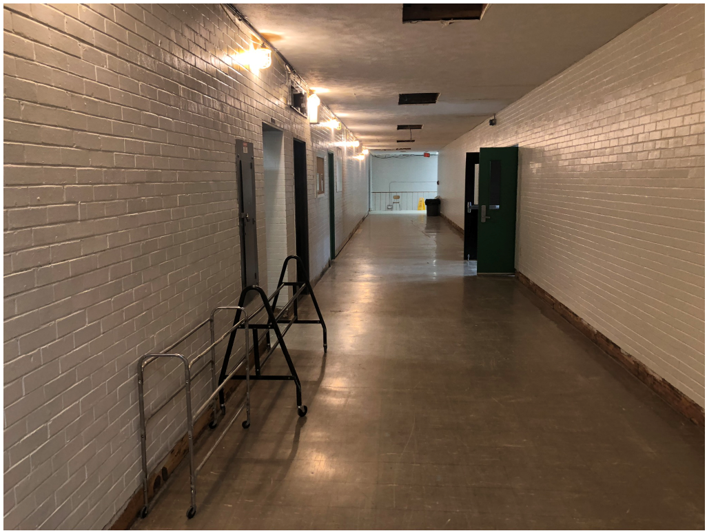
Figure 7 – Paint at Interior Corridor
