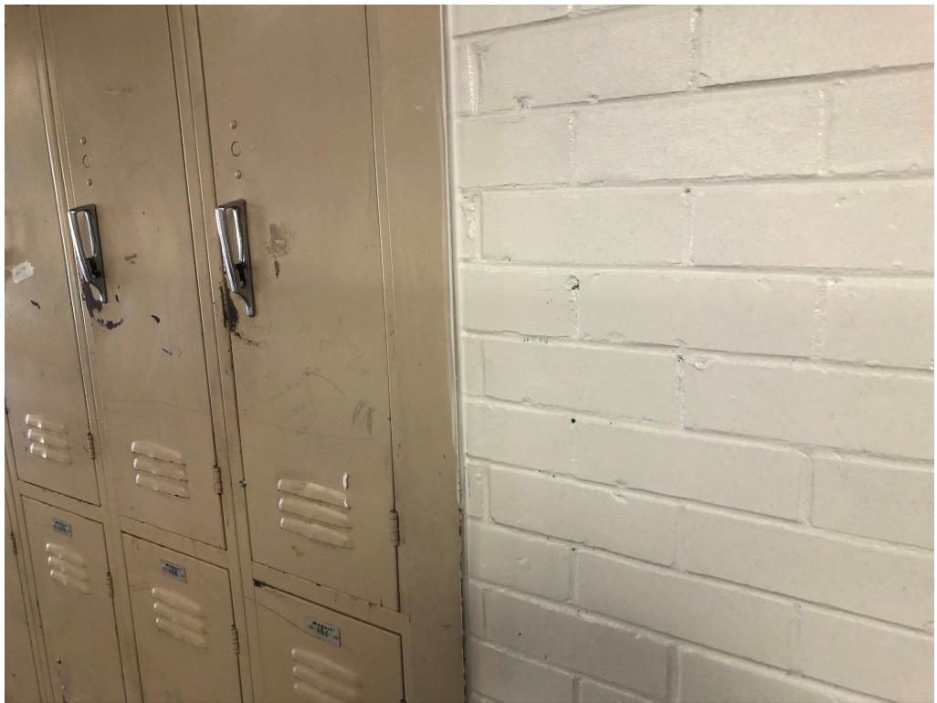
Figure 12 – Paint touch Ups Still Required
