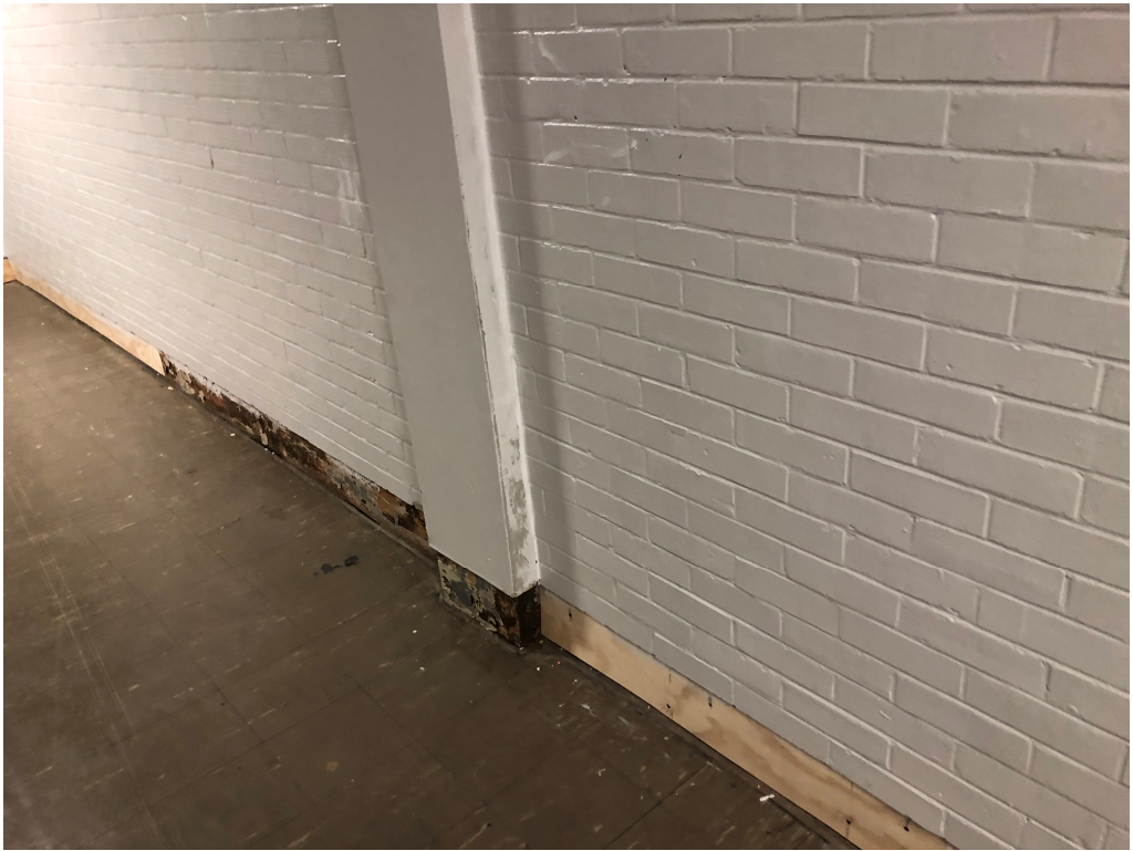
Figure 9 – Paint touch Ups Still Required
