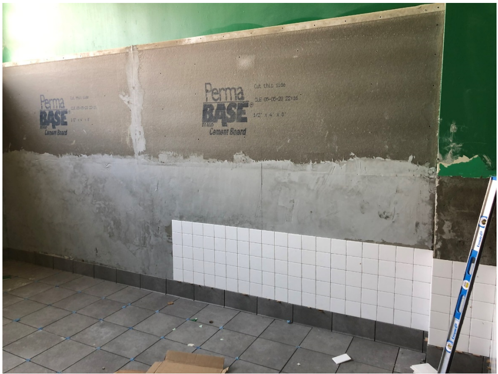
Figure 5 – E-226C Bathroom Tile
