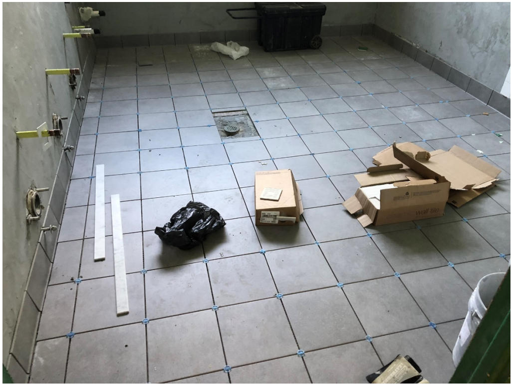
Figure 3 – E-226C Bathroom Tile
