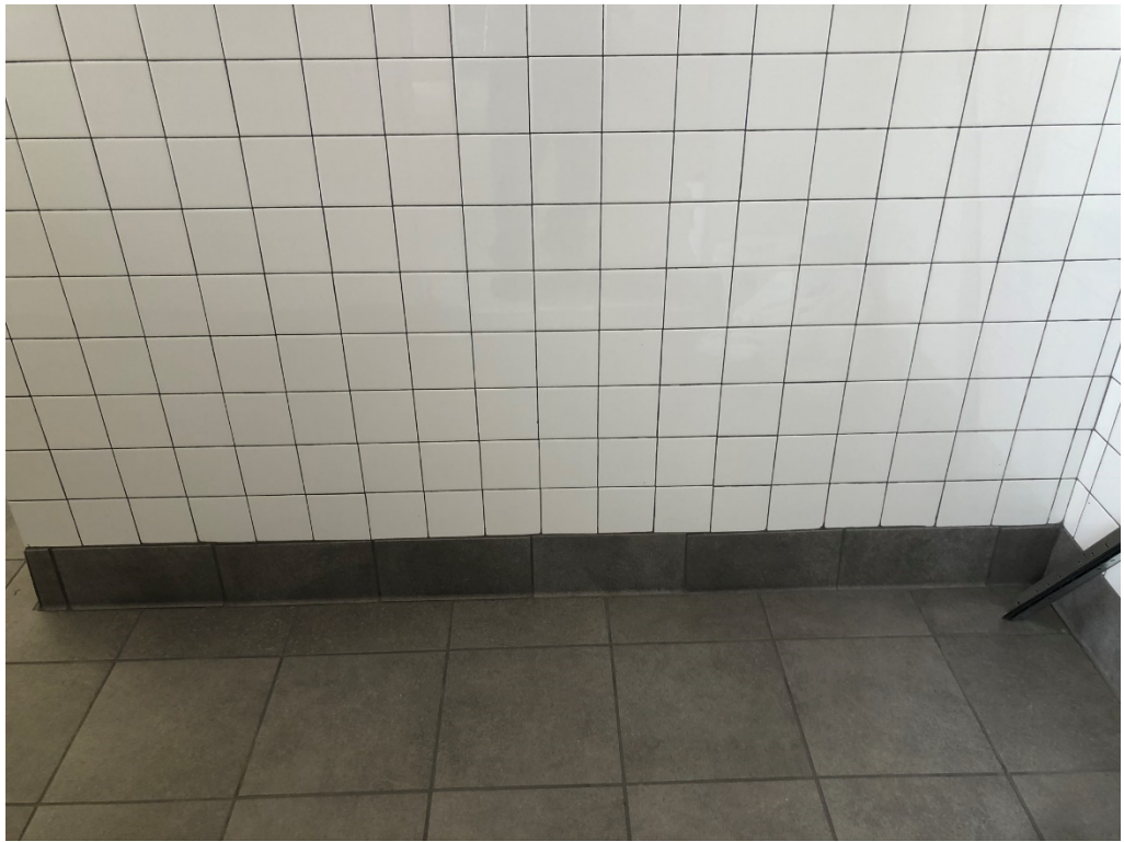
Figure 15 – E217A Bathroom (crooked tile base needs to be reset for flush appearance)
