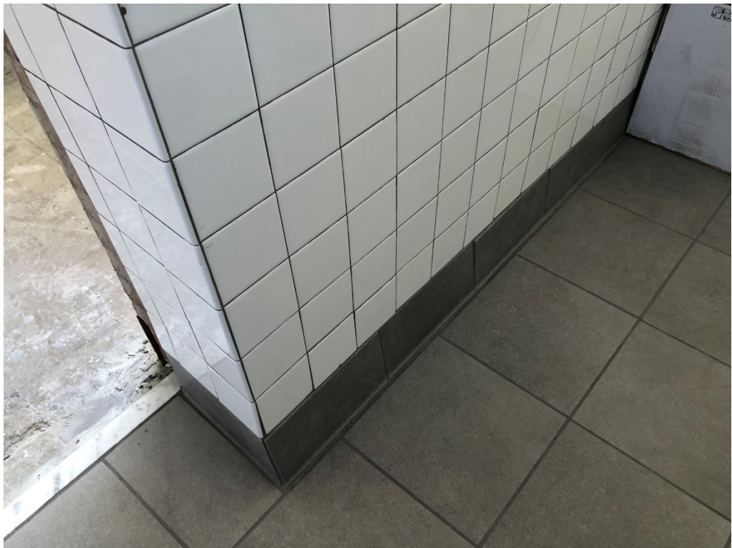
Figure 16 – Tile Base needs to be reset and floor tile need a sliver of tile to make up gap
