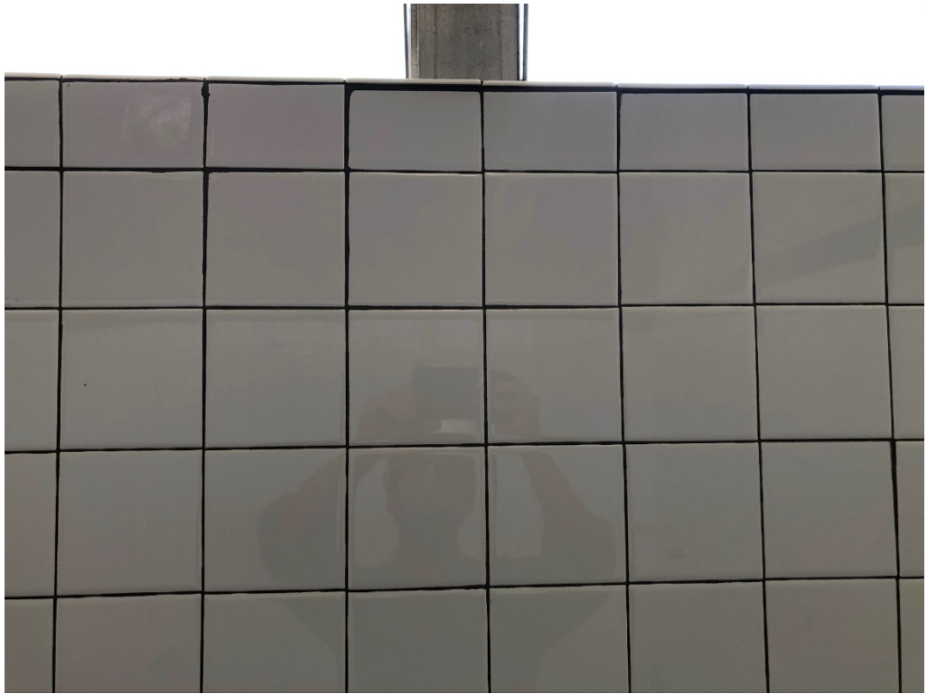
Figure 19 – E217A Bathroom (tile at top of wall needs to be reset)
