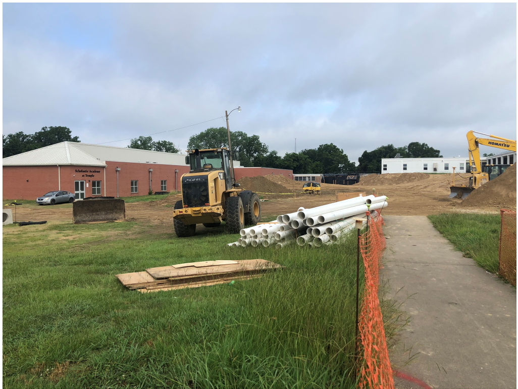
Figure 2 – Drainage Pipe On Site
