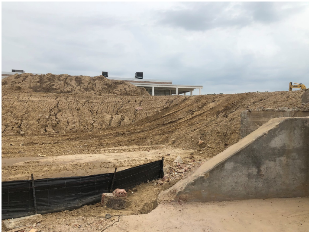
Figure 8 – Dirt Work Erosion
