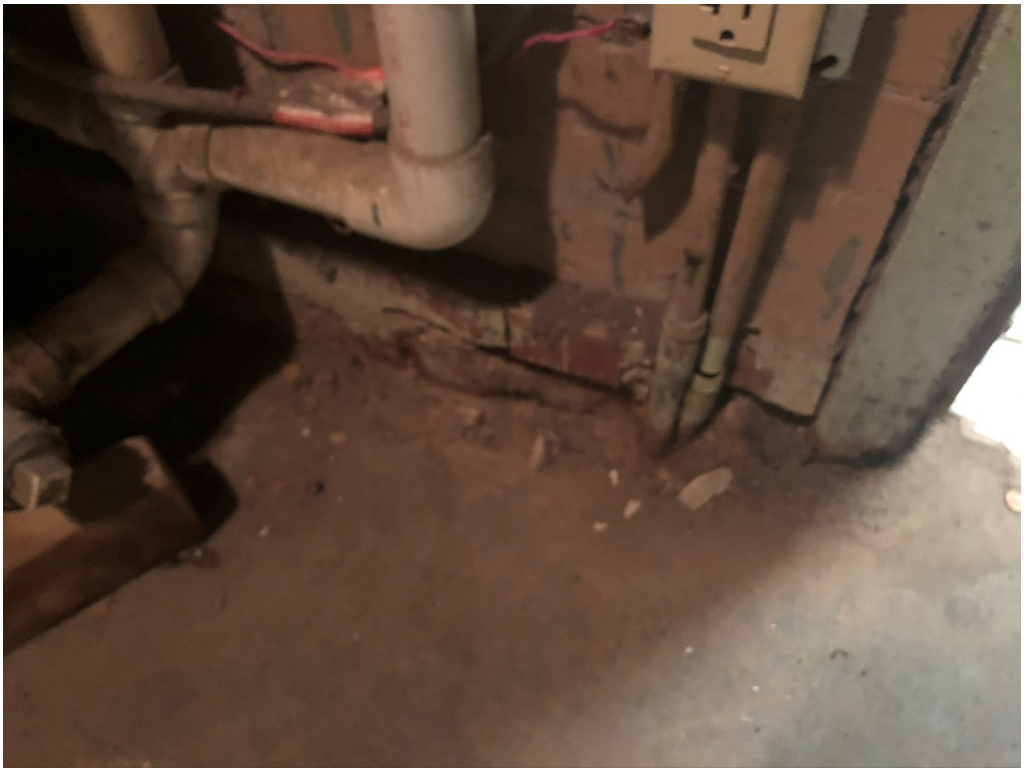
Figure 3 – Offset in lower 2 courses of brick (note mop sink in upper left)
