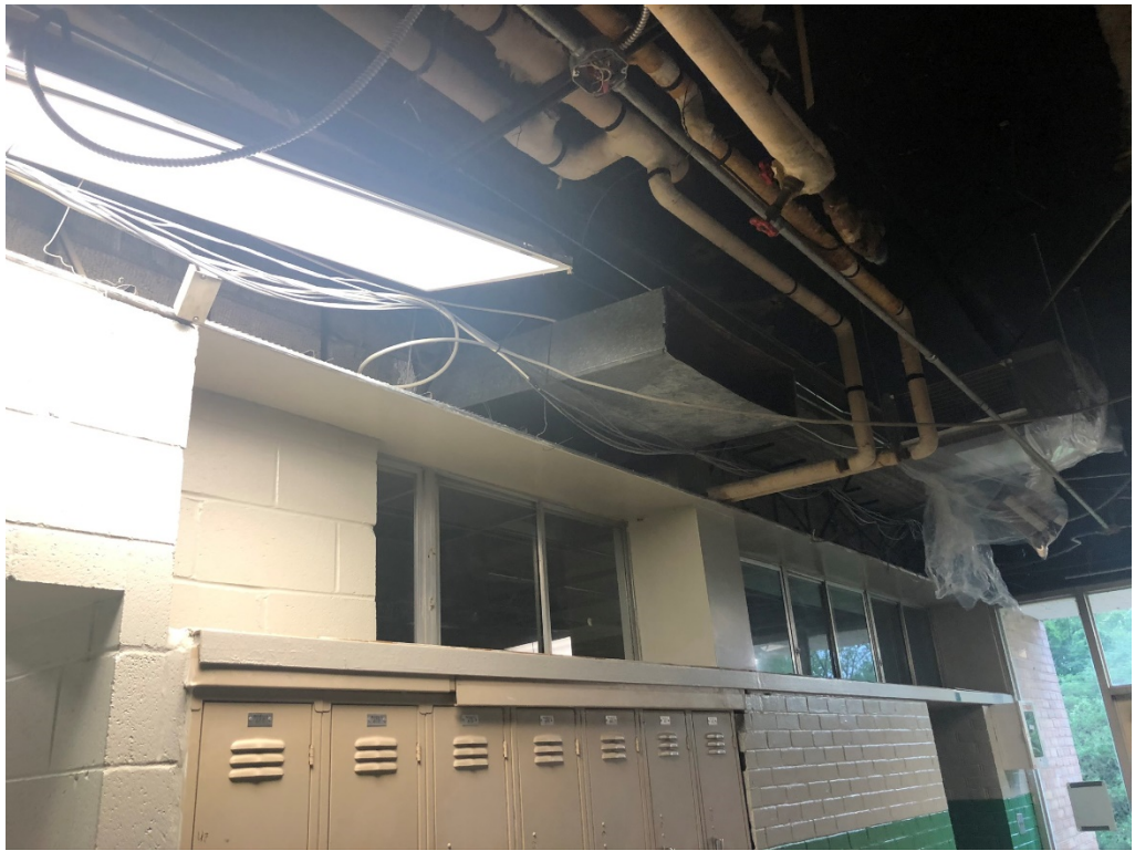
Figure 5 – Return to Sped E-227 (Contractor proposes to cap, leaving room without return)
