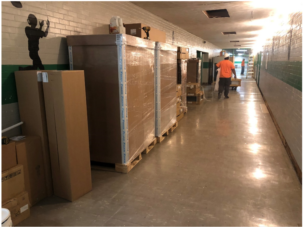
Figure 11 – HVAC Equipment on Site Ready for Install
