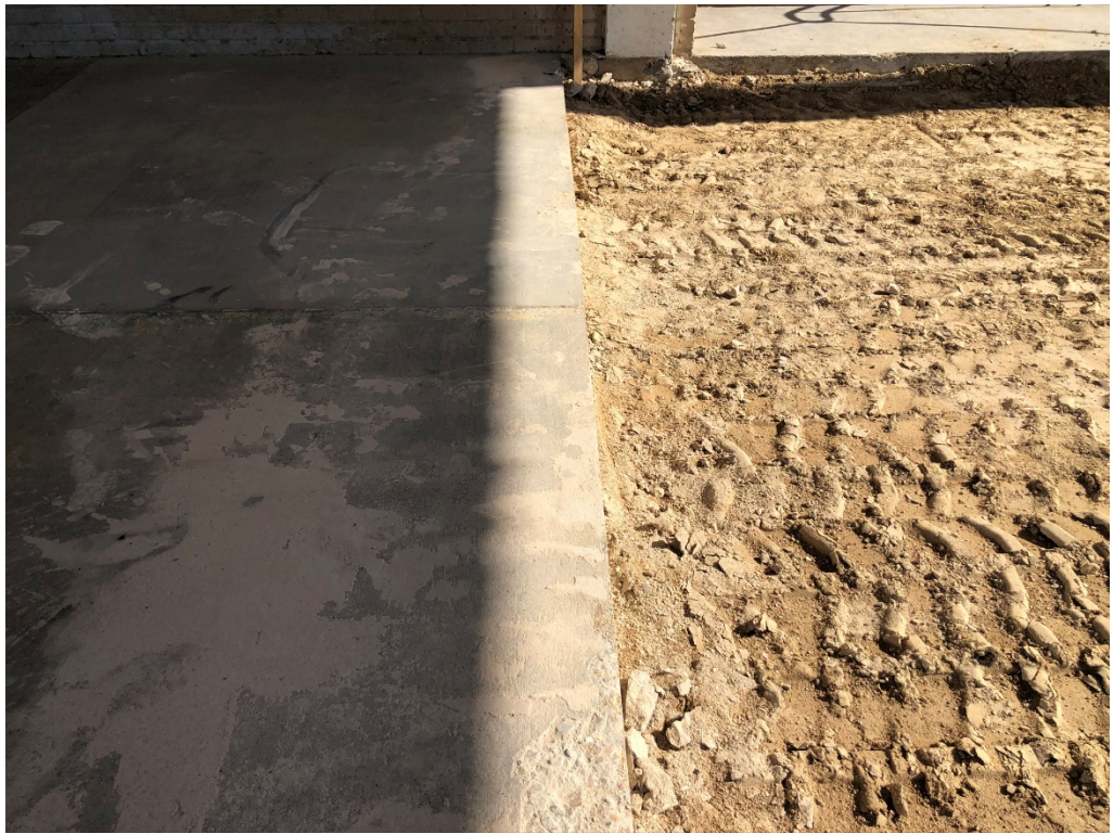
Figure 3 – Saw Cut at Removed Slab (Will Additional Saw Cut be made for 2'-0" Offset?)
