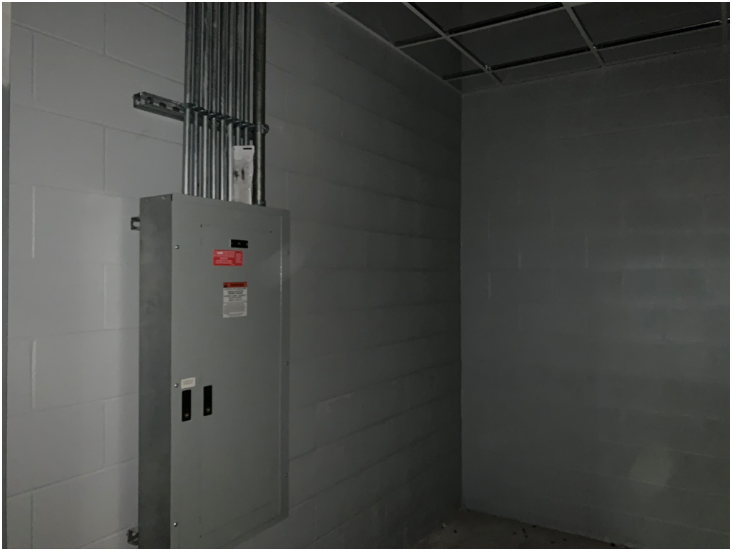
Figure 12 – Electrical Subpanel Installed
