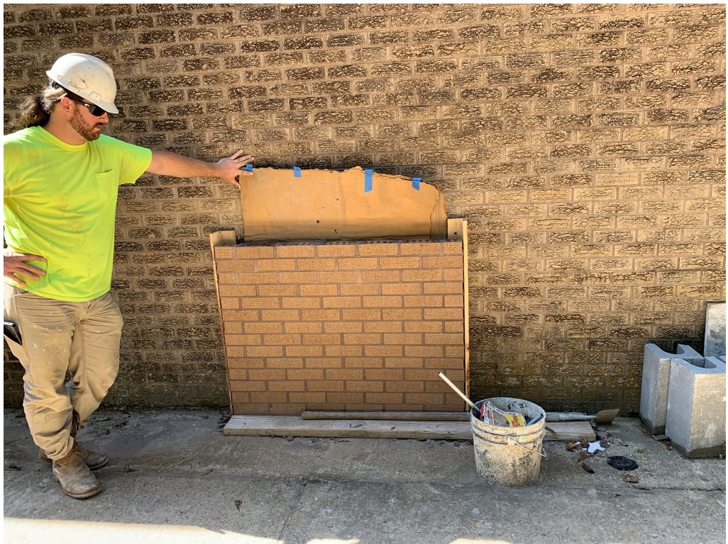
Figure 2 – Mock Up Brick Wall; there's some unevenness in the mortar color
