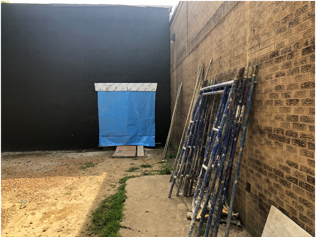
Figure 6 – Mason's Scaffold On Site; Brick to be delivered within the next week
