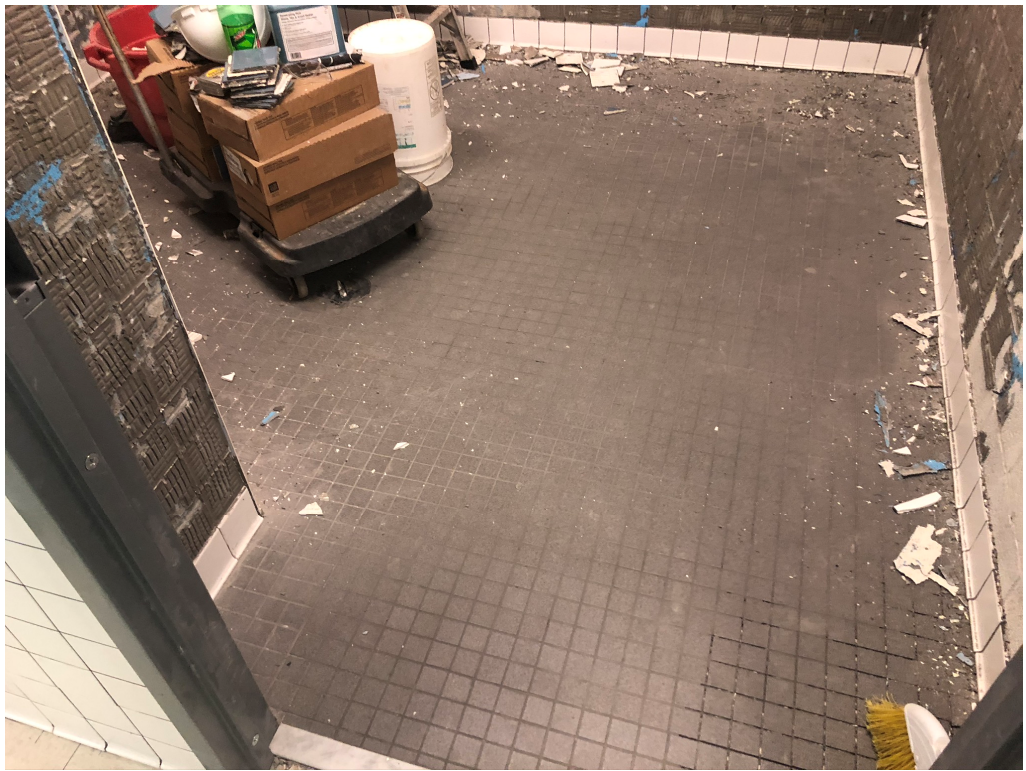
Figure 5 – Floor Tile Installed; Tile rejected is being removed
