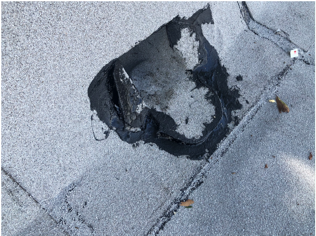
Figure 12 – Roof Outlet; roll roofing needs to be re-adhered
