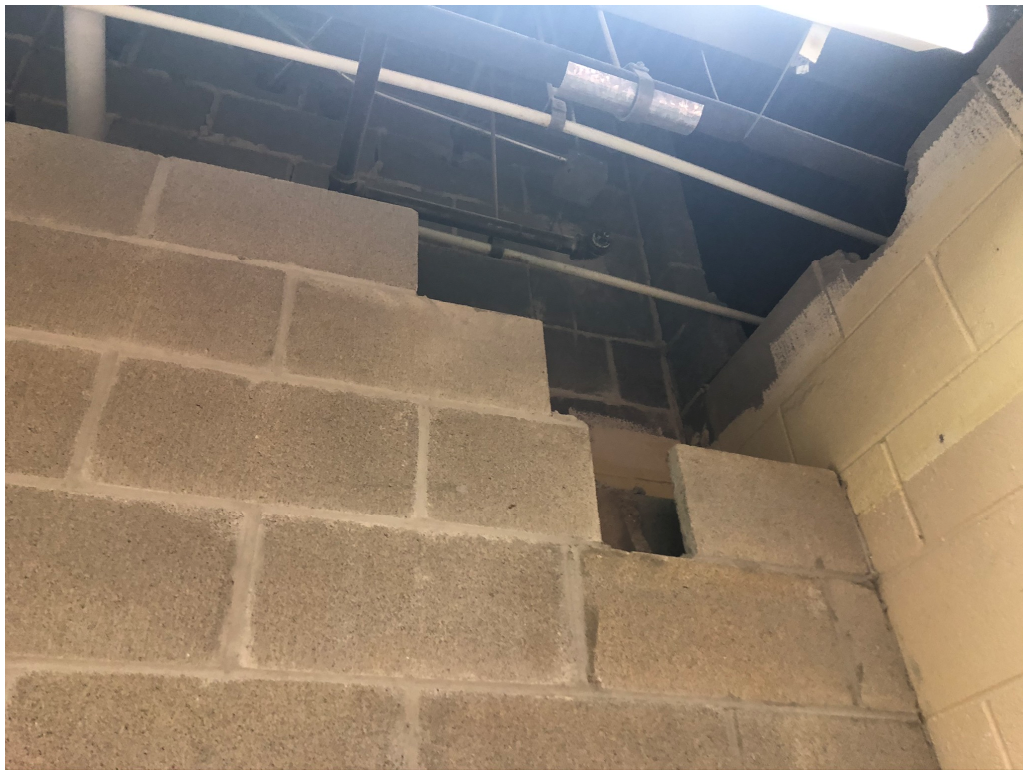
Figure 5 – Sprinkler Head Capped
