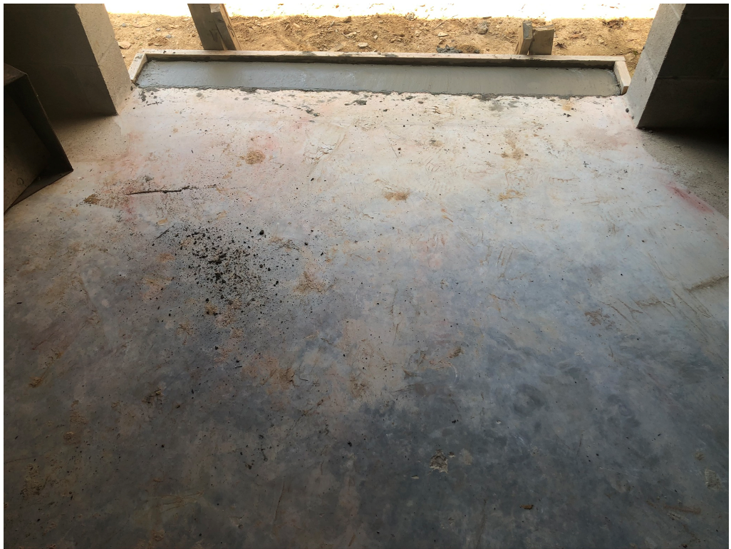
Figure 8 – Opposite End Concrete Step Through Brick Envelope
