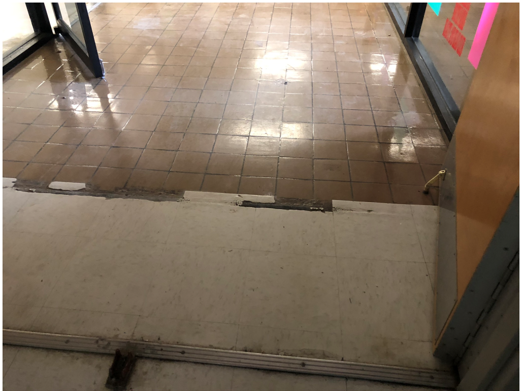
Figure 2 – VCT to be removed to threshold and ceramic tiled overlaid with new VCT
