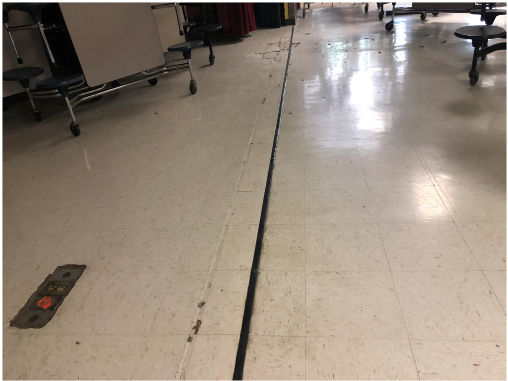
Figure 1 – VCT to be replaced in single row at damage in this photo
