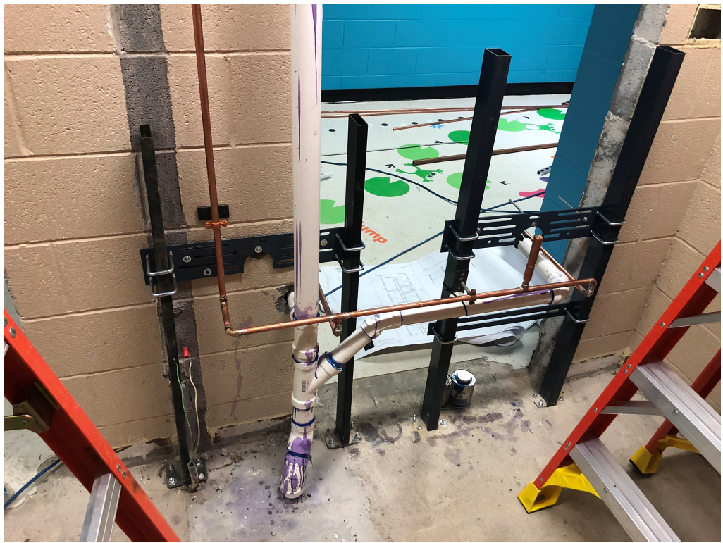
Figure 11 – Plumbing Support for EDF's
