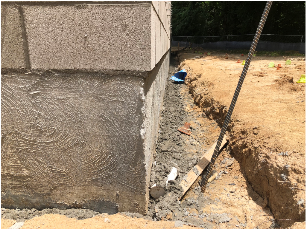
Figure 6 – CMU Wall Offset from Foundation (SDG: Acceptable?)
