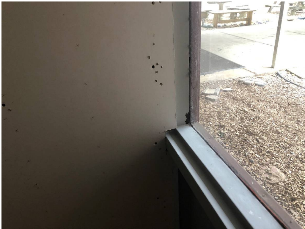
Figure 6 – Drywall Bead Need at Gypsum End
