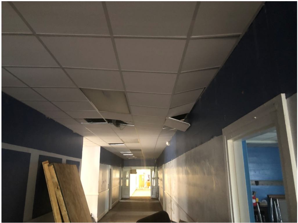
Figure 3 – New Damage at new Ceiling Noted in Main Hall
