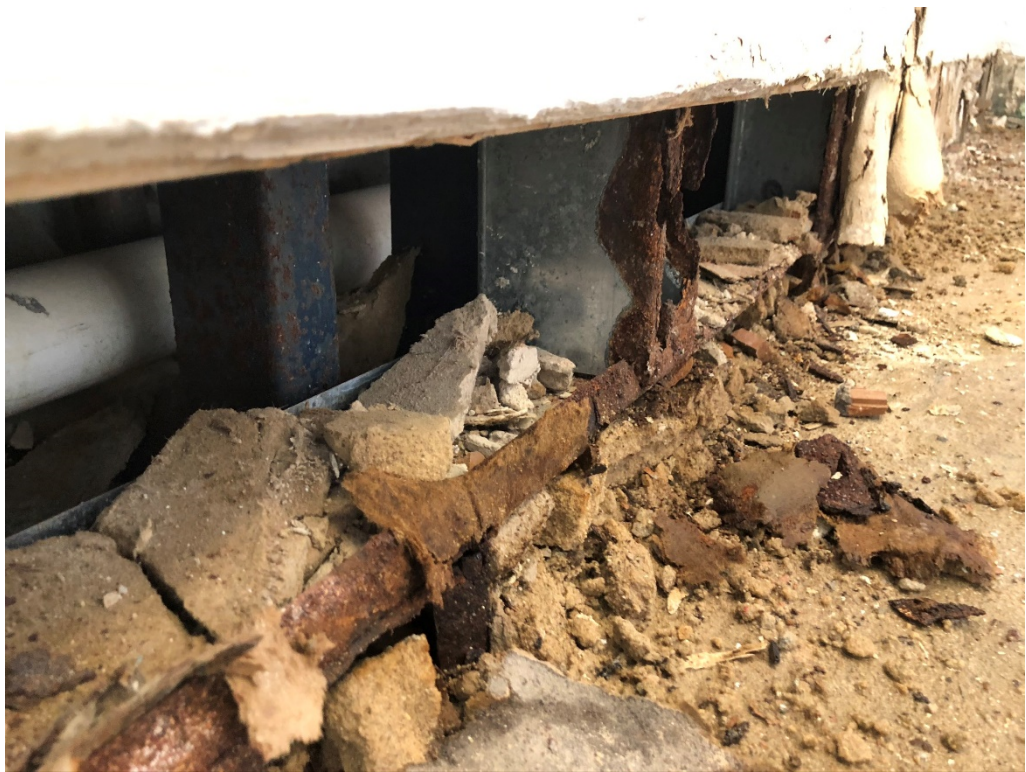
Figure 4 – Some Surface Rust Noted; Contractor should Patch as Needed to Secure Substrate
