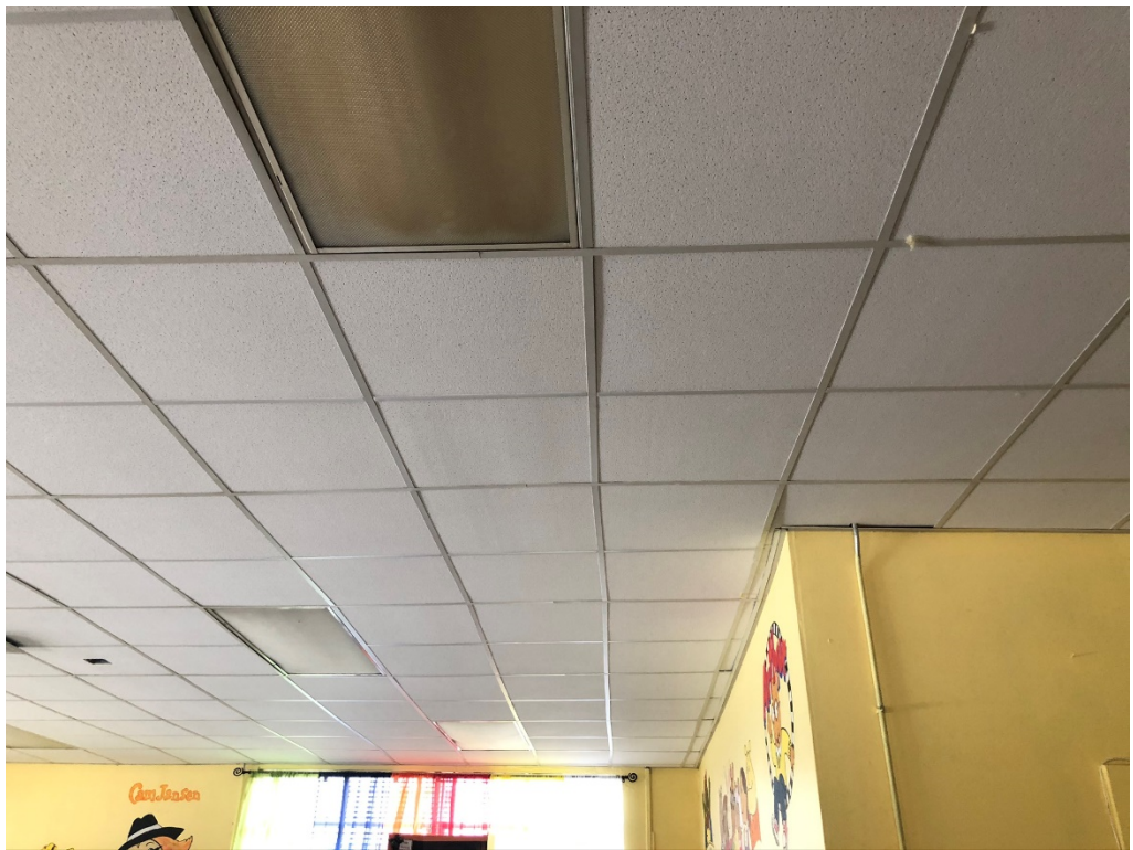
Figure 8 – Some Adjusting Required at the end of this Row at Ceiling Grid
