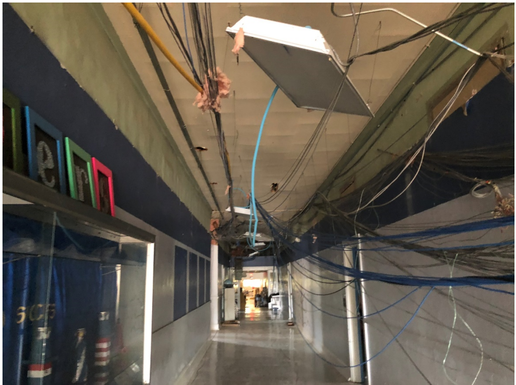
Figure 4 – Ceiling Demo Progress (Can these comm wires be temporarily supported to protect from damage?)
