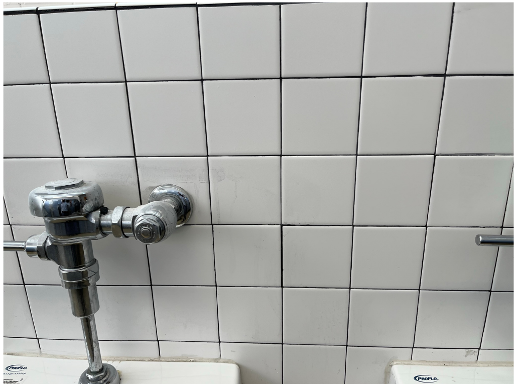
Figure 1 – Poorly done tile work
