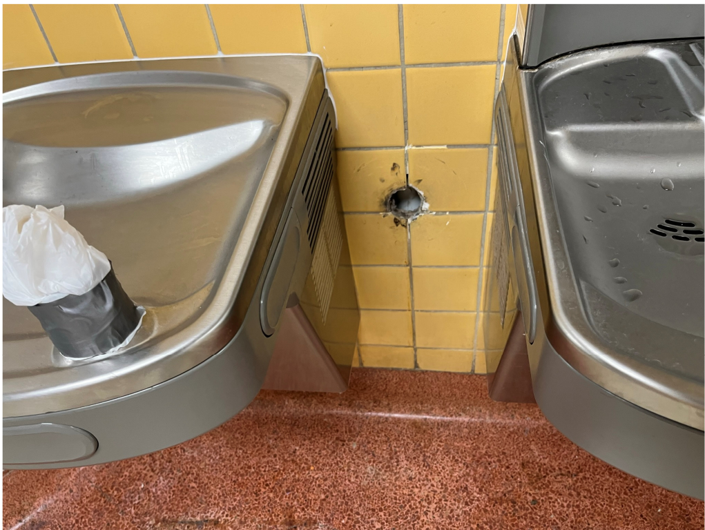
Figure 5 – Exposed Holes between water fountains
