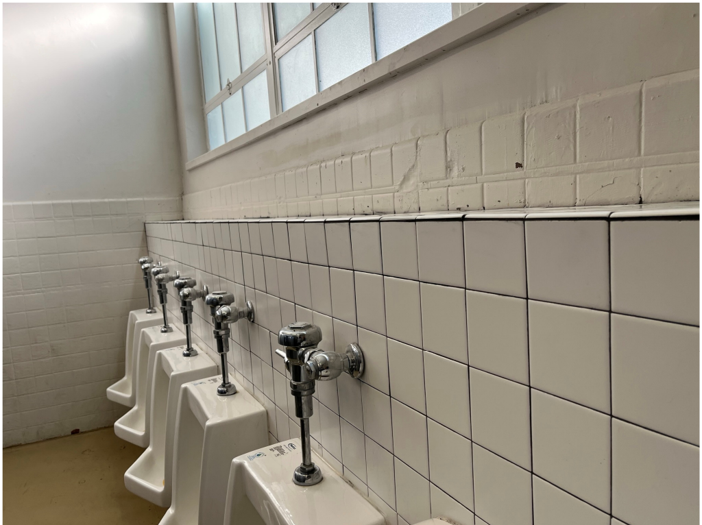
Figure 3 – Poorly done tile work
