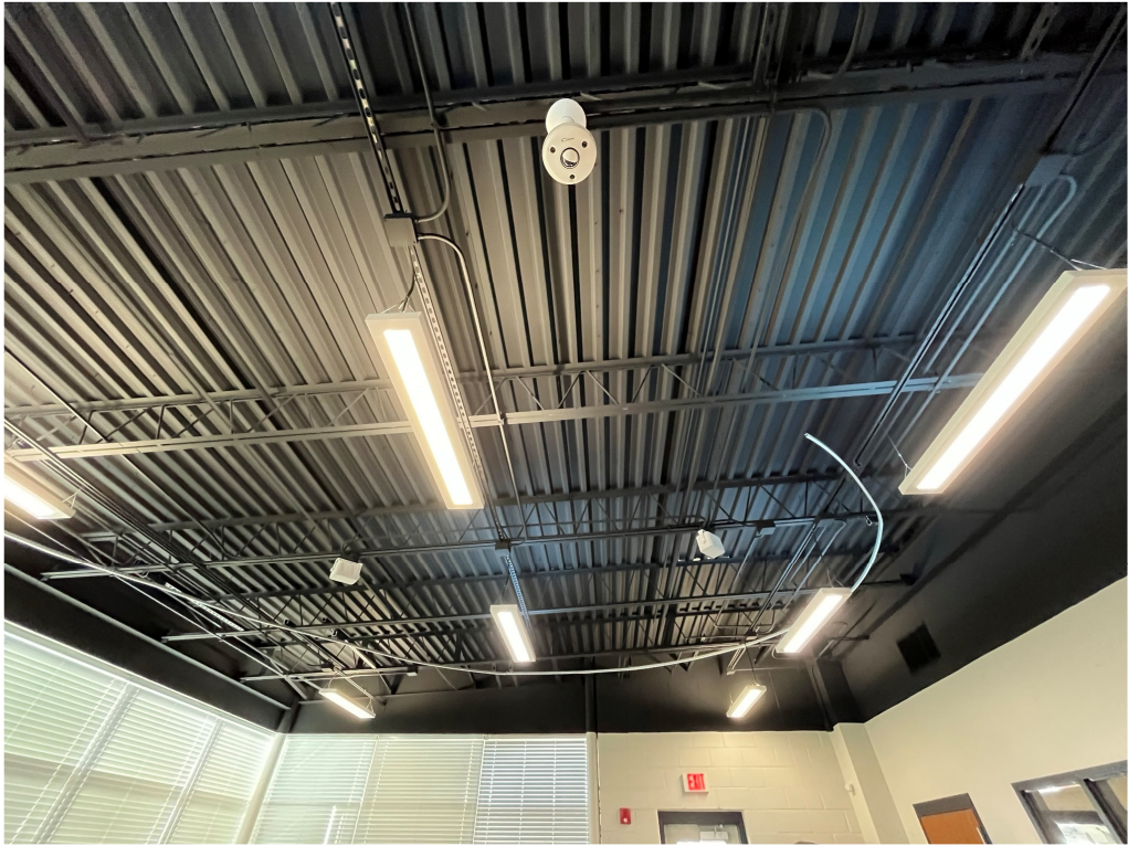
Figure 7 – This end creates a funny shape that does not conform to design
