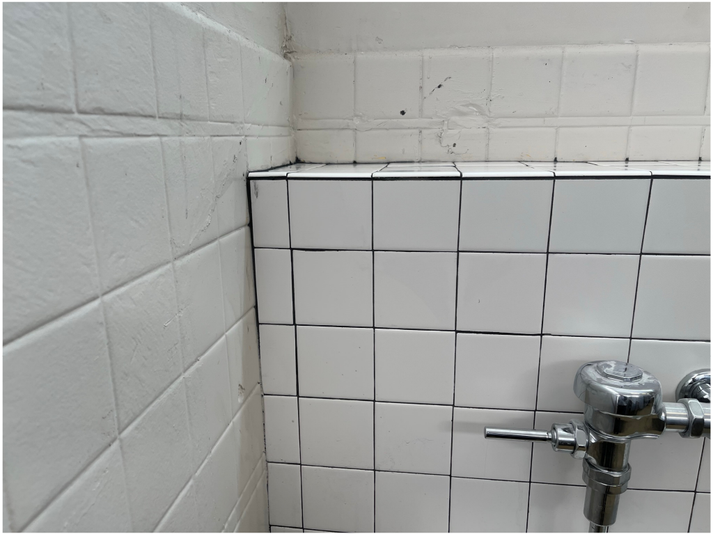
Figure 2 – Poorly done tile work
