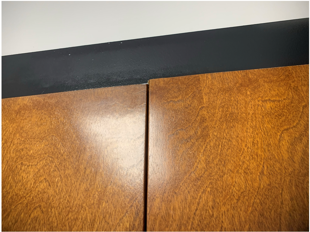
Figure 17 – Doors Require Adjustment; Also stationary leaf requires flush bolt
