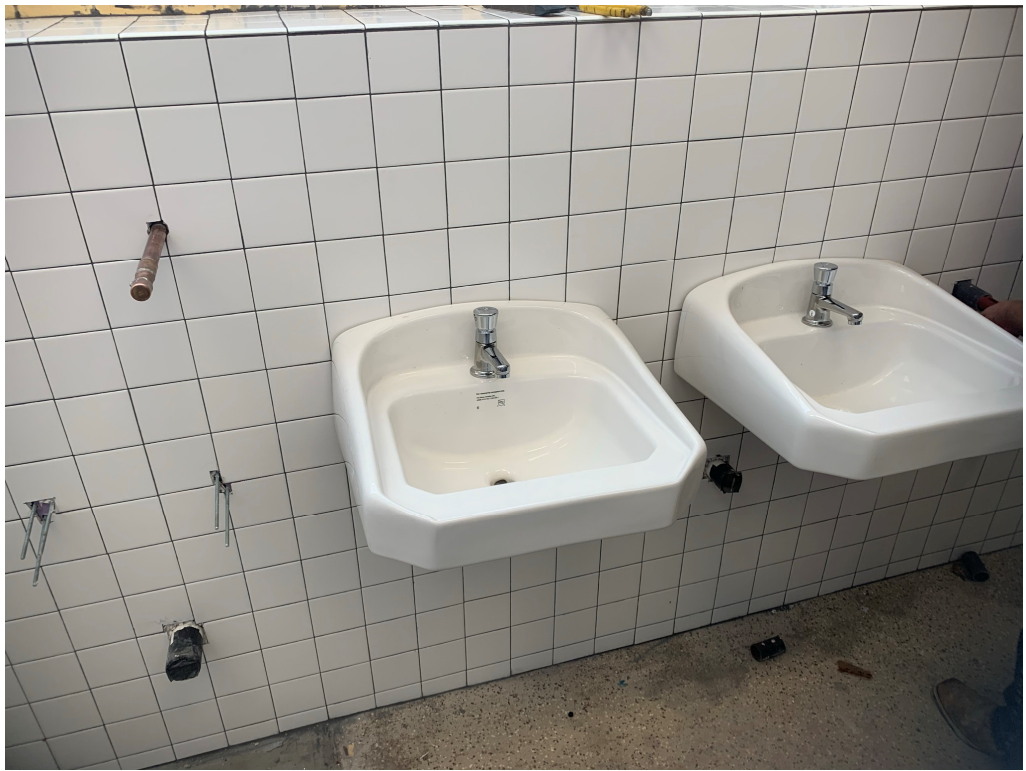
Figure 11 – Sink on left in Boys is Crooked and Requires Adjustment
