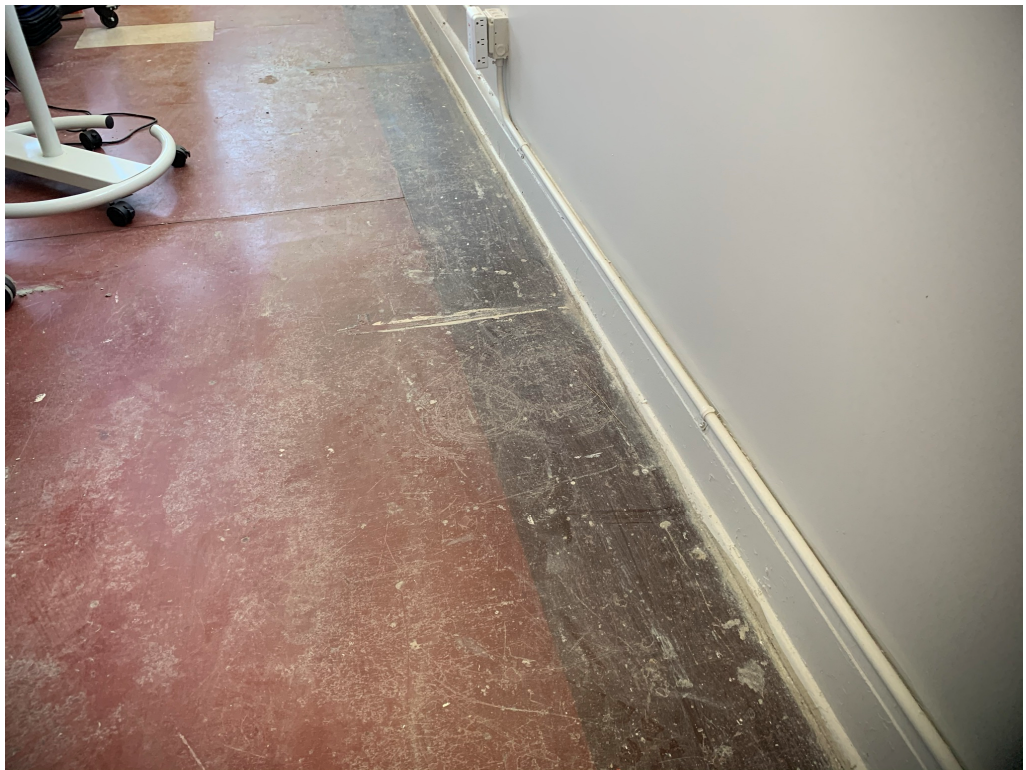
Figure 8 – Existing Floor Condition @ 2 nd Floor
