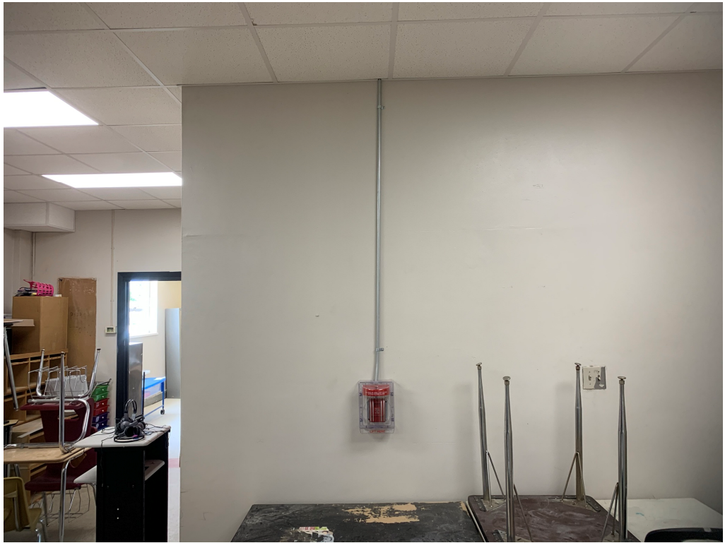
Figure 3 – This Conduit needs to be Straightened
