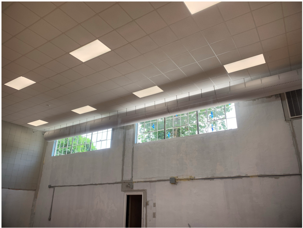
Figure 5 – Sock Duct installed at Playroom
