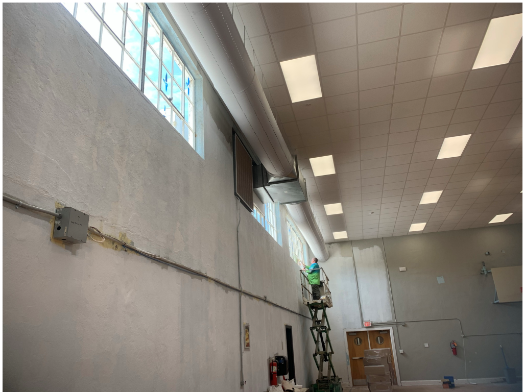
Figure 4 – Sock Duct installed at Playroom
