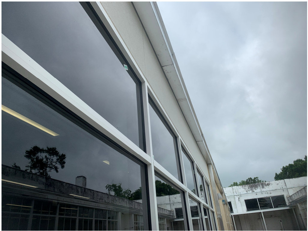
Figure 23 – Stucco to aluminum joint is flush here but offset on east side
