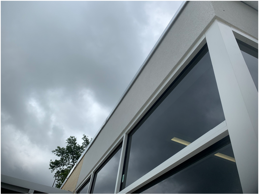
Figure 21 – Stucco to aluminum joint is offset and looks good
