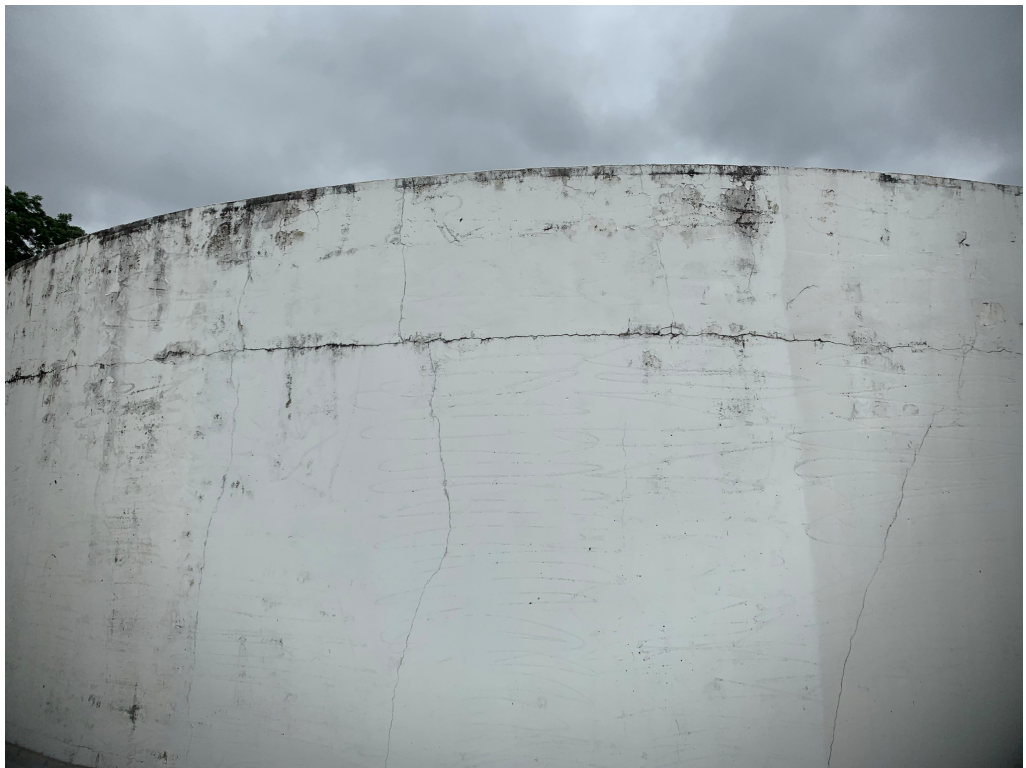
Figure 18 – Existing Wall damage (good potential for water leakage)
