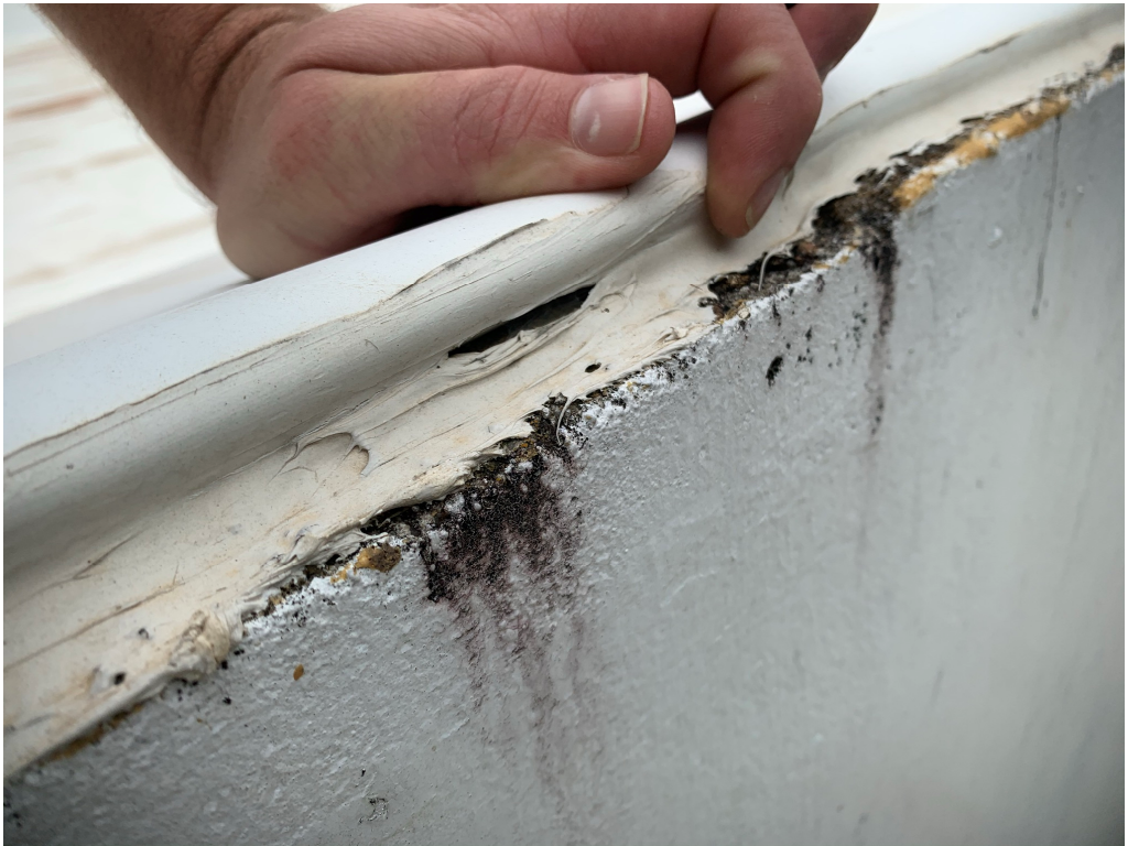
Figure 6 – Mastic does not fully cover connection at Parapet
