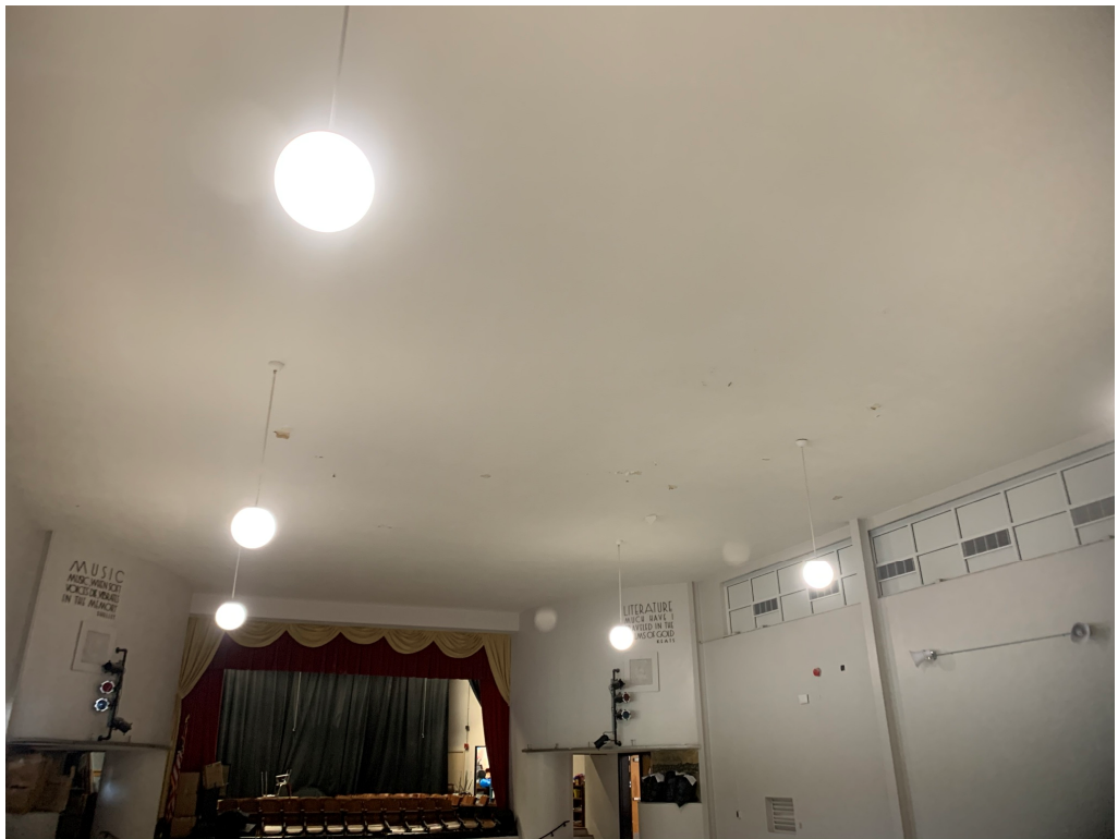
Figure 2 – Moisture up to 22%, per contractor's reading, causing paint to peel
