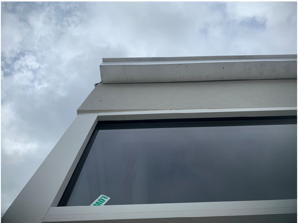
Figure 22 – Stucco to aluminum joint dives from offset to flush
