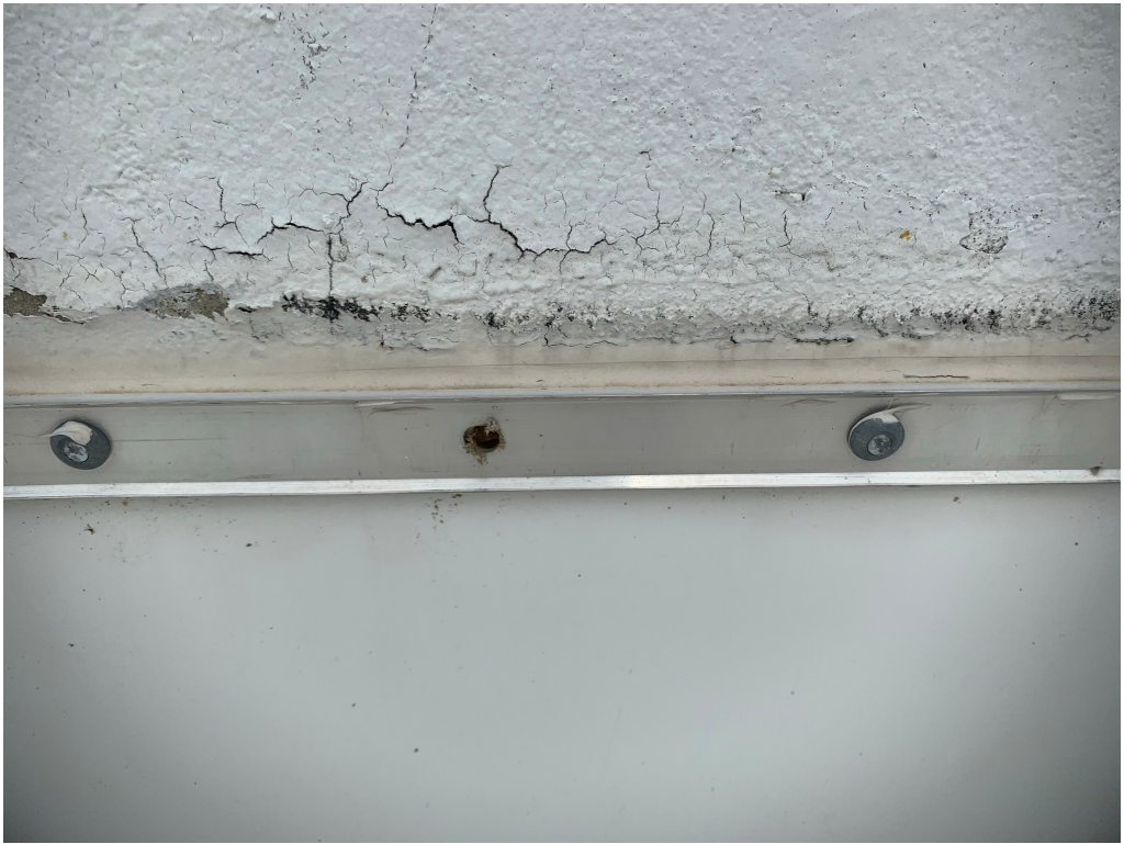
Figure 13 – Screw Missing at termination bar could be water issue
