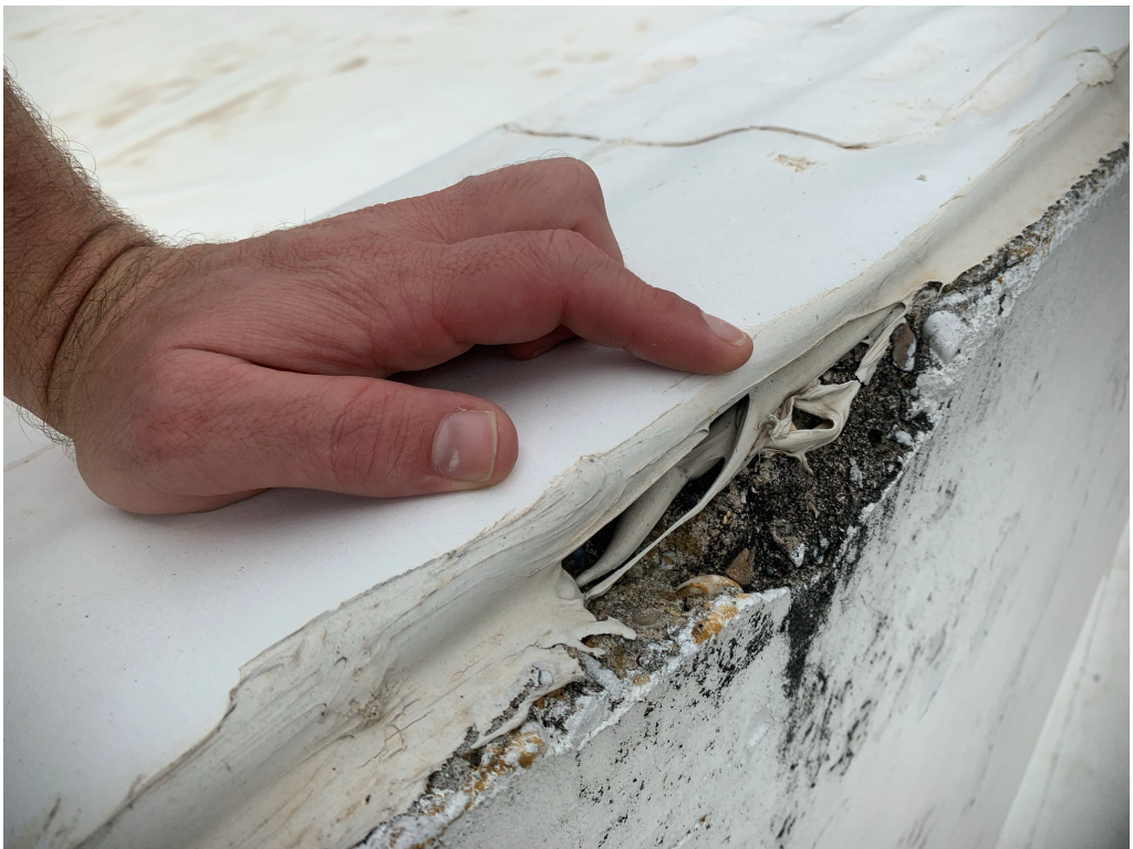
Figure 10 – Mastic does not fully cover connection at Parapet
