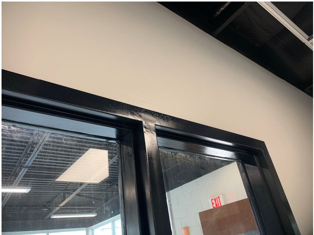
Figure 24 – Paint Drips need to be sanded out for smooth finish
