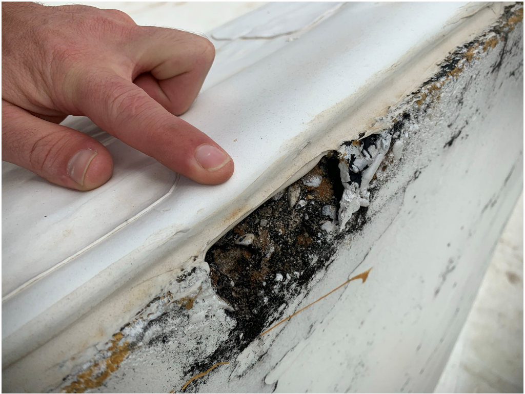
Figure 15 – Mastic does not fully cover connection at Parapet
