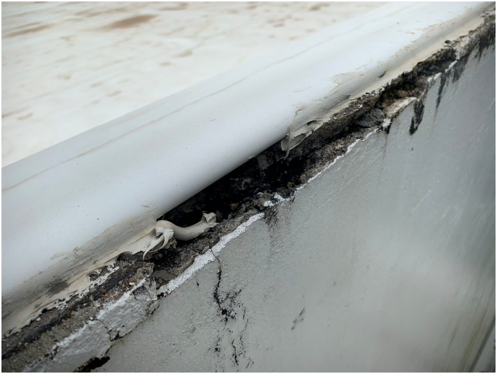
Figure 11 – Mastic does not fully cover connection at Parapet
