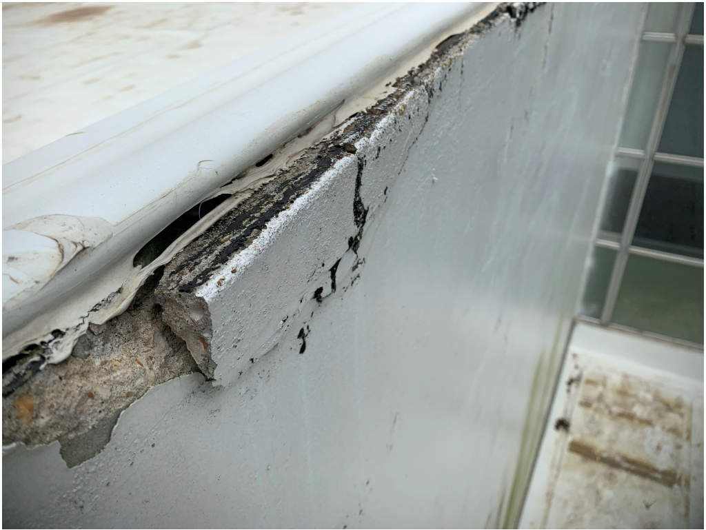
Figure 9 – Mastic does not fully cover connection at Parapet
