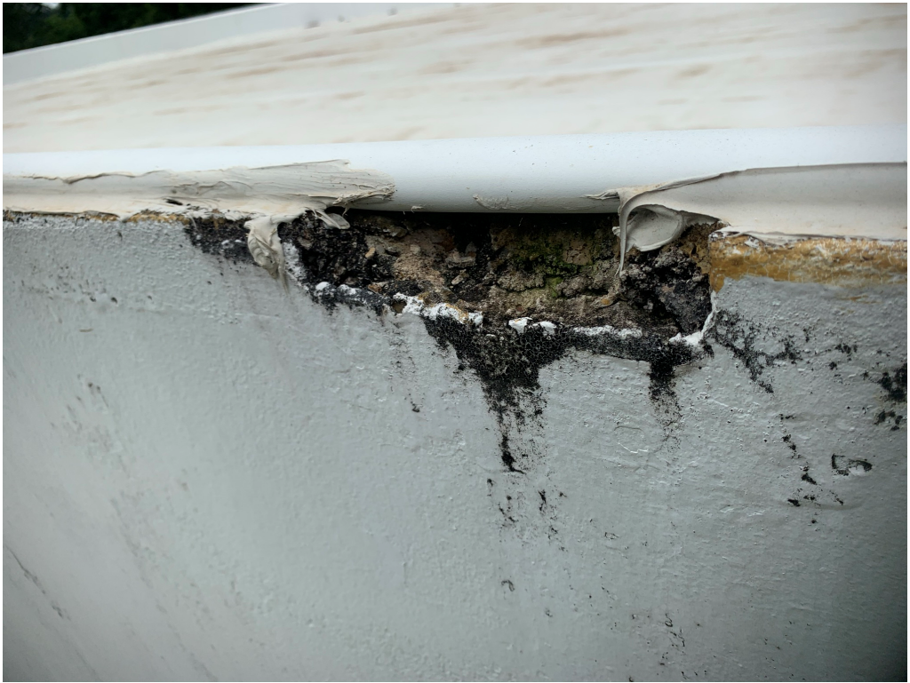
Figure 5 – Mastic does not fully cover connection at Parapet
