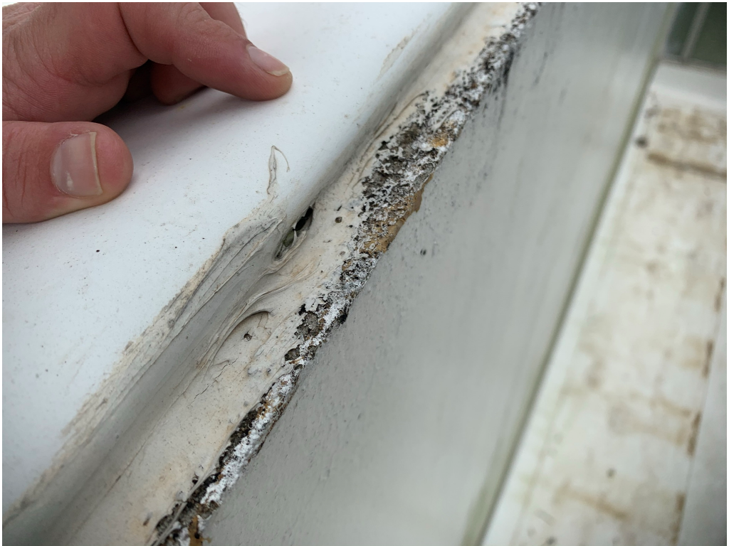
Figure 8 – Mastic does not fully cover connection at Parapet
