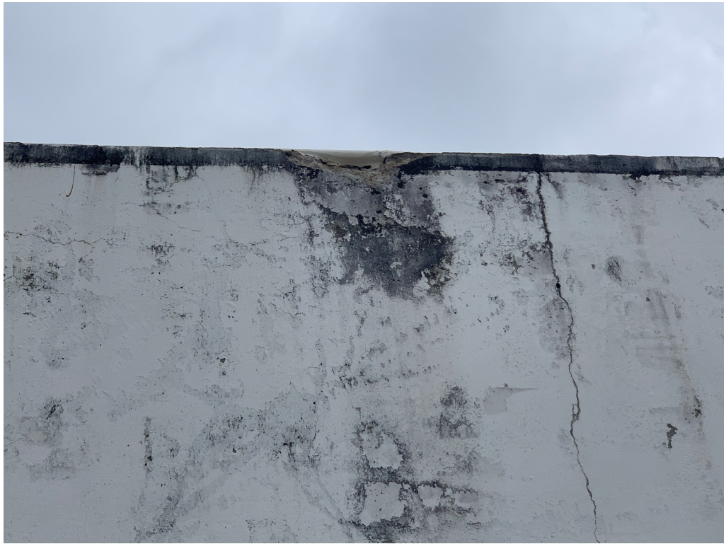
Figure 17 – Existing Wall damage (good potential for water leakage)
