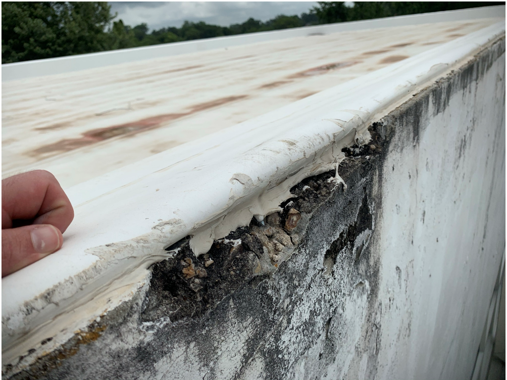
Figure 14 – Mastic does not fully cover connection at Parapet
