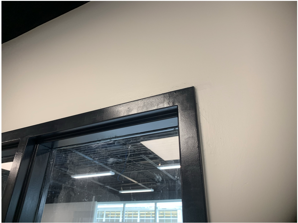
Figure 25 – Paint Drips need to be sanded out for smooth finish
