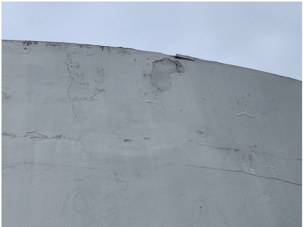
Figure 20 – Existing Wall damage (good potential for water leakage)
