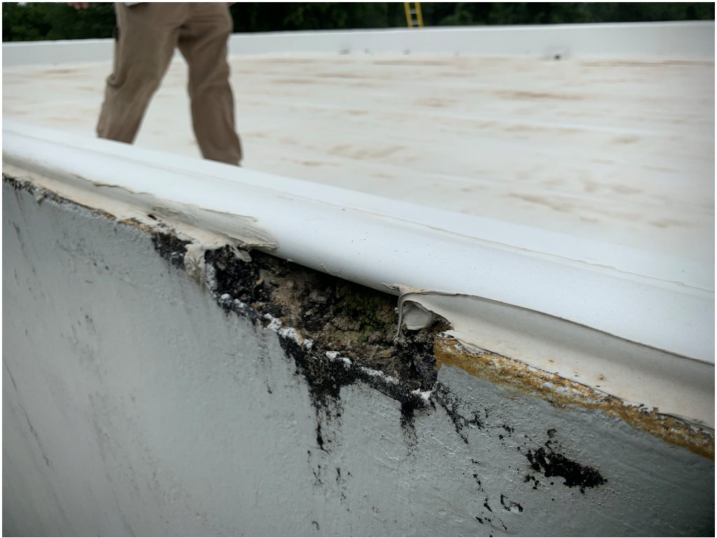
Figure 7 – Mastic does not fully cover connection at Parapet
