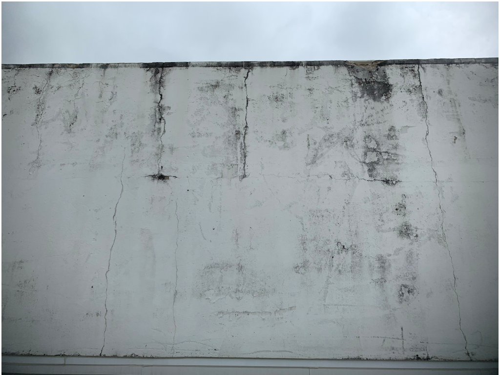
Figure 16 – Existing Wall damage (good potential for water leakage)
