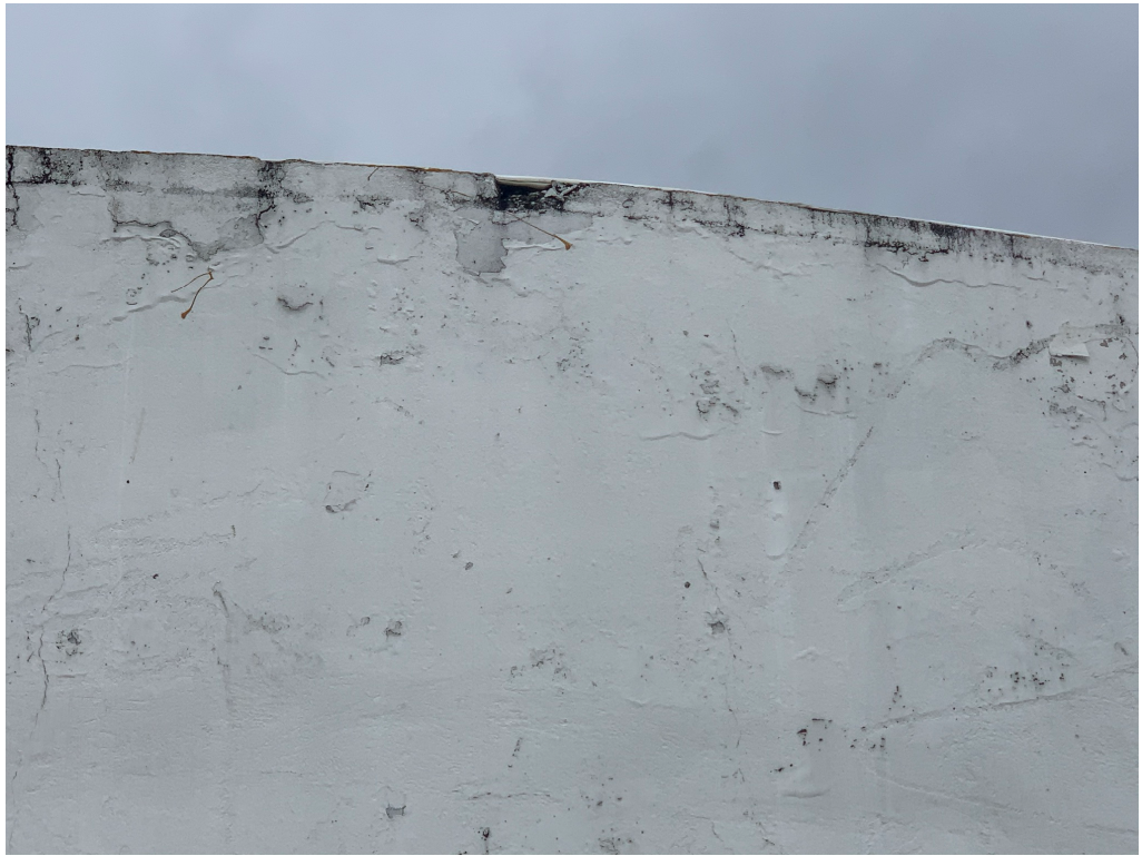
Figure 19 – Existing Wall damage (good potential for water leakage)
