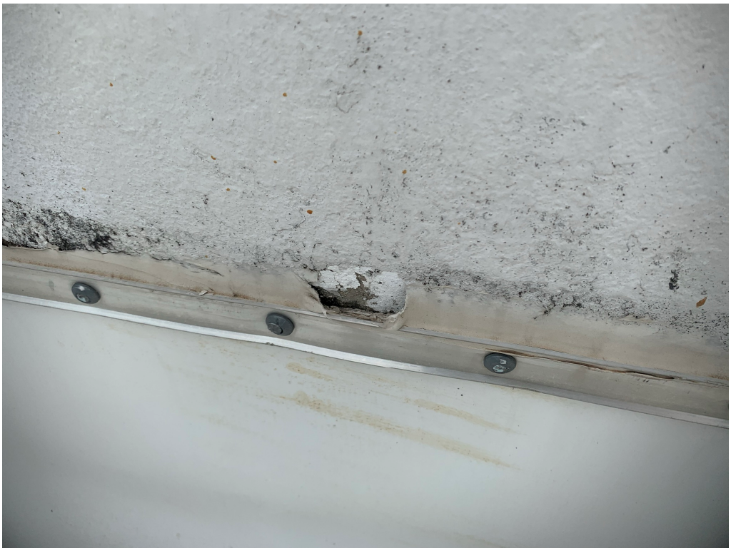
Figure 12 – Break in mastic could cause water leak
